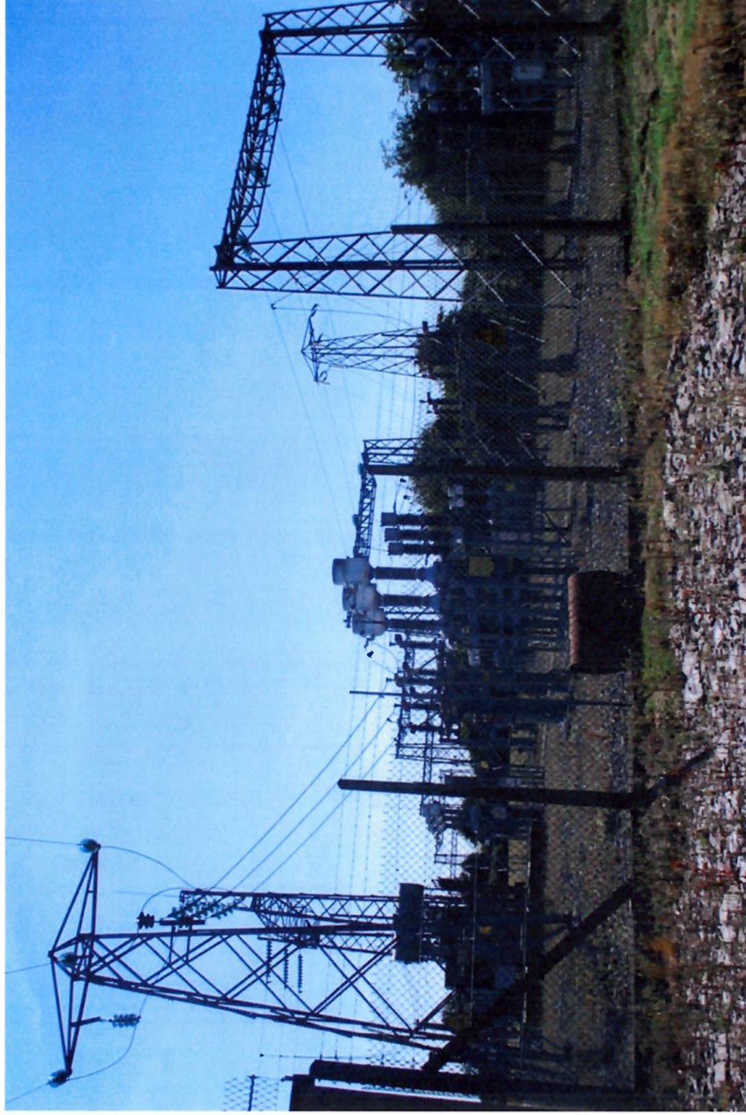
Photo 4 – Existing electrical transmission infrastructure on the site
