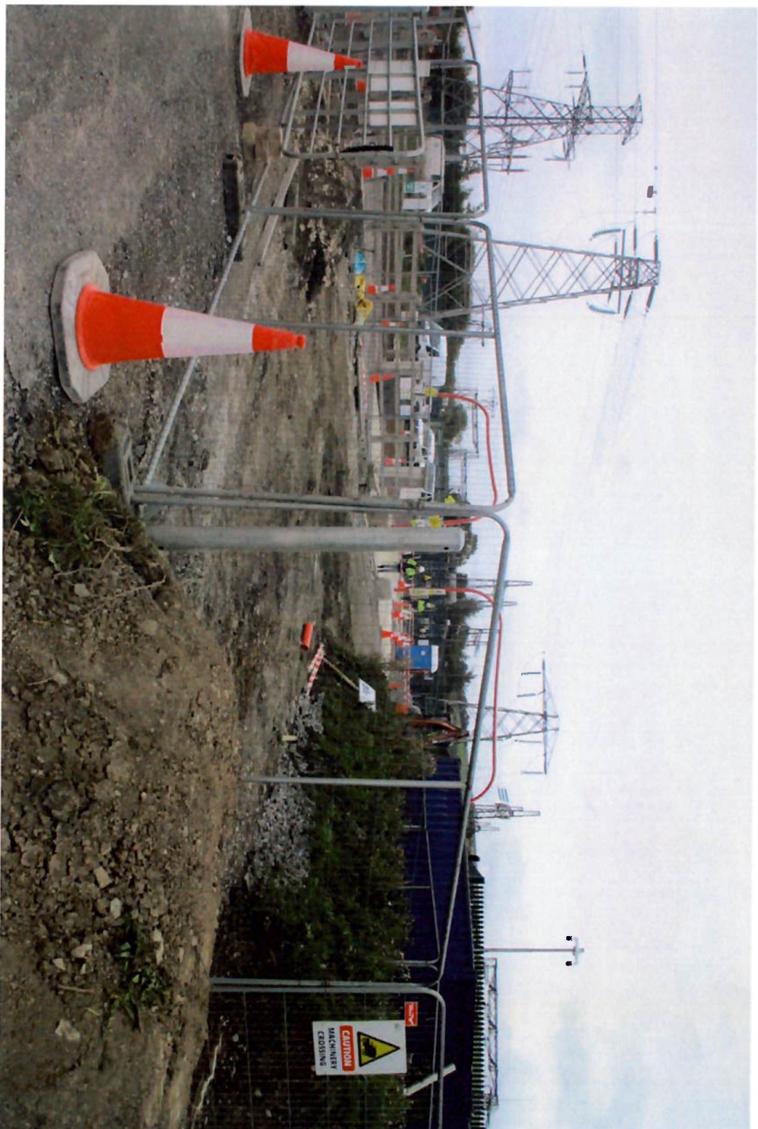
Photo 5 – Existing Trian 110kV substation immediately to the east of the subject site
