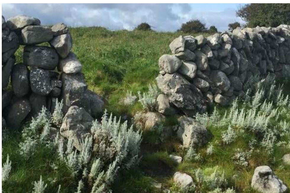
Figure 9: Collapsed stone wall that needs to be rebuilt.
