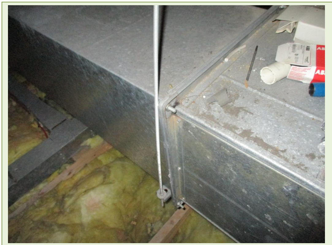
Seals between ducting. No ACM's detected
