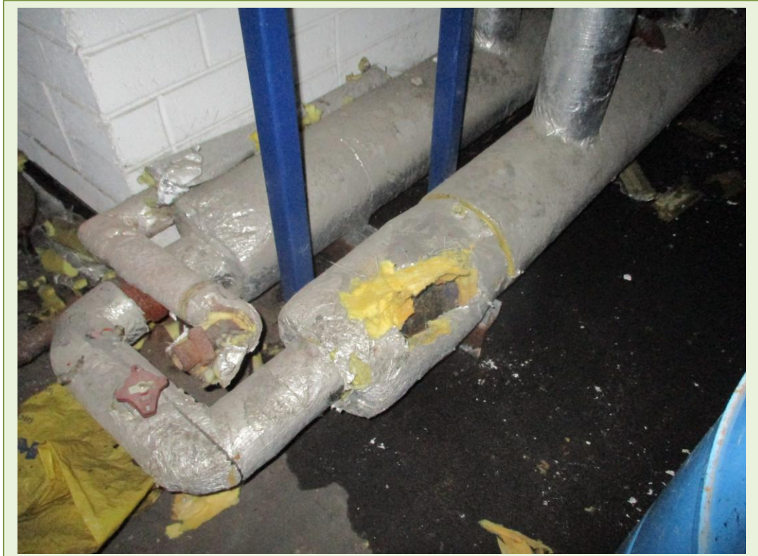
Fiberglass insulation in plant room. No ACM's detected
