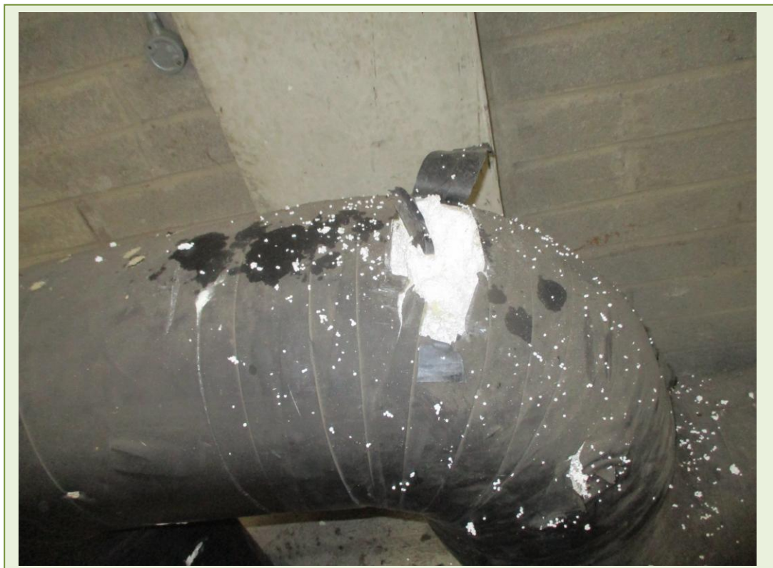
Polystyrene insulation on cold lines. No ACM's detected
