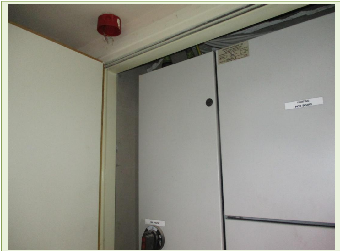
Board around electrical panel. No ACM's detected
