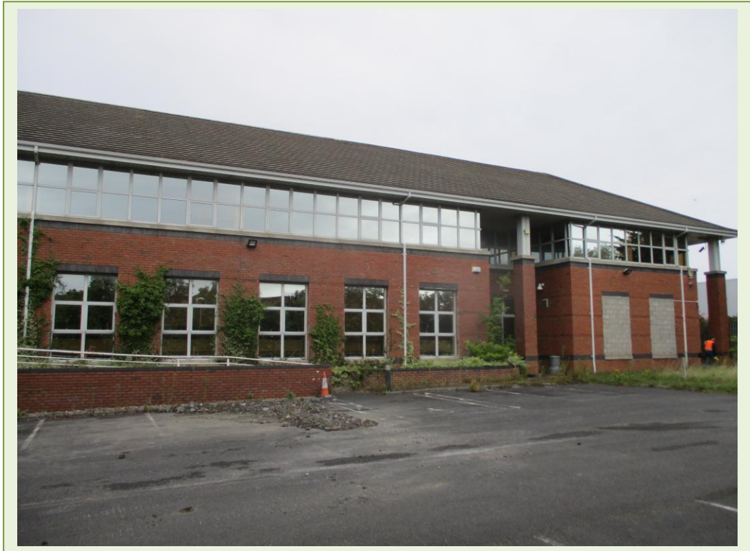
Tiles on roof of office block. No Asbestos Containing Materials (ACM's) detected
