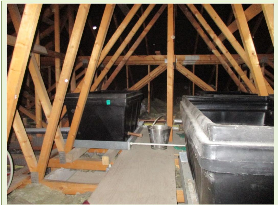
Attic insulation, roof felt and water tanks in office block. No ACM's detected
