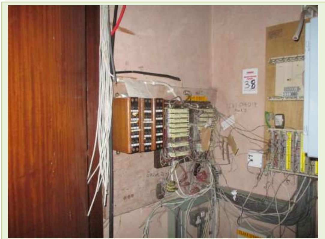
Telecoms fire stopping. No ACM's detected
