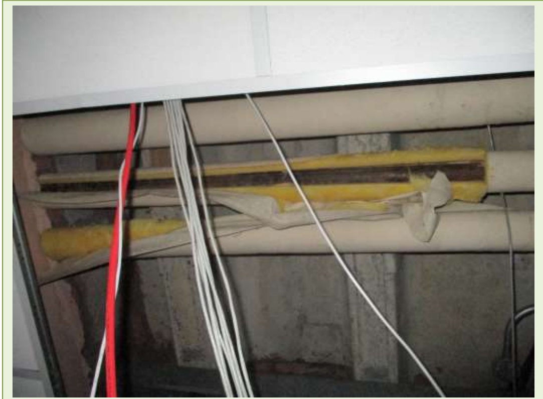
Fiberglass pipework insulation. No ACM's detected
