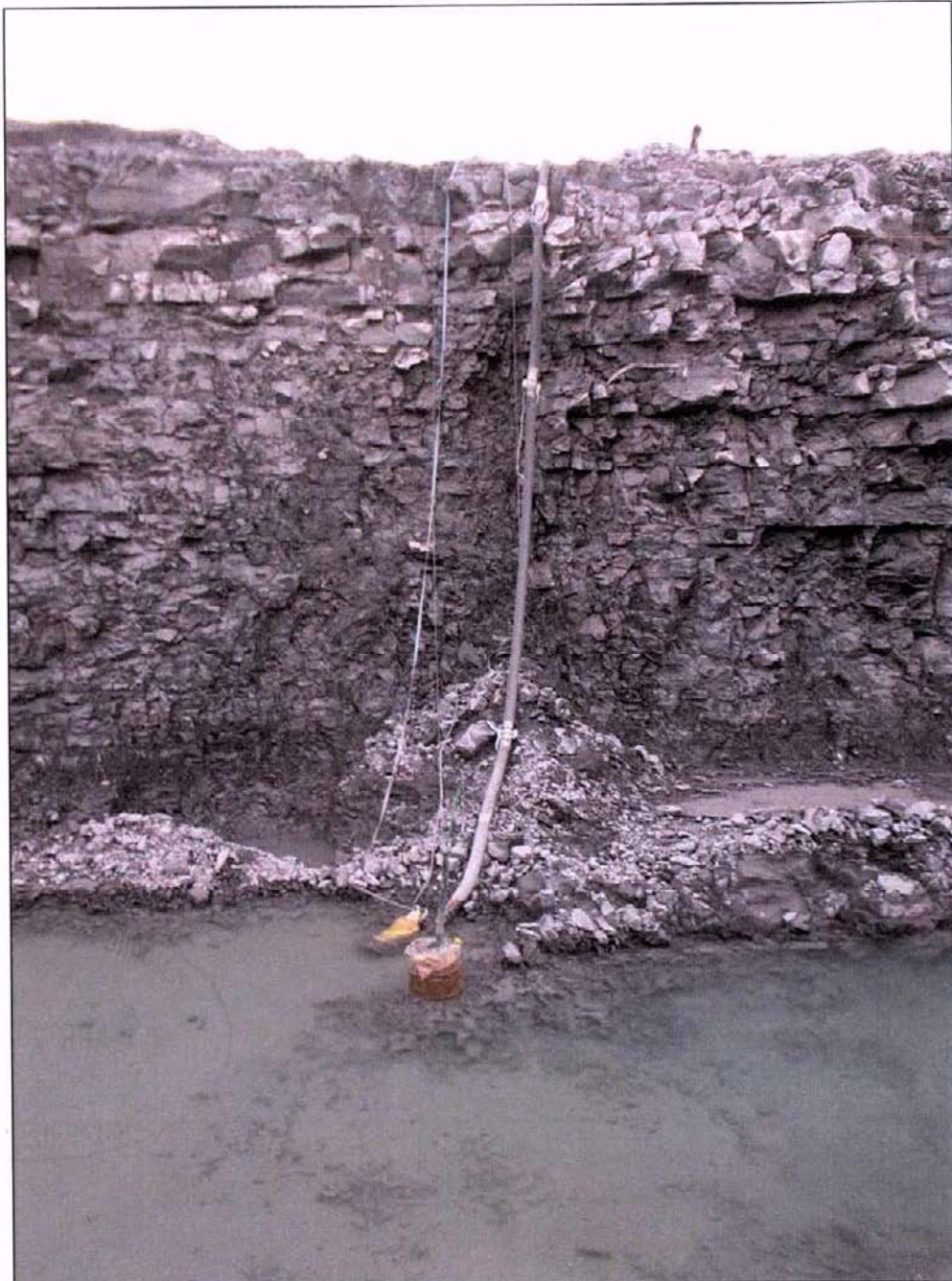
Plate 3.6 Sump and pump
