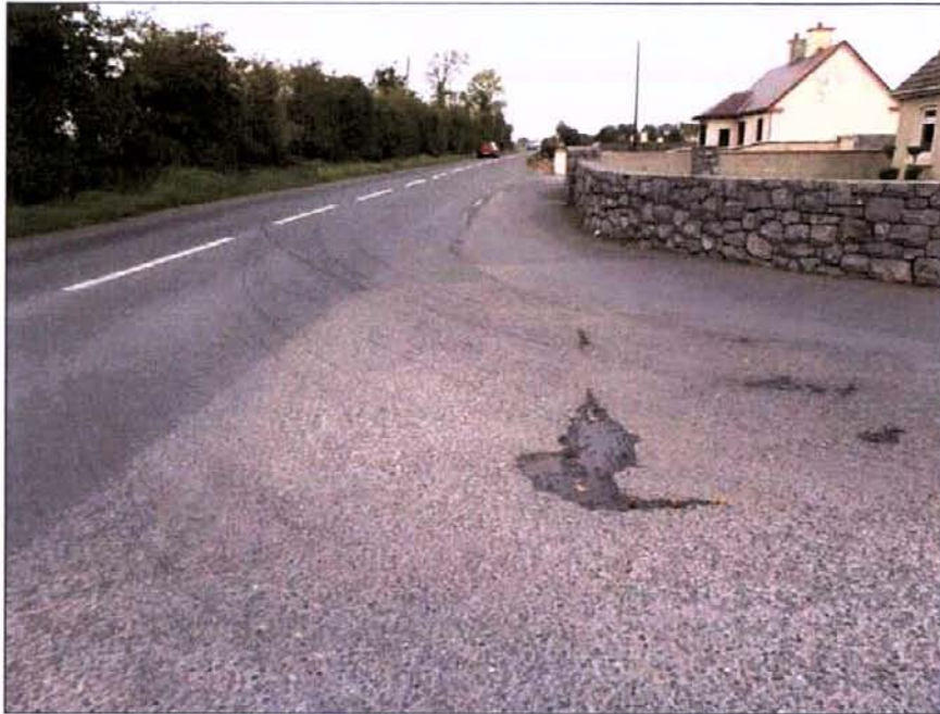
Plate 12-1 Looking east along the R339 Monivea Road taken from the junction with L7109
