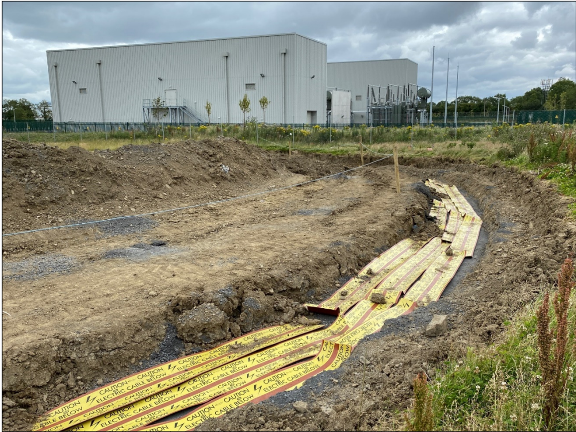
Figure 6.6 Area of spoil and bare ground (ED2) and improved agricultural grassland (GA1) to the west of the existing Castlebaggot 220/110kV substation within the grid connection route for the Proposed Development.
