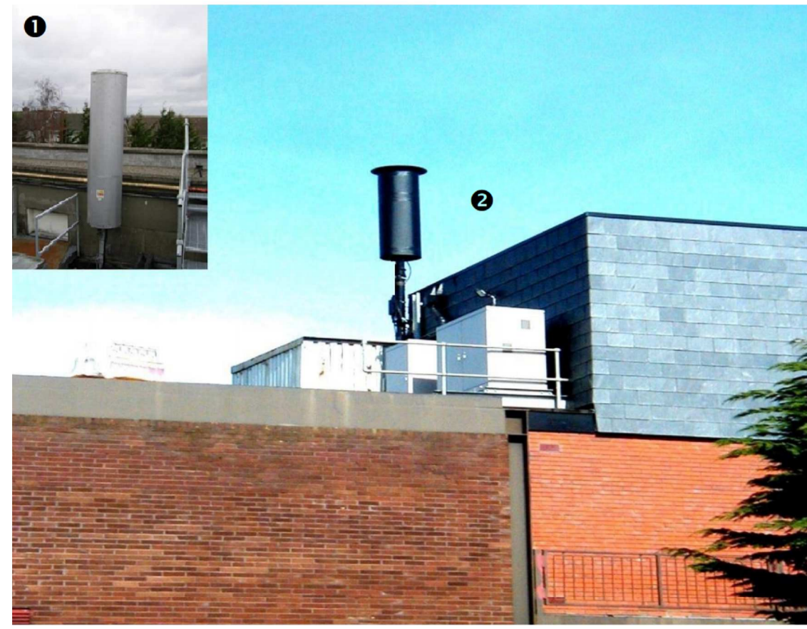
Typical Telecom Installations
