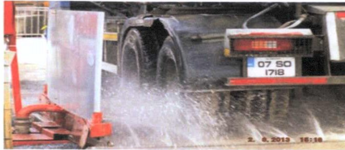
Figure 9 – Typical Wheel Washing Facility
