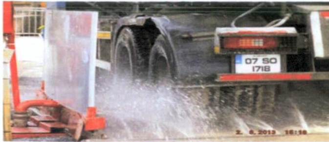
Figure 8 - Typical Wheel Washing Facility
