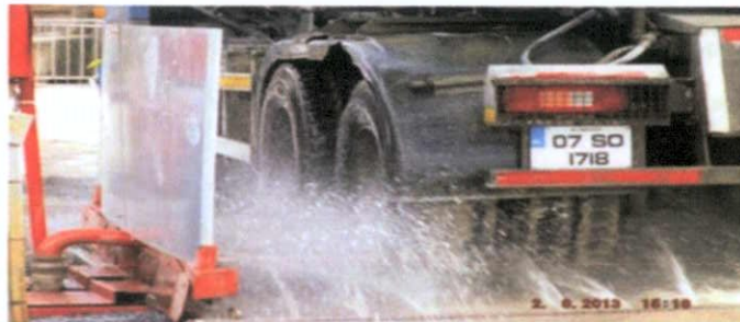
Figure 8 – Typical Wheel Washing Facility
