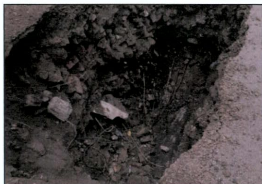
Figure 57 The floor abutting the wall foundation
