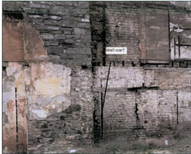
Figure 81 Wall scar of Building 2
