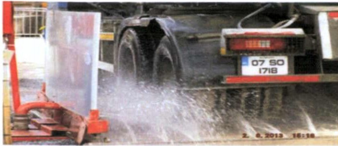
Figure 8 - Typical Wheel Washing Facility
