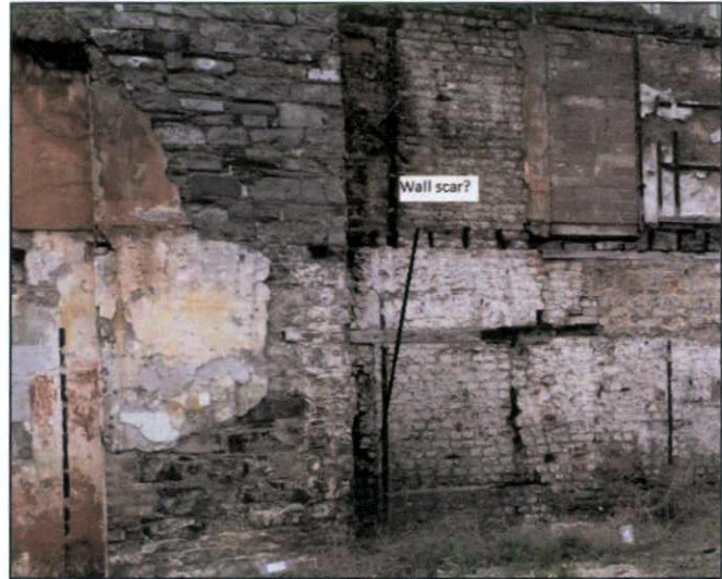
Figure 81 Wall scar of Building 2
