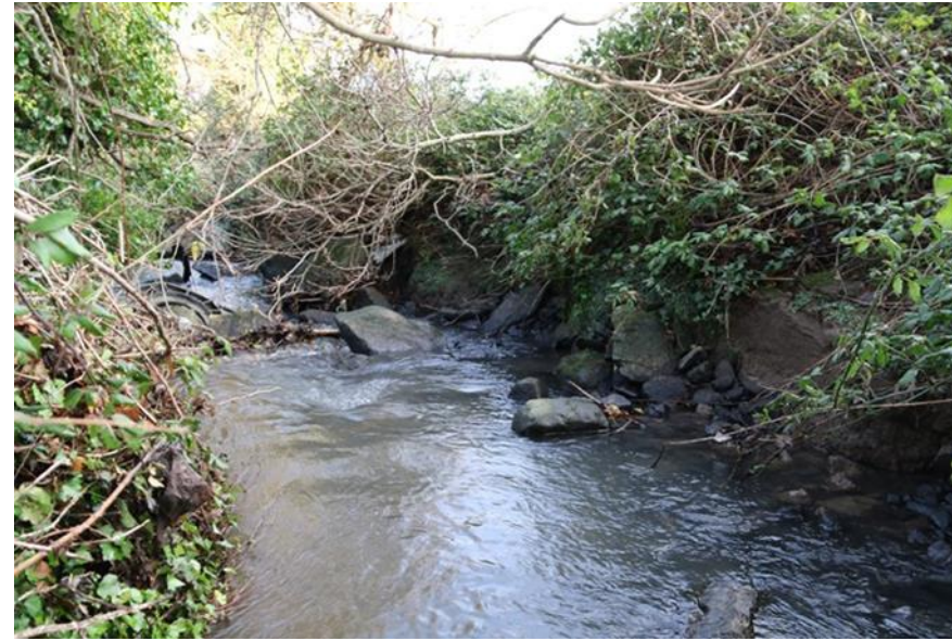
Photo 5: Collapsed stone in river channel
