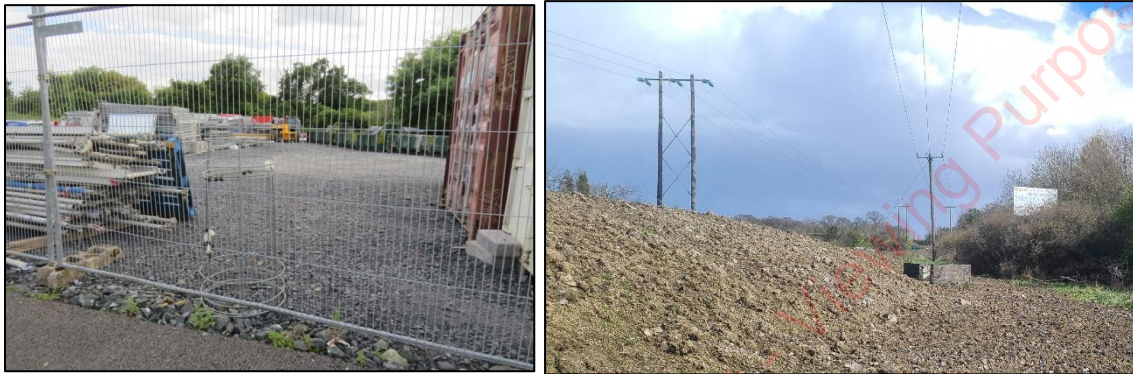
Plate 2: Left - Spoil and bare ground habitat within the campus. Right – haul road undergoing construction in the north lands.
