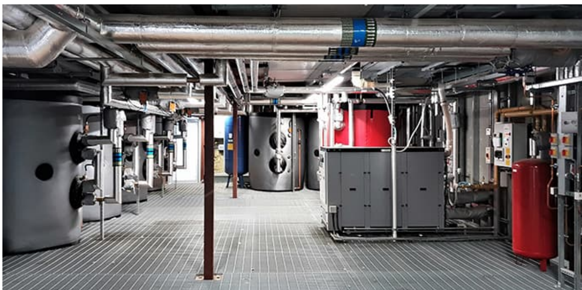
Figure 7: Example Centralised Plantroom
