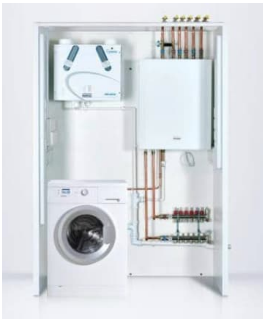
Figure 2: HIU for Centralised Heating System
