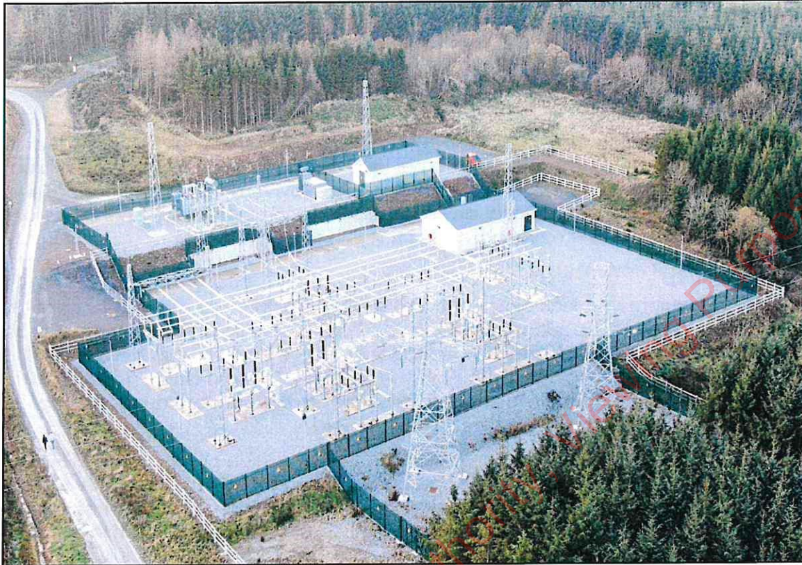
Figure 3.3: Example of a 110kV AIS Substation with split-level design
