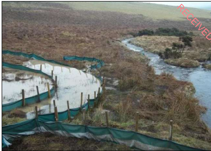
Plate 1: Photograph of Silt Fencing
