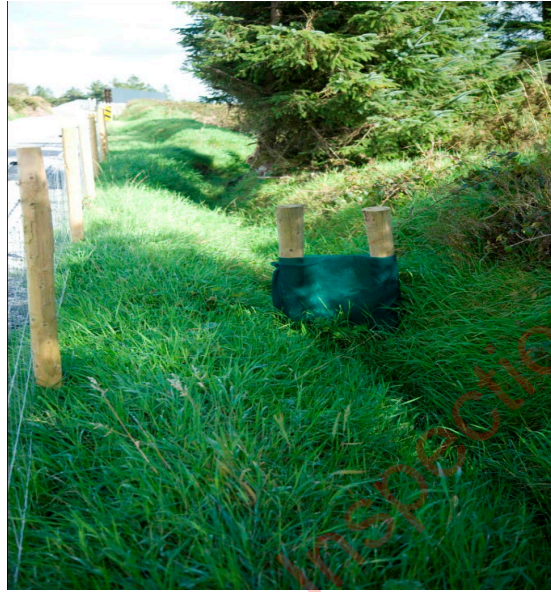
Figure 3-5: Silt trap across grassed swale
