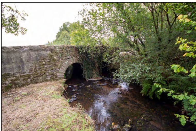
Plate 13 Bridge Site 4 had some suitable crevices and bat potential. However, no bats or signs of bat usage were recorded during the survey.
