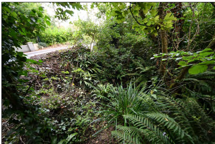
Plate 1 Bridge Site 1 was assessed as having no bat potential; it is too low for bats to use and has no suitable crevices / access.
