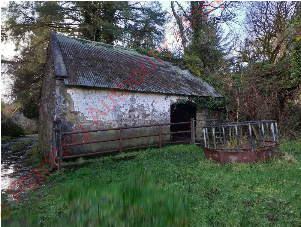
Plate 4 - Derelict cattle shed
