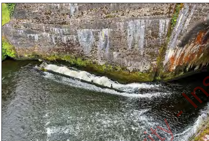
Plate 26 The fish pass at the culvert which was not working during the site visit. The boards on the fish pass were broken. This is downstream of survey Site A12.
