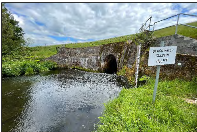
Plate 25 The River Blackwater culvert under the headrace canal. This causes an upstream migration barrier for fish. This is downstream of survey Site A12.
