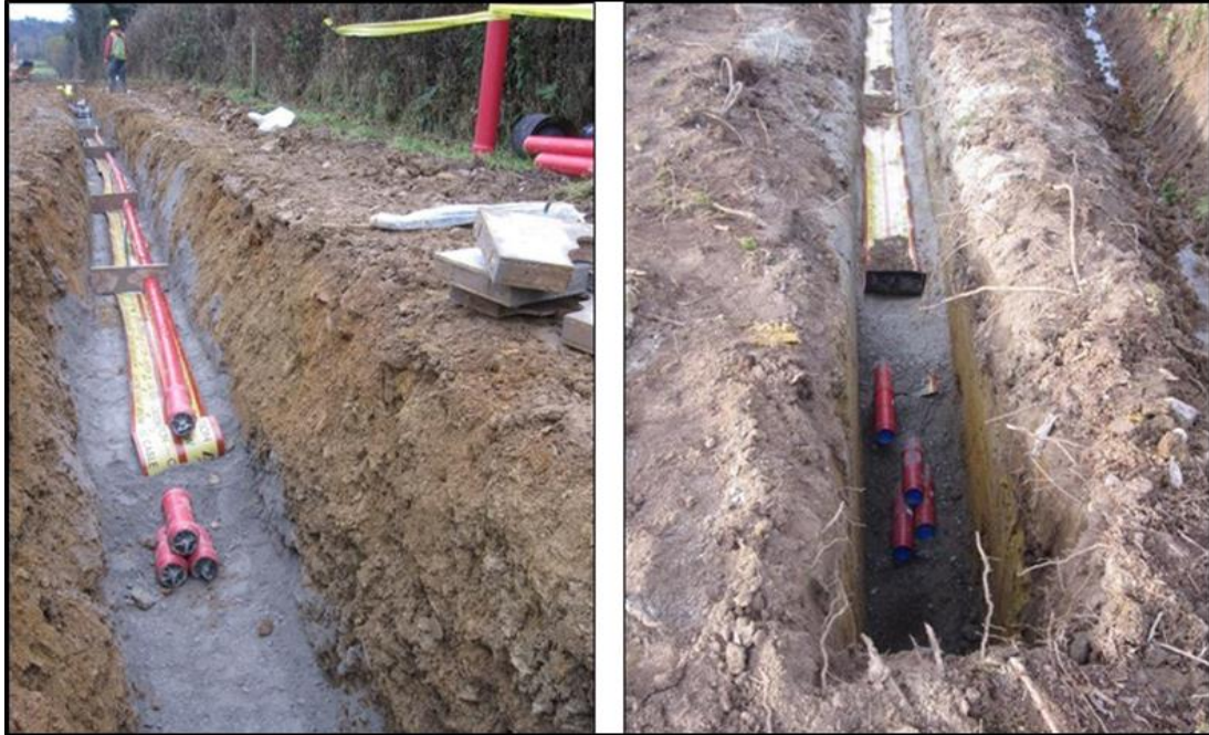
Plate 2-1 Typical Cable Trench View
