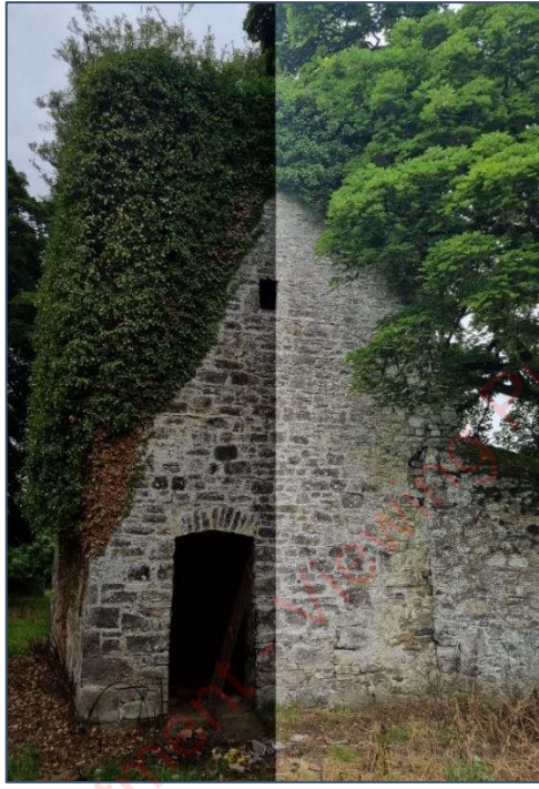
Plate 4-4 East facing wall of the castle tower with potential access through door and window
