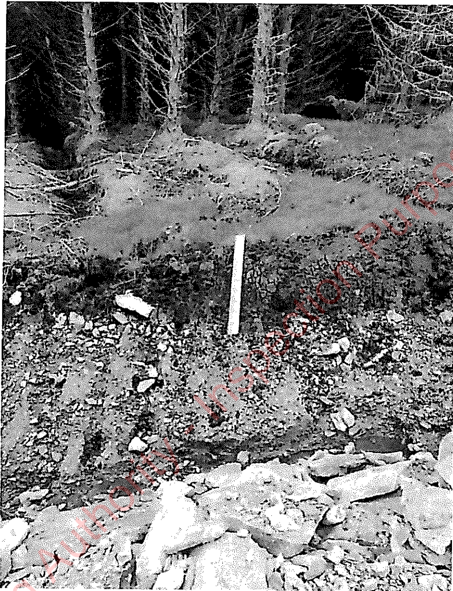
Peat and till exposed at new access track and drainage associated with ongoing forestry activities observed during site survey.
