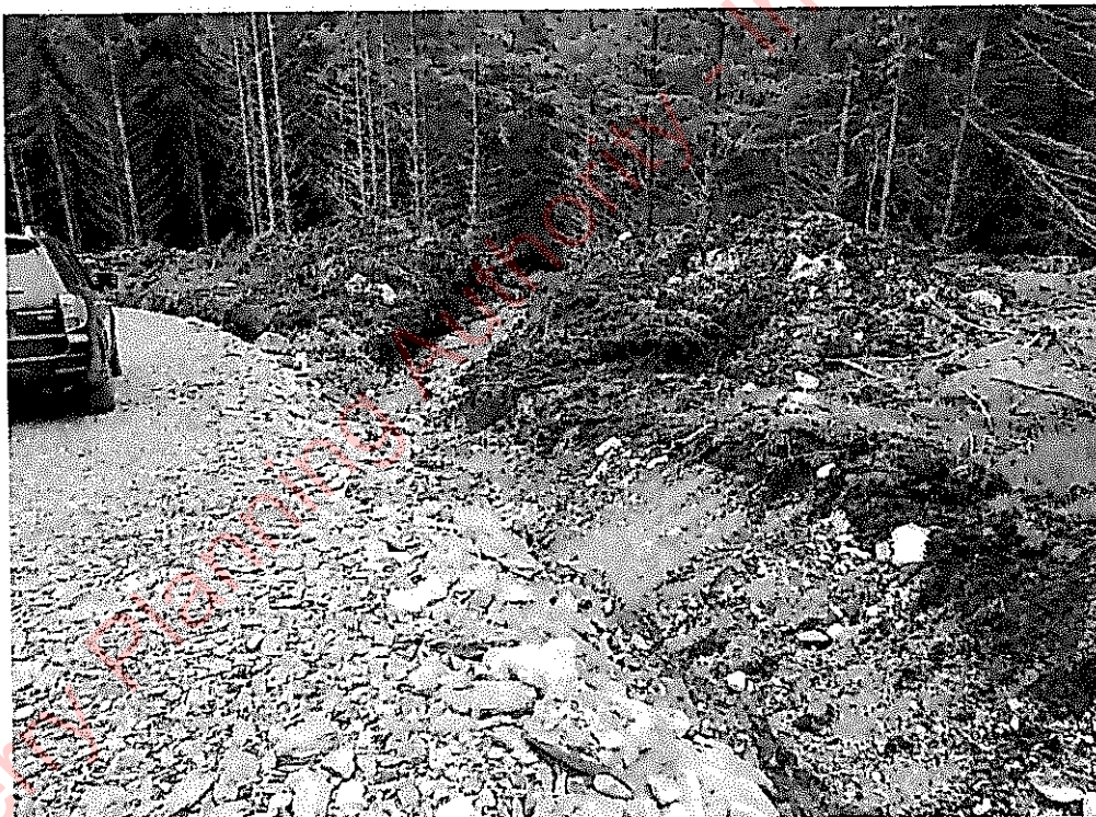
New access track and drainage associated with ongoing forestry activities observed during site surveys 16/06/2020.
