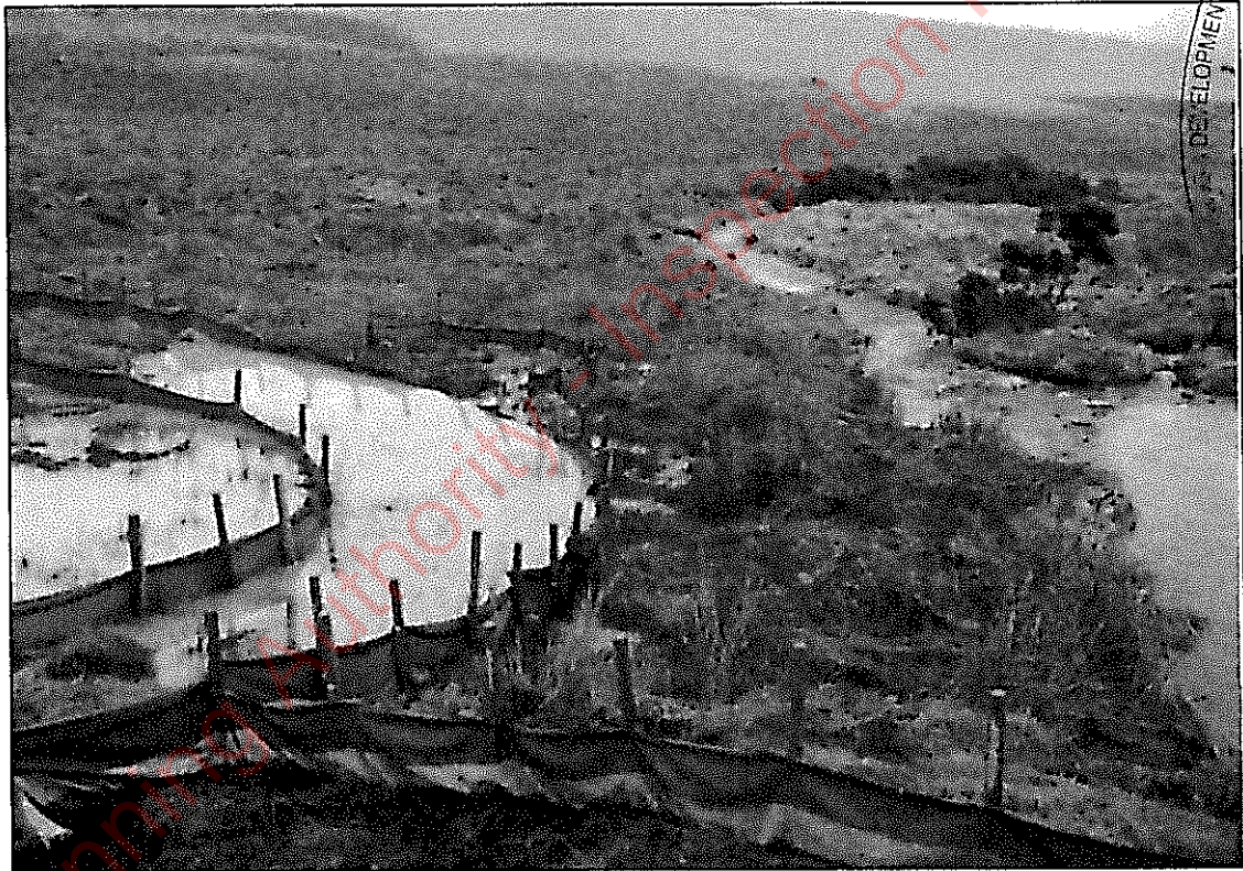
Plate 5.2: Photograph of silt fencing
