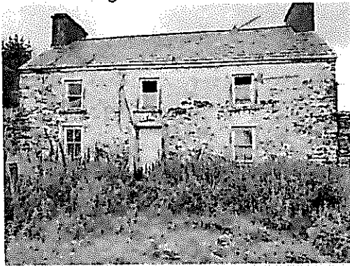
3. Derelict dwelling indicating potential access points via soffit, ridge tiles and gaps in roof tiles and open window.
