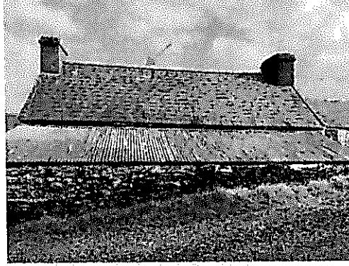
2. Rear view of dwelling indicating potential access points in raised ridge tiles and soffit
