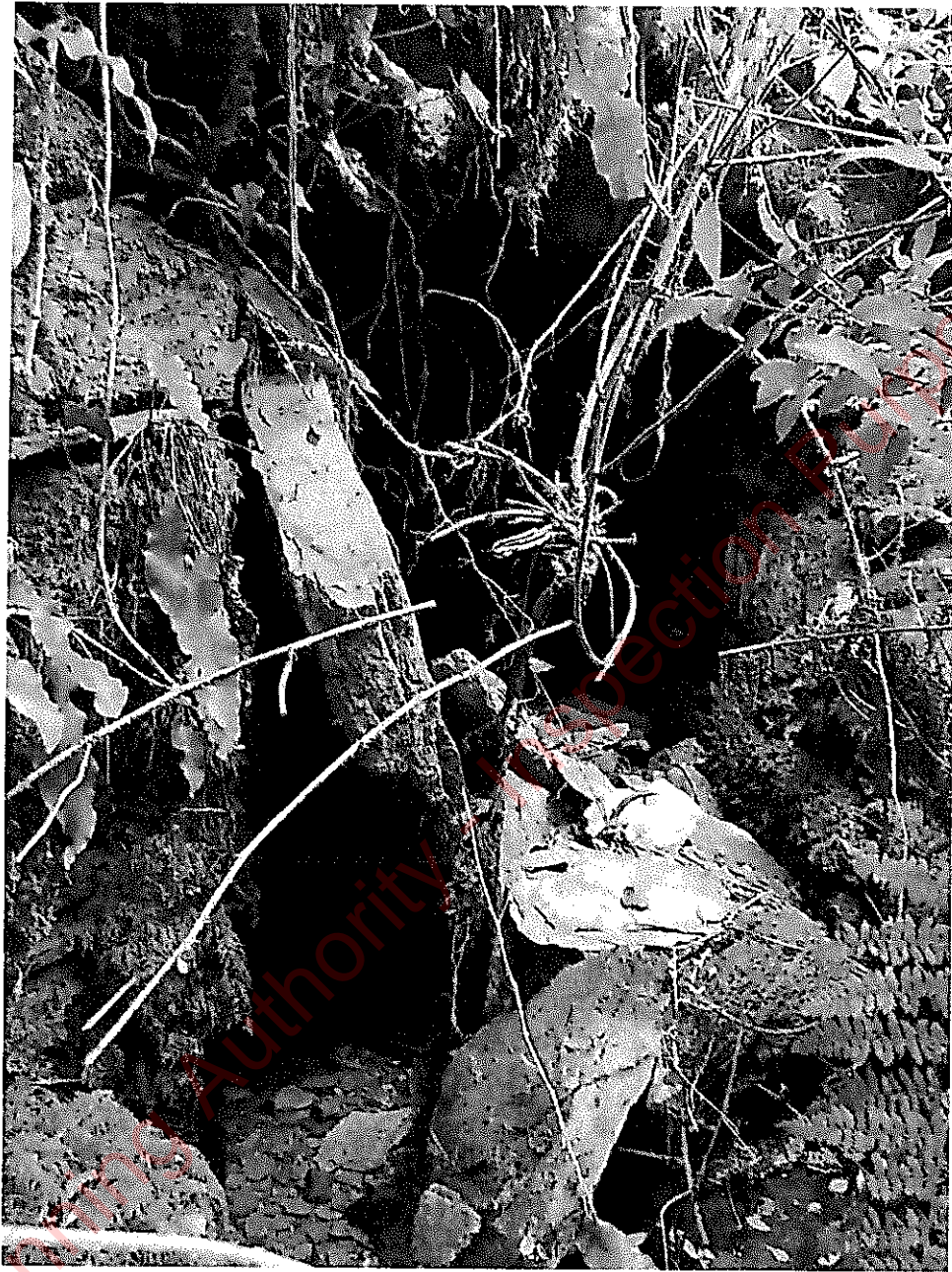
Collapsed stones at the west end of the south span
