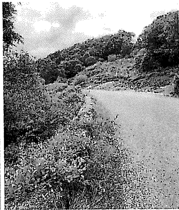
Image : 53 Stone wall to LHS of the road as there is a significant elevation change from the roads surface to the existing ground
