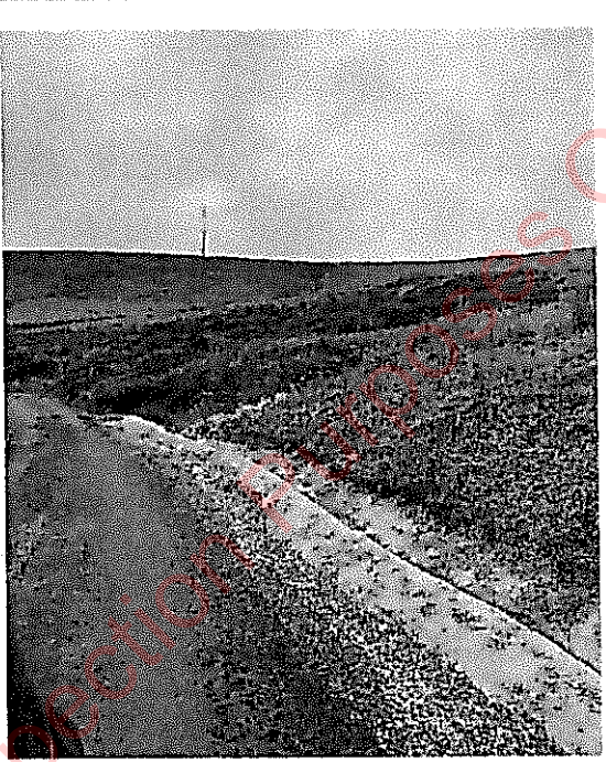
Image : 18 Joint bay on the road here with a links box and communications chambers visible.
