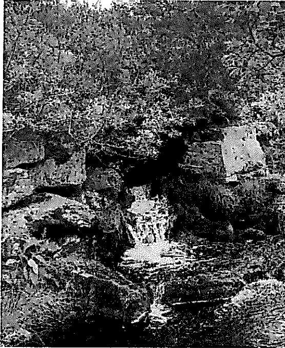
Image : 80 Stream crossing track at this location with a partial collapsed storm pipe
