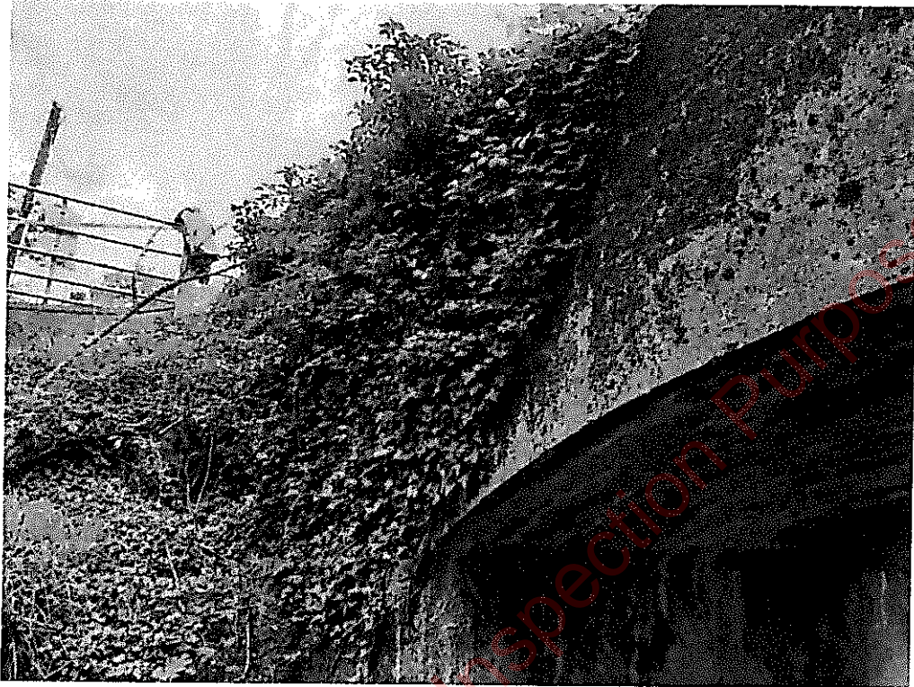
Vegetation growth on the west elevation
