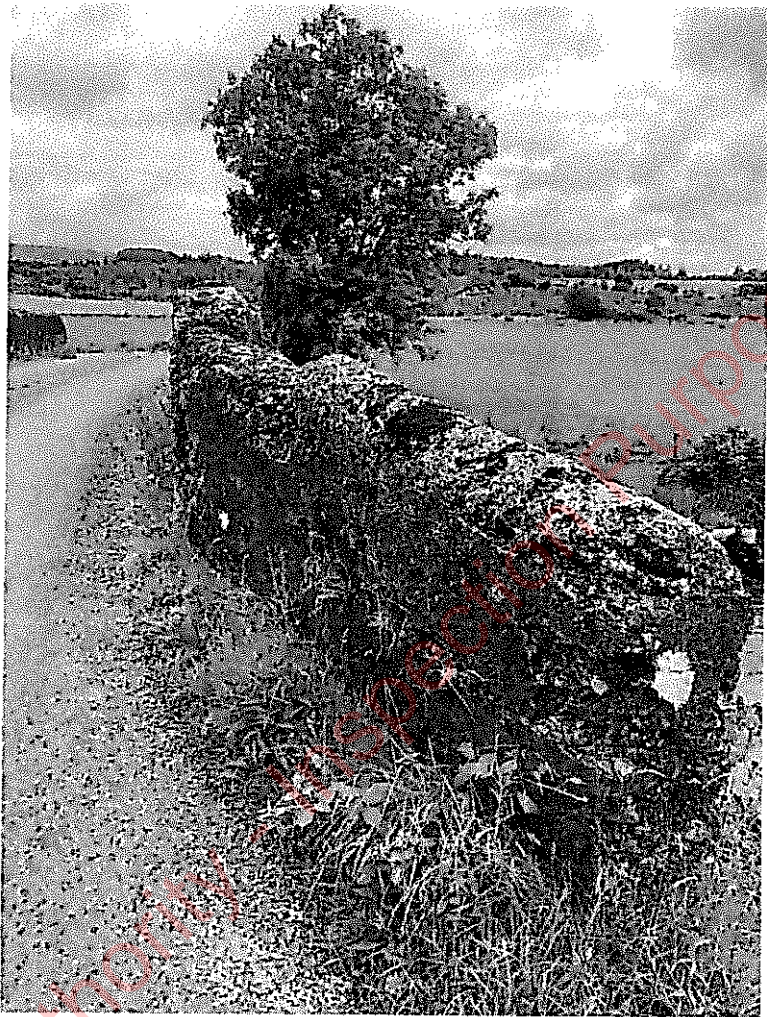
Close up of parapet showing concrete damage
