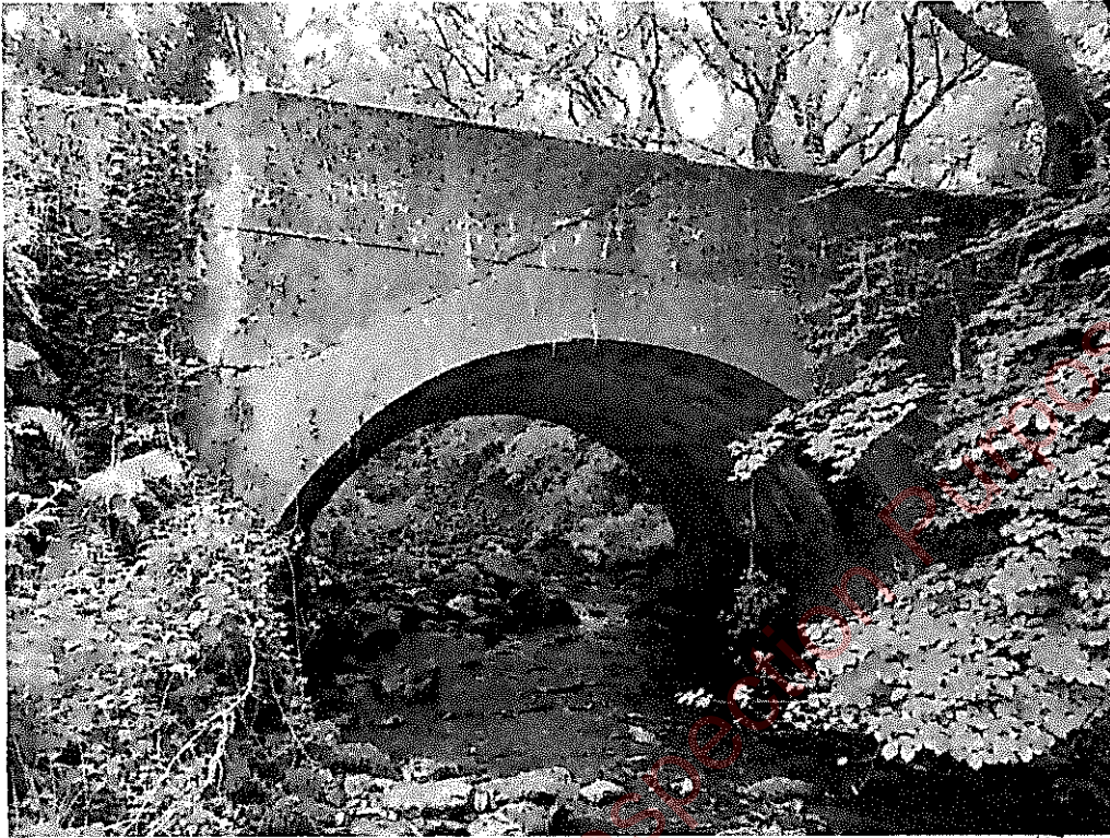
General view of the south elevation, note damage to parapet and west spandrel
