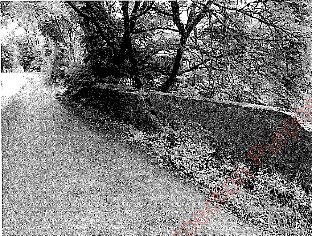
South parapet showing partial collapse extending from the centre of the bridge
