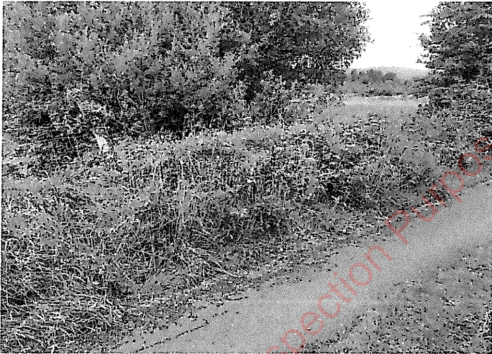
Stone masonry wall on the D/S side of the bridge in poor condition and very overgrown with vegetation. Masonry block wall on the U/S side of the bridge as seen in previous image,
