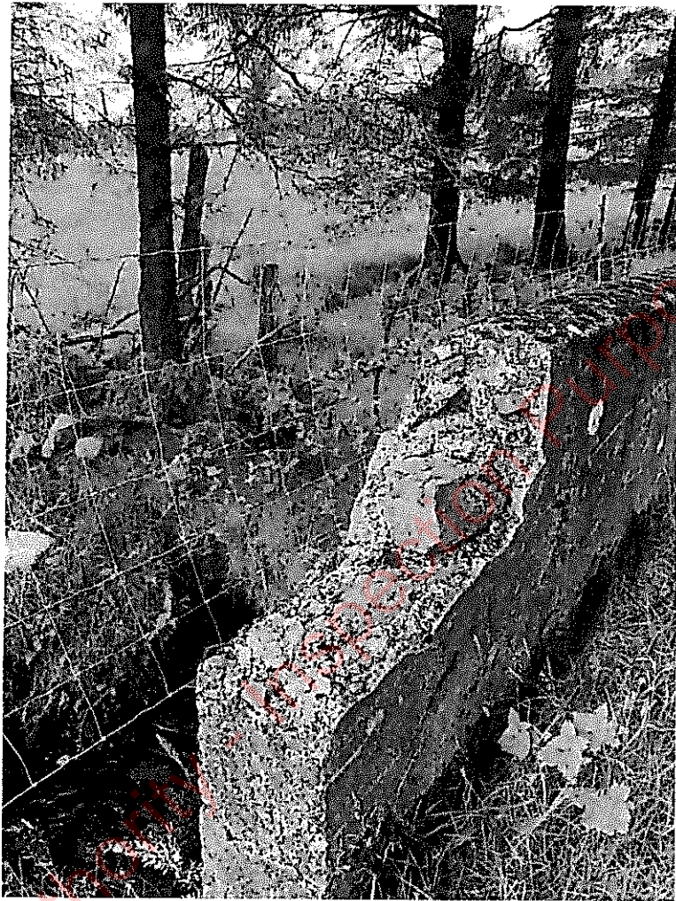
Knocked section of the downstream parapet
