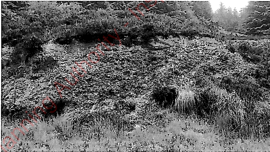
Figure 6-5: Exposed overburden cut with evidence of erosion/shallow slips (ITM 516203E, 582876N)
