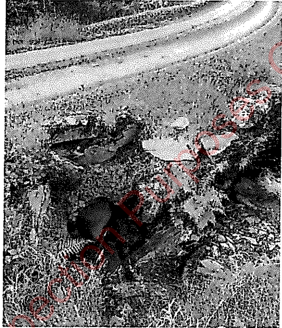
Image : 14 Two twin wall drainage pipes crossing under road. Depth of cover approx. 500mm
