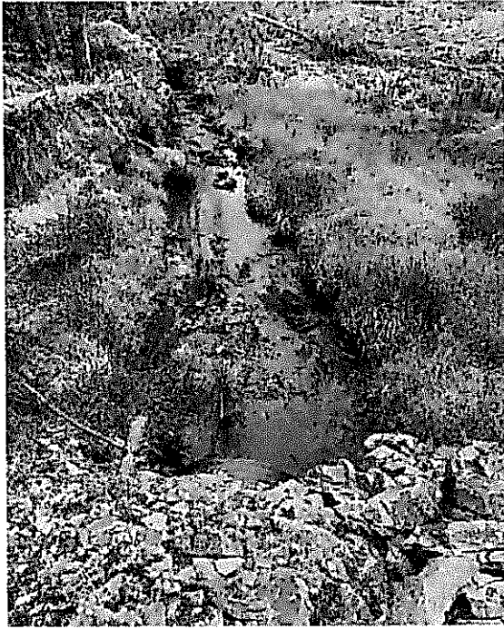
Image : 82 Stream crossing track at this location with a partial collapsed storm pipe
