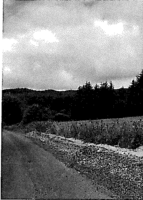
Image : 31 Joint bay on the road here with a links box and communications chambers visible
