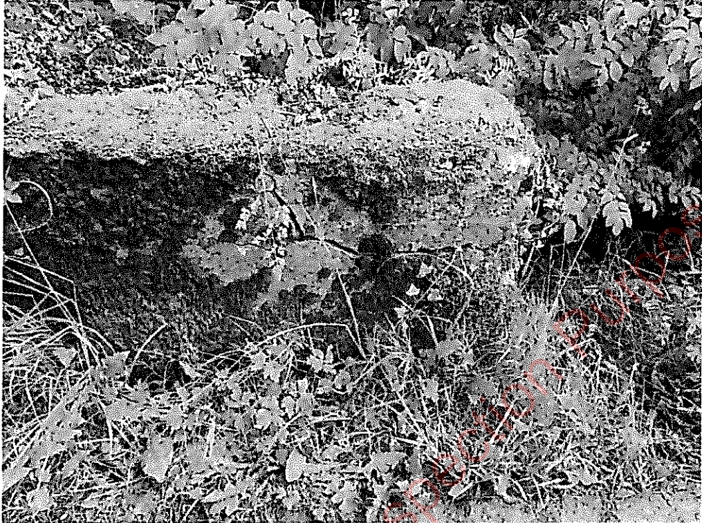
Local damage to the west parapet
