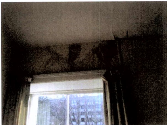
Fig. 35 Example of decay due to water ingress from breaches in roof coverings, at 2 nd floor (later intervention) level
