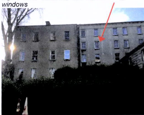
Fig. 23 North elevation of Milltown Park, which was vertically extended in the late 19 th century. The north elevation of its rear, higher, extension was constructed in the 20 th century.
