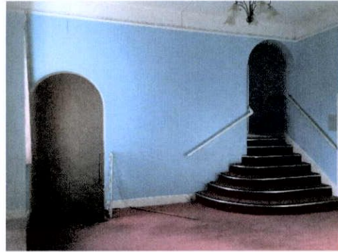
Fig. 30 First floor level infilled entrance hall with later wall painted blue. Curved stair leads to vertical extension wing above a former orangerie.
