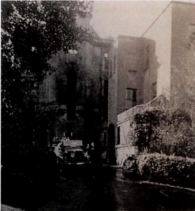
Fig. 16 The fire damaged exterior of the Finlay Wing, indicating its original height of three storey over basement with pitched roof over.
