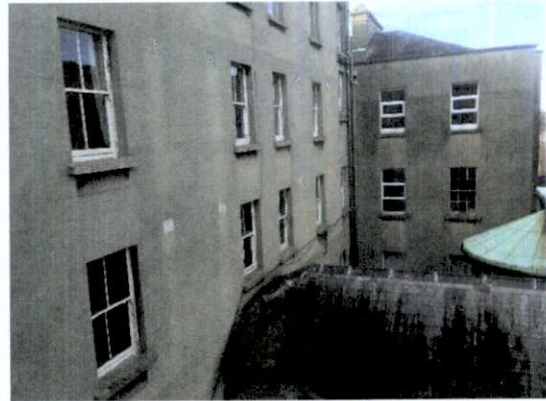
Fig. 40 View of the (later) northern extension from a rear 1 st floor window of Milltown Park house, towards the opposing (original) H form building comprising a lower building, possibly intended to align with MPH.
