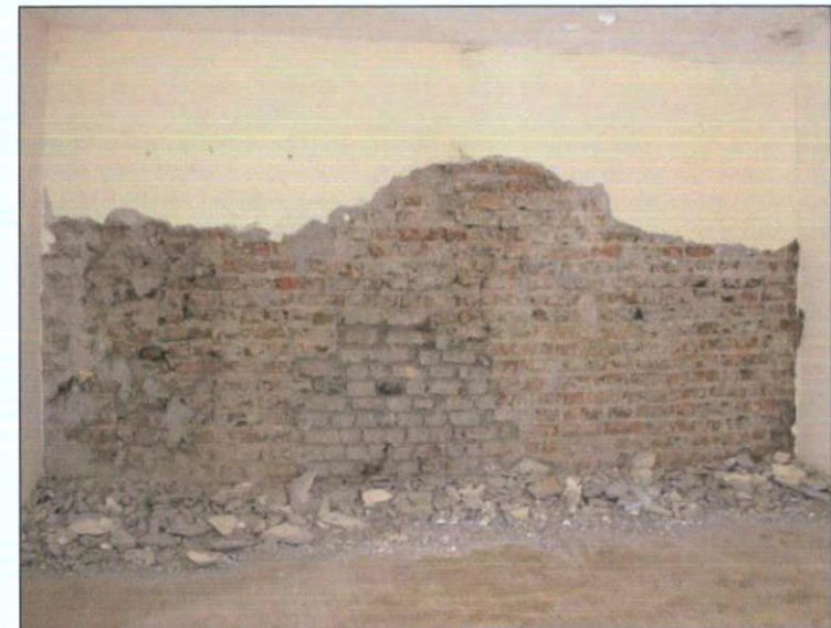
P 15 Infilled opening identified under plaster at first floor level, front room, 13 Moore Street, October 2020.
