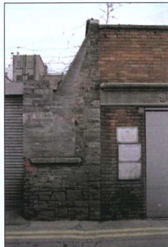
P 12 Evidence of possible bullet damage at rear of 57 O’Connell Street Upper
