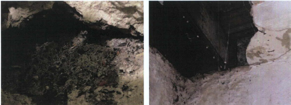
Fig.4.7.7: The clinker concrete used to form the rear, party and internal walls is a distinctive mix with coarse angular brick shards as aggregate; and this material was also used for the construction of Nos.4,5 and 6 Moore Street.
