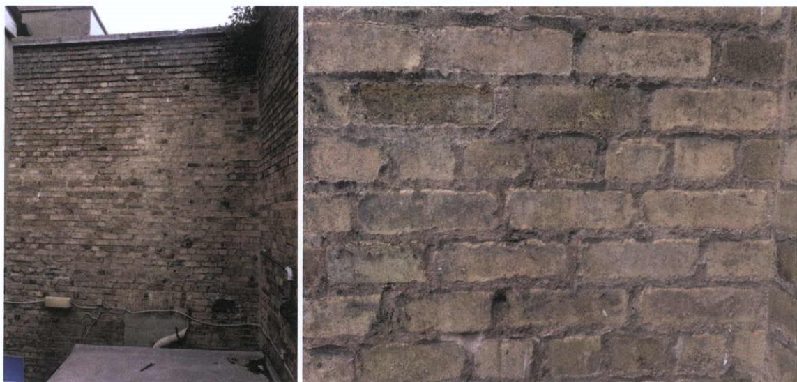
Fig.4.1.1: General view of the brickwork at the rear of 37 Henry Place adjacent to the alley separating Nos.9 and 10 Henry Place.
