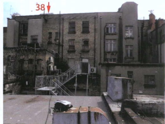
Fig.4.2.3: No.38 Henry Street forming part of a terrace using identical c.1920 yellow stock brick.
