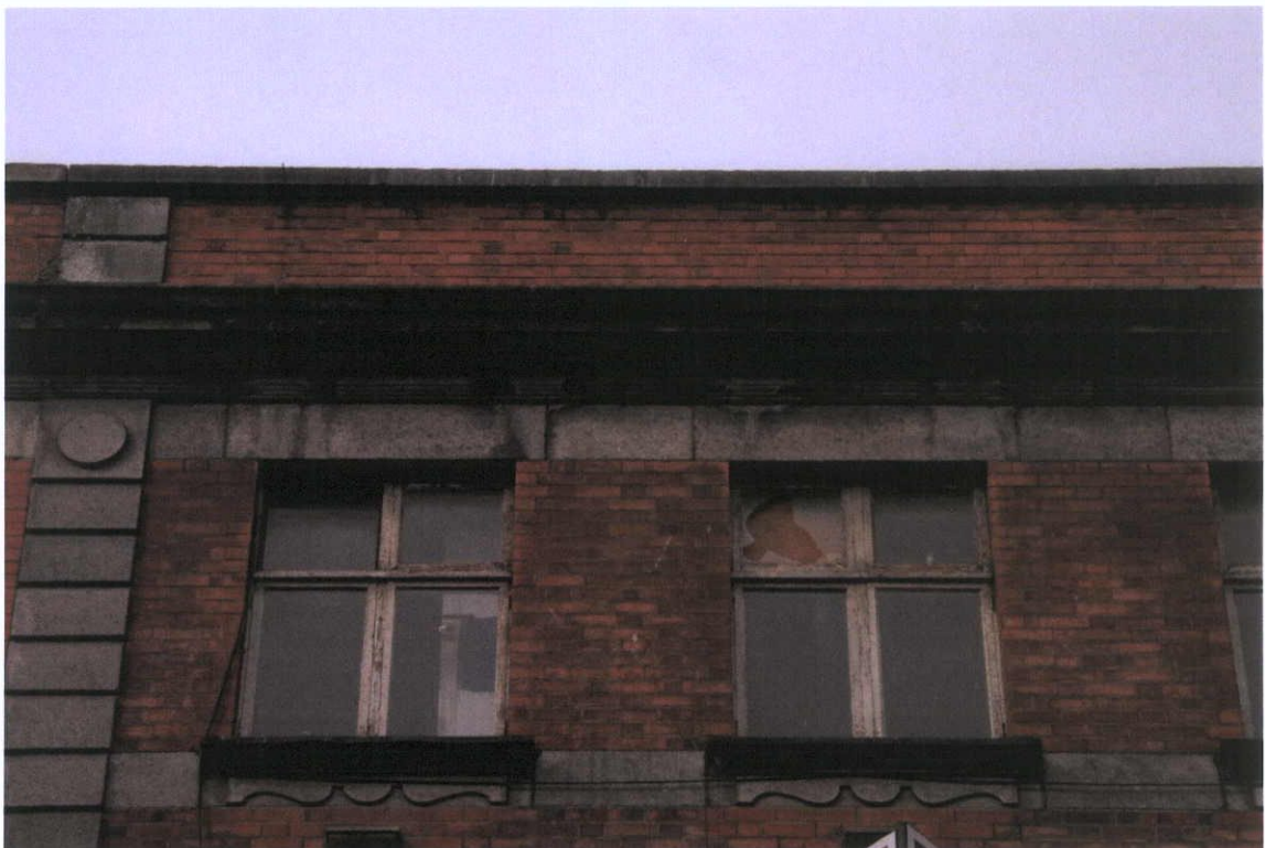
Fig.4.4.2: Soiled brick and granite detailing at upper floor level.
