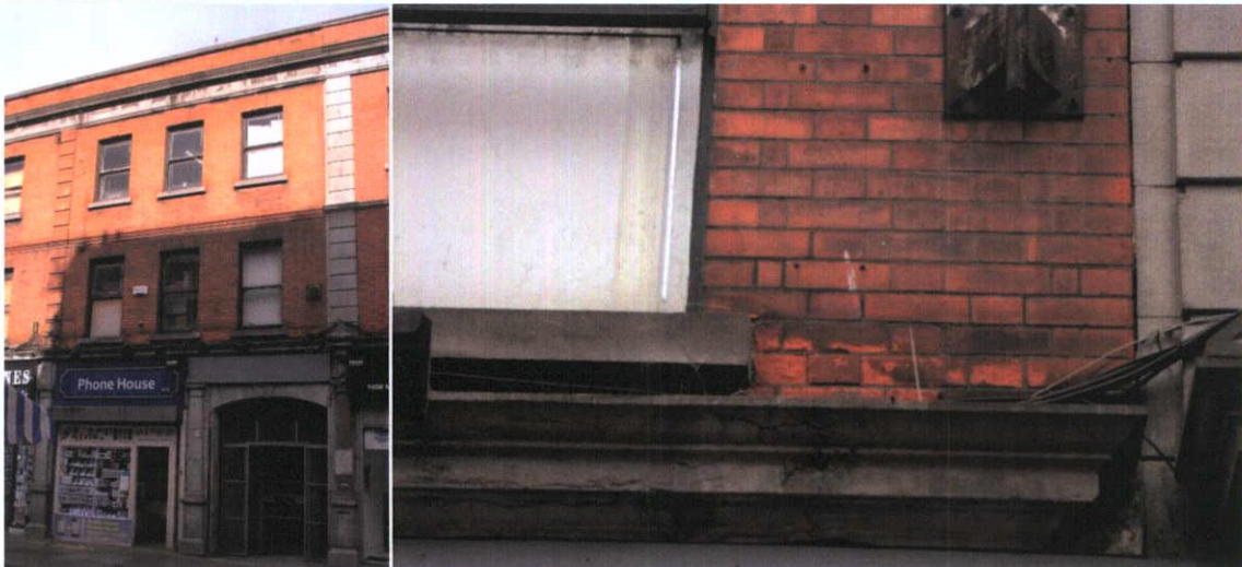
Fig.4.7.2: No.3 Moore Street built with machine-cut homogenous red brick with limestone used for window cills and architectural detail. The masonry is soiled, exaggerating certain stone features.
