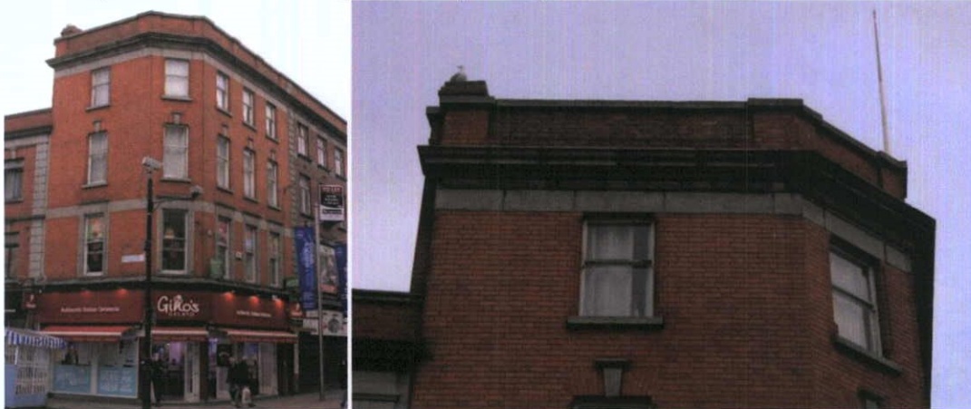
Fig.4.5.2: Soiled brick and granite detailing at upper floor level.
