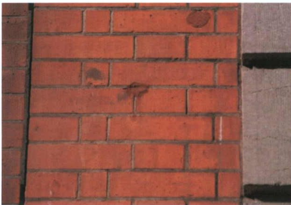
Fig.4.2.2: The brickwork and limestone detailing on the façade of 38 Henry Street has been cleaned and small 'plastic' mortar repairs (appearing dark red) seen.
