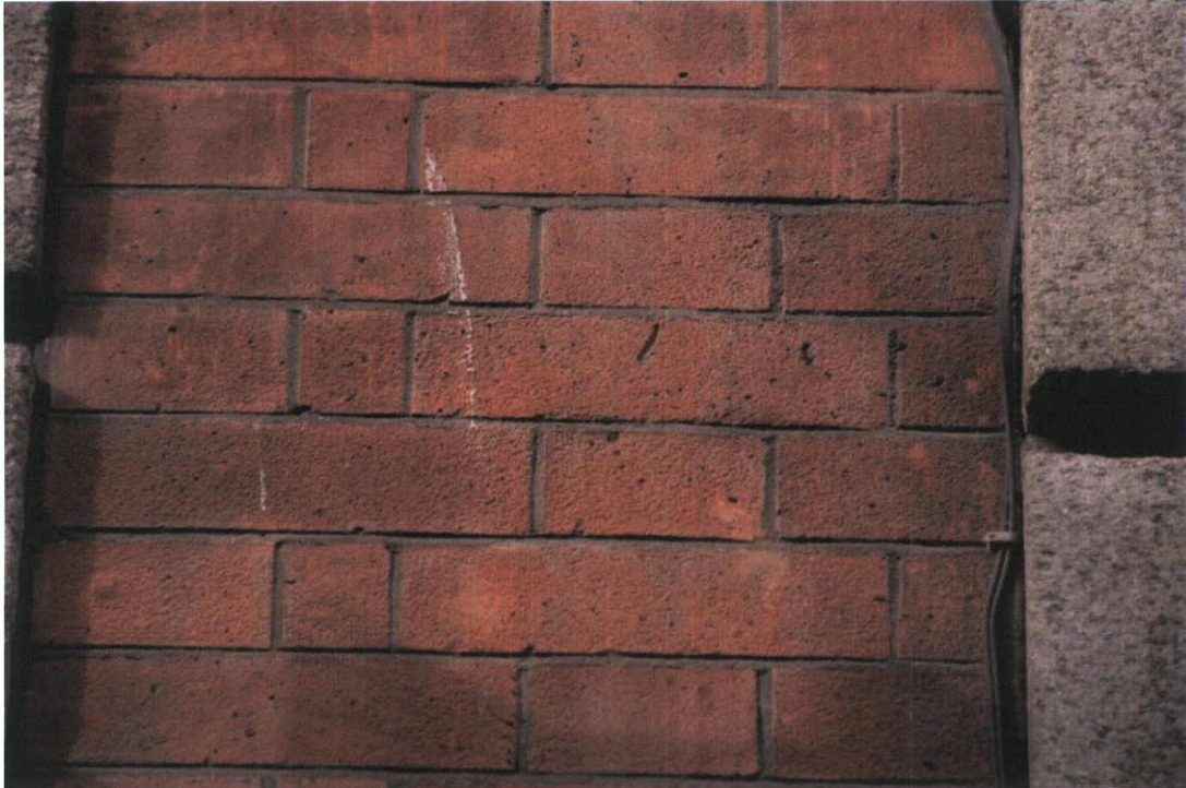
Fig.4.3.3: Detail of the brickwork on the façade of 39 Henry Street showing a damaged surface (probably from past cleaning) and the edge of the Leinster granite detail.
