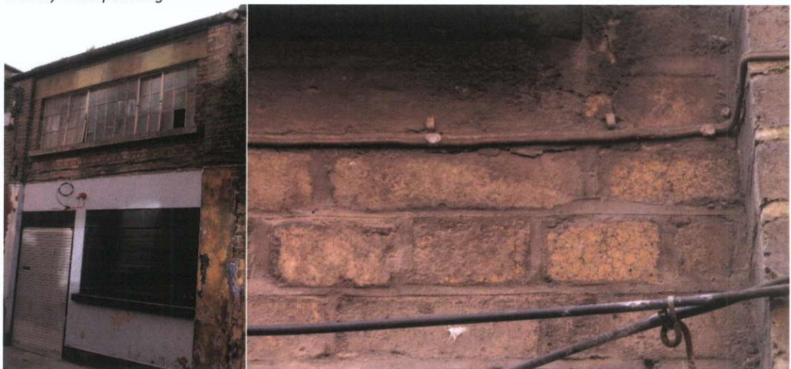
Fig.4.13.2: The brick is pointed in lined Portland Cement-based mortar, and the buff-coloured brick has crazele (network of minor cracks also called crack networks, termed 'crazing' for terracotta).
