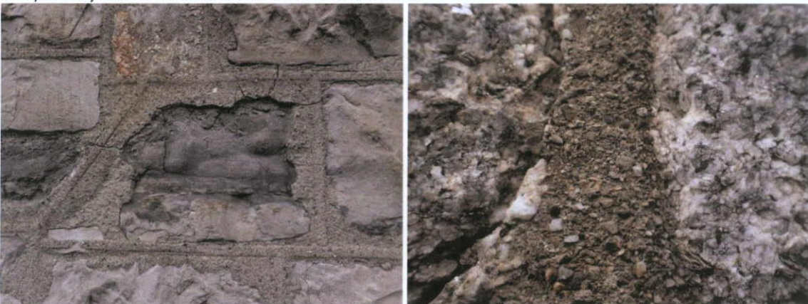
Fig.5.5.6: Mid-twentieth century Portland Cement-based repair and pointing mortar.
