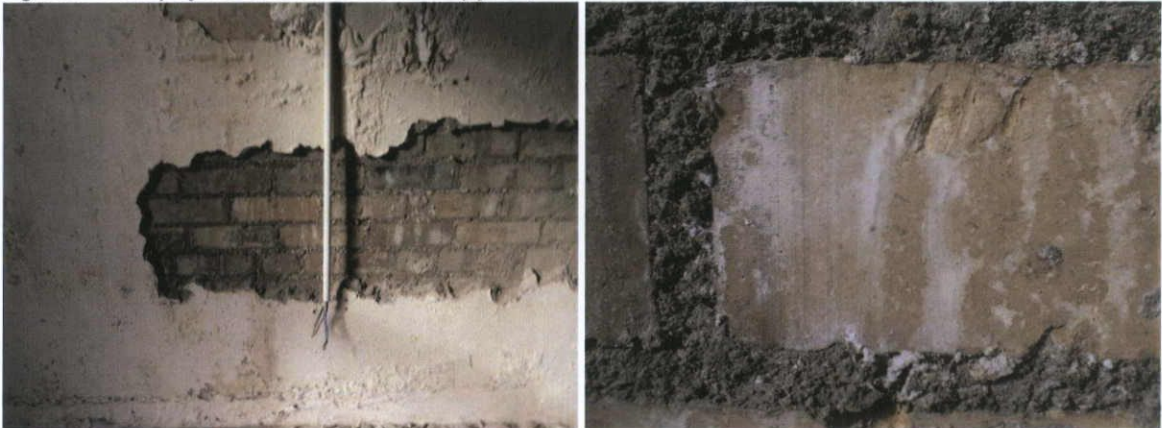
Fig.6.1.8: The north wall (party wall with No.22) consists of kiln-fired extruded machine-cut yellow stock brick. Similar brick is found in the link building between 42 O'Connell Street and O'Connell Hall.
