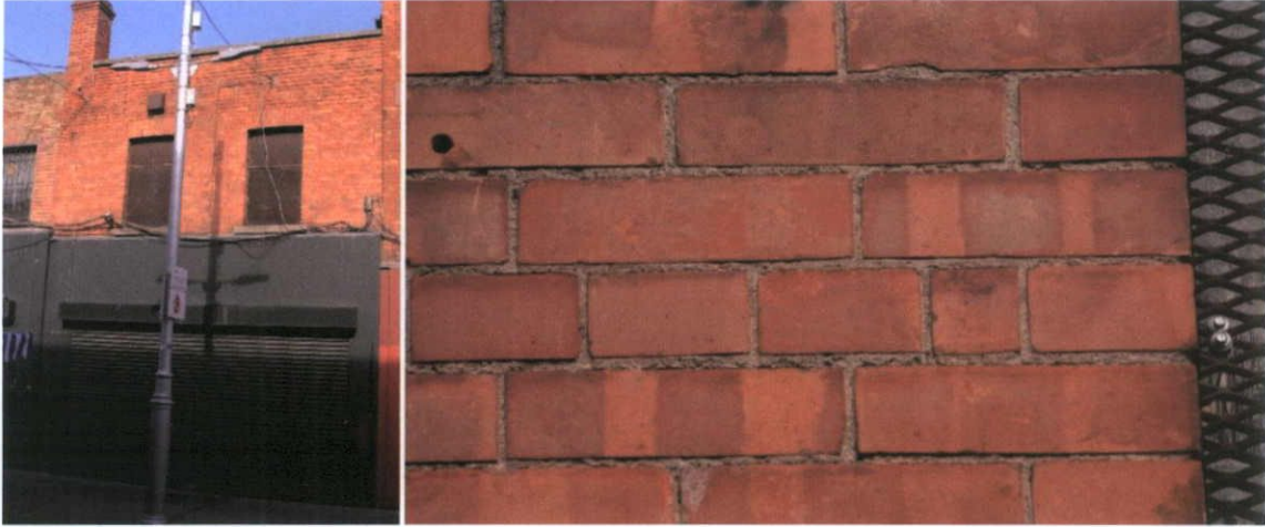
Fig.5.7.3: The first floor has brick with 'kiss marks' from the firing process. This type of brick is found in buildings in Dublin City from the 1890s and used thereafter for a number of decades.
