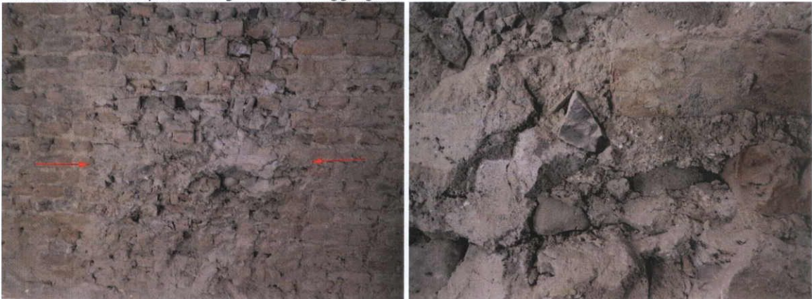
Fig.5.3.7: 'Creephole' at ground floor level, front room, south wall: showing a change in construction with the insertion of broken cobbles and other materials bonded in a cement-based mortar.
