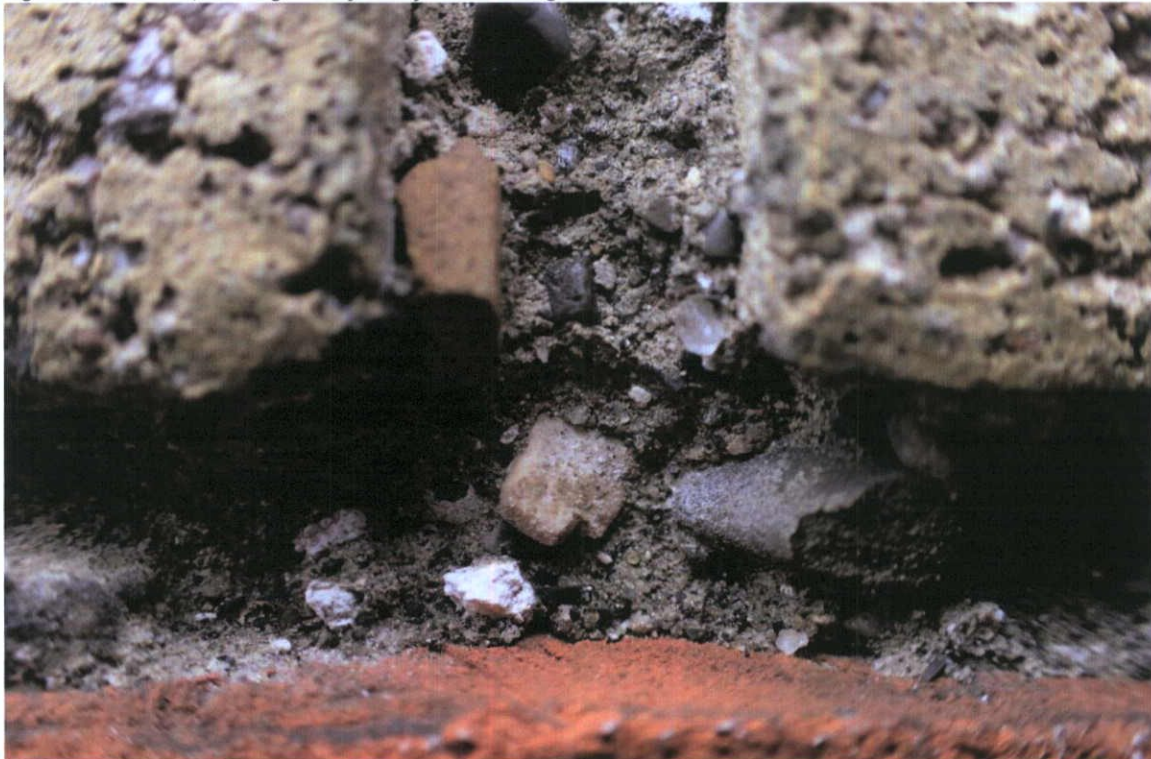
Fig. 4.17.4: Poorly sorted limestone, sandstone, quartz and chert aggregate with coarse lime lumps in a water-damaged lime binder.
