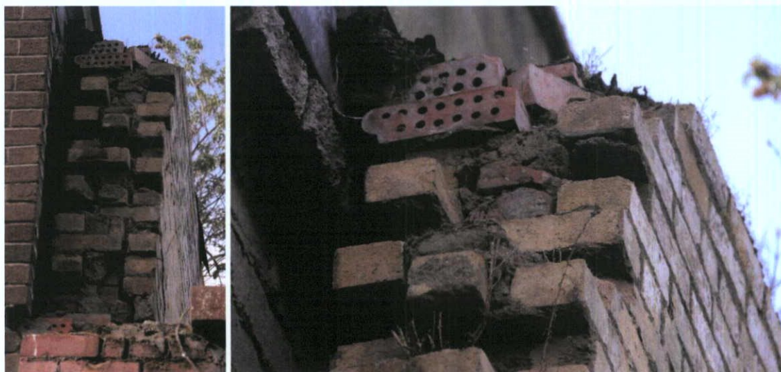
Fig.5.6.2: Detail of the inner leaf of yellow stock brick forming the west wall at first floor level; with moulded perforated red brick indicating decorative treatment to the west elevation of the building.
