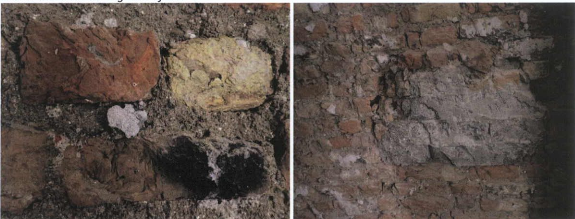
Fig.5.3.9: Late eighteenth/early nineteenth century brickwork, ground floor, south wall, with concrete infill.
