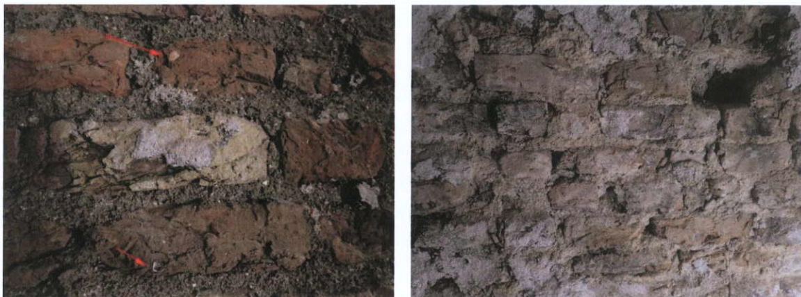
Fig.5.3.2: 13 Moore Street, Ground Floor, Rear Room, north face of south wall (party wall with No.12). Detail of handmade brickwork from the internal party wall between Nos.13 & 12 Moore Street with burnt shell inclusions (arrowed) within the fired clay matrix (left). The original brick at first floor level (right) is also hand-made and of varying dimensions and qualities, laid in deep lime mortar joints. These are ‘place’ bricks intended to be coated with a lime plaster.
