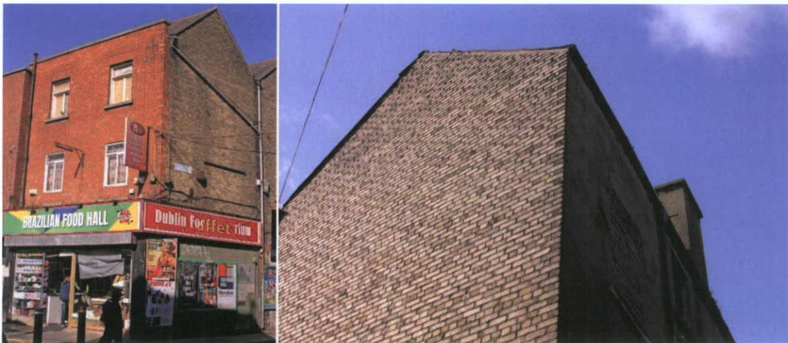
Fig.5.1.1: Façade and side (south) elevations of No.10 Moore Street with the rear (east) rendered.
