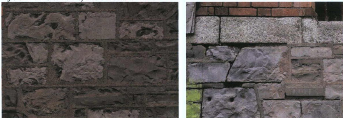
Fig.5.5.2: The coursed hewn Calp limestone masonry has been repointed with coarse-grained Portland Cement strapwork, which was also used as a repair mortar at the time of application.
