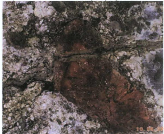
Fig. 4.17.9: Crushed brick in the mortar.
