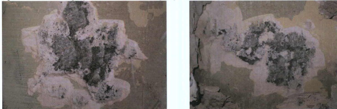
Fig. 4.17.13: Cement used to plaster the inside of the north wall at first floor level.
