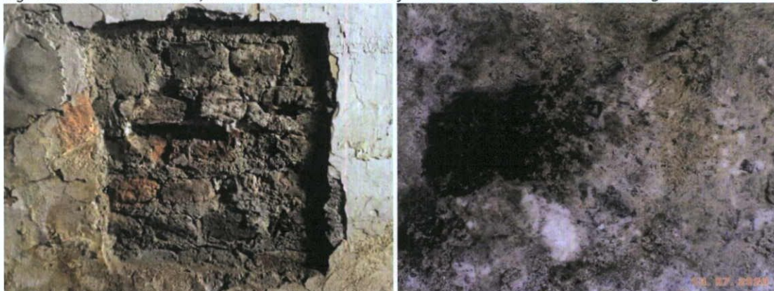
Fig.4.16.19: Nineteenth century stock brick and Calp limestone masonry at the south end of the west wall at ground floor level of No.10 Henry Place, coated with a cementitious internal plaster.
