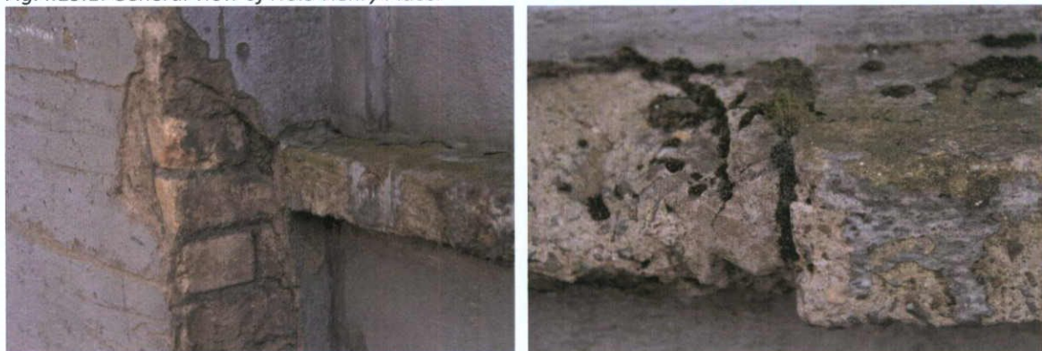
Fig.4.15.2: The piers on the façade are of yellow stock brick, while the cill is concrete.
