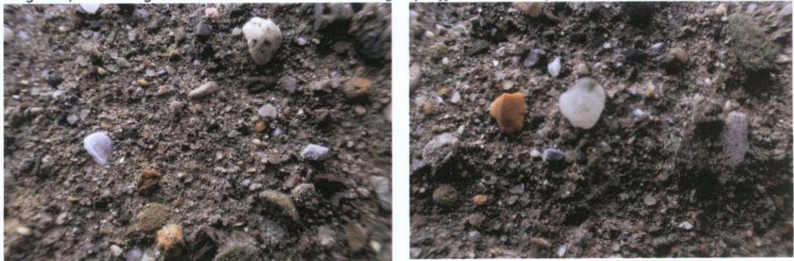
Fig.4.10.3: Detail of the aggregate standing proud of the surface of the render at the rear of No.6 Moore Street consisting of rounded natural aggregate and shell.
