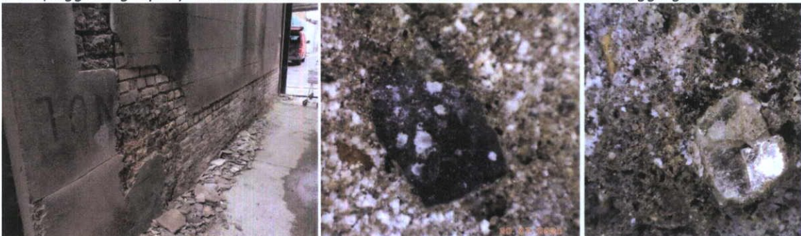
Fig.4.16.6: The north end of the east wall is coated with a Portland Cement render above a c.1920s yellow stock brick masonry substrate.
