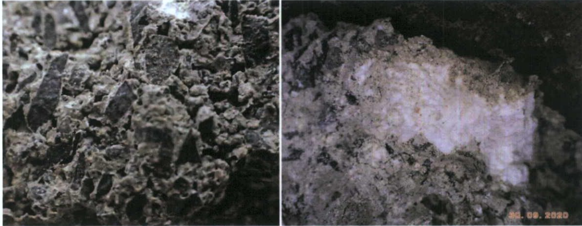
Fig.5.3.10: Detail of 20 th century concrete repair to the south wall at ground floor level.
