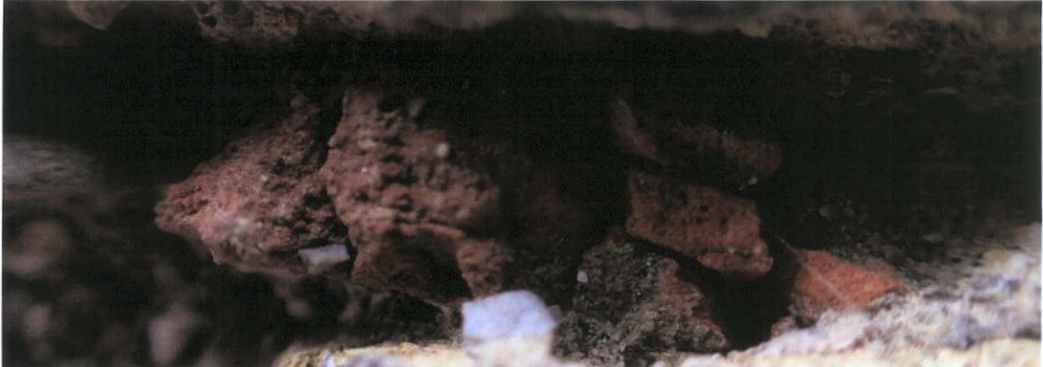
Fig.4.17.5: Crushed brick used as aggregate in the mortar.
