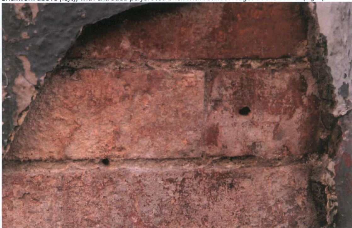
Fig.4.14.4: Detail of the curved brickwork at the north-east corner of the building.
