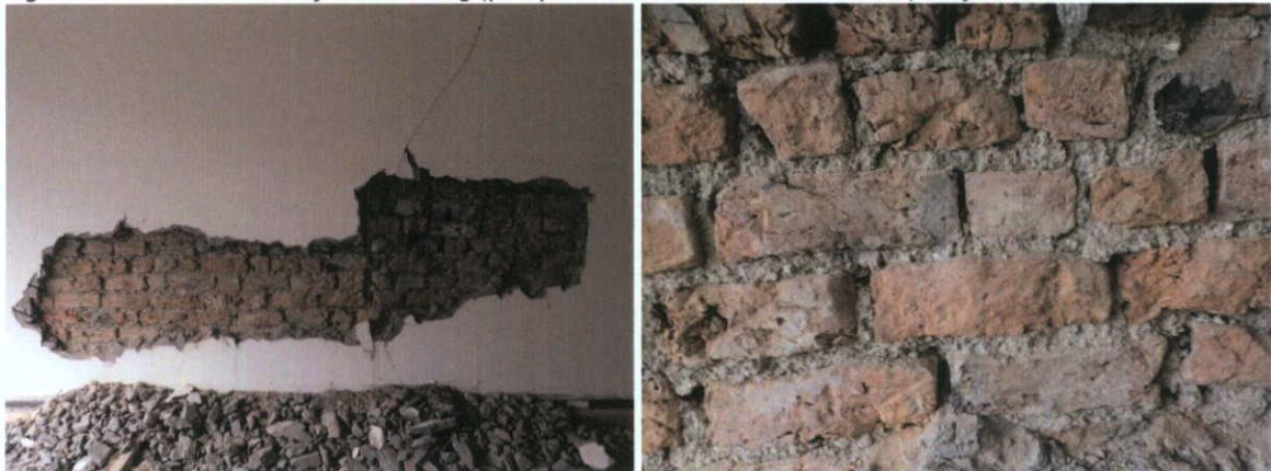
Fig.6.1.4: The party wall between Nos.20 and 21 is of hand-made clamp-fired brick laid in deep lime mortar joints.
