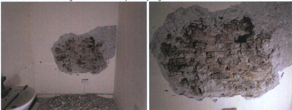
Fig.5.3.5: Internal party wall at upper floor level showing hand-made brick bedded in a lime bedding mortar.
