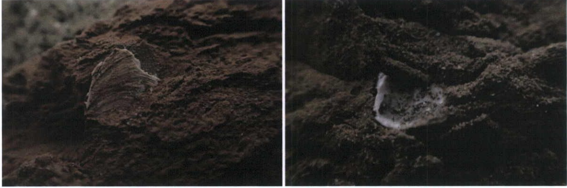
Fig.5.3.3: 13 Moore Street, Ground Floor: Detail of burnt shell inclusions in the brick.
