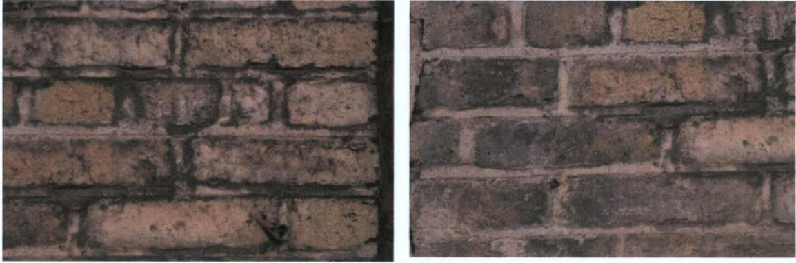
Fig.4.13.3: Soiled buff-coloured brick in lined flush pointing.
