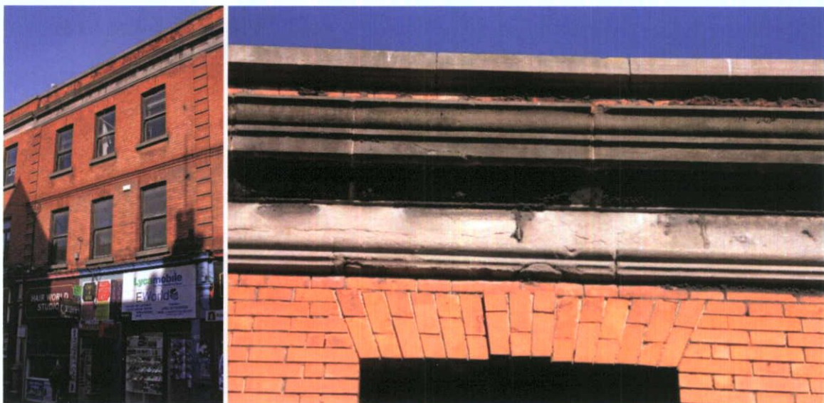
Fig.4.10.1: Limestone frieze and brickwork at No.6 Moore Street, matching that of Nos.3-5.
