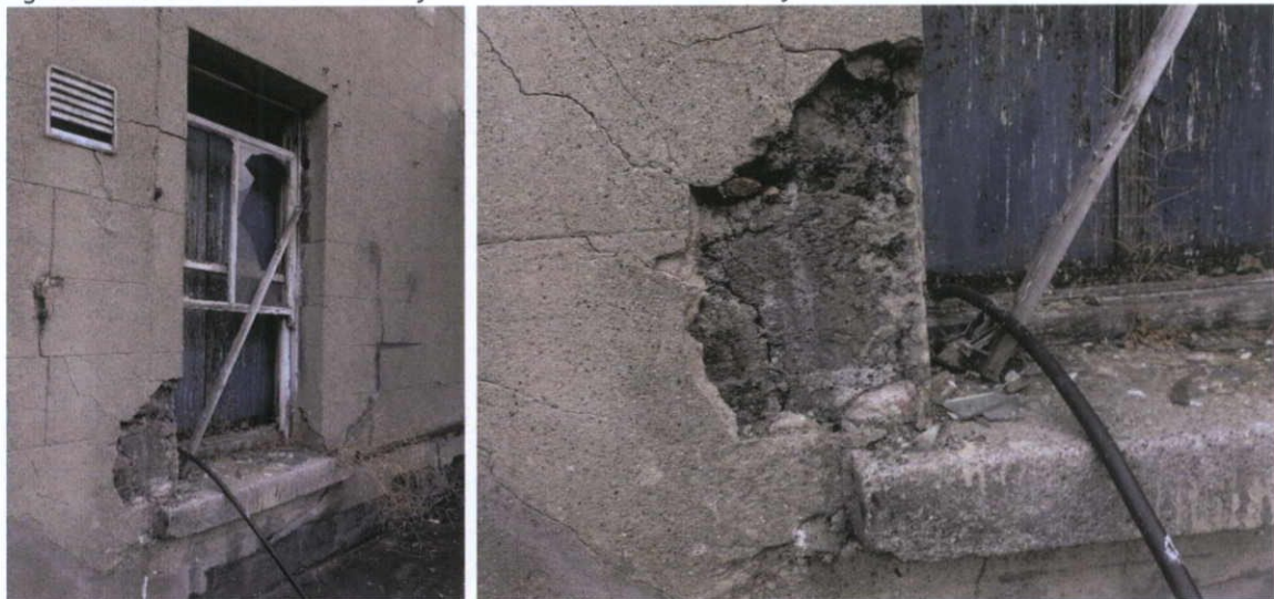
Fig.4.8.5: Ruled and lined Portland Cement render over a concrete structure. Rear elevation, No.4 Moore St.
