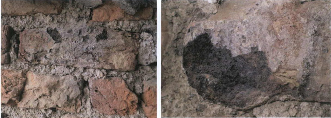
Fig.6.1.7: Many of the bricks were unevenly fired, with sections over-fired and partially vitrified.
