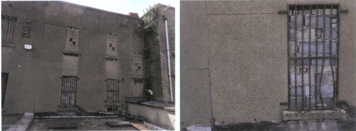
Fig.4.10.3: The rear elevation has a Portland Cement render which has weathered differently to its neighbor, indicating that the cement binders are slightly different in composition.
