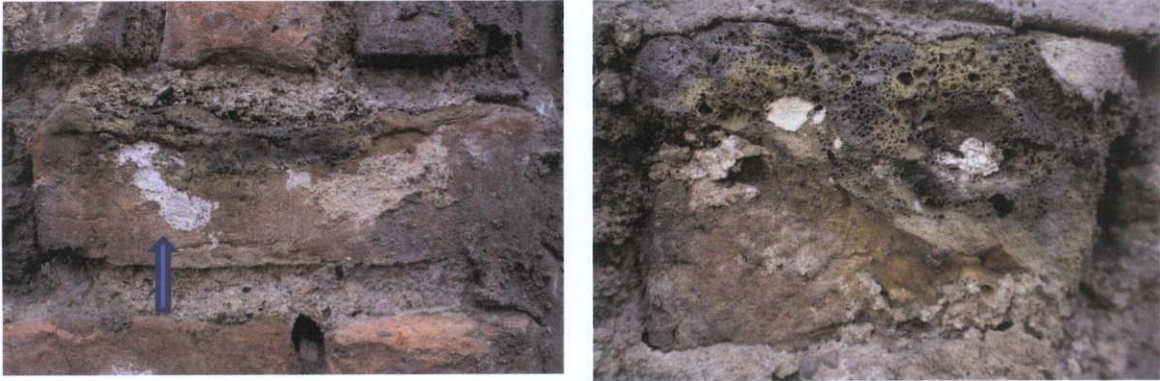
Fig.8.4.12: Poorly-fired place brick in a deep lime-based mortar joint, showing a remnant of a lime-based plaster adhering to part of the surface (left, arrowed). Right: Poorly-fired place brick showing vitrified areas, voids, warping, but with traces of limewash on the surface of the brick.
