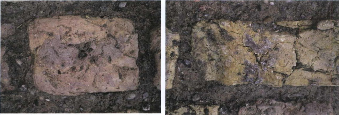
Fig.5.2.5: Stretcher and header views of yellow-pink stock brick with shrinkage cracks laid in coarse-grained pozzolanic lime mortar.
