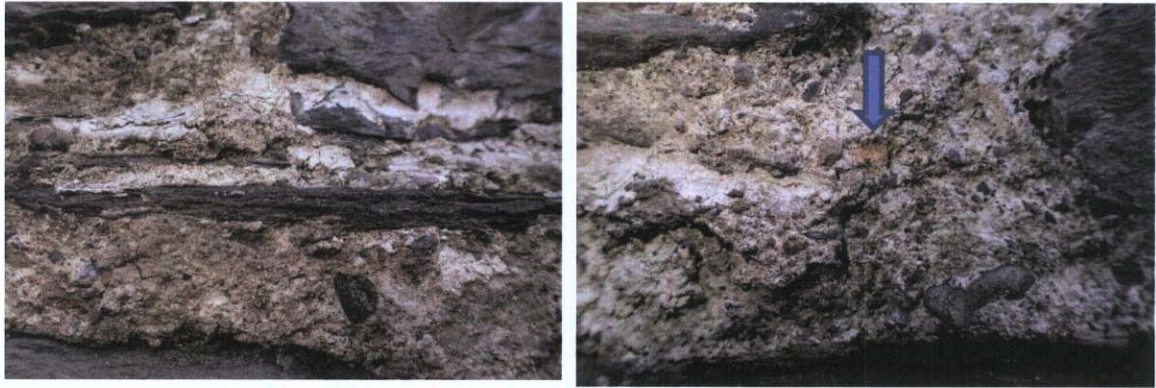
Fig.6.4.6: Slate pinnings (left) and coarse brick aggregate (right, arrowed) as an occasional component of the aggregate fraction of the mortar.
