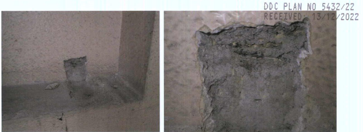
Fig.5.2.16: 1920s yellow stock brick in cementitious mortar exposed in the party walls of the south wall at ground floor level.
