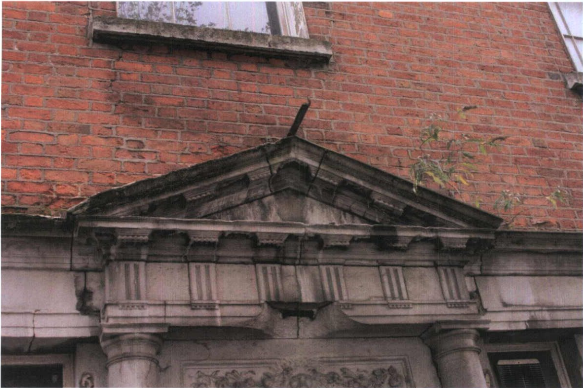
Fig.4.3.2: The red facing brick is laid in Flemish bond and has been repointed throughout in a Portland Cement-based mortar. The repointing is failing (losing bond) in areas of saturation, and loss of the surface of the brick is evidence in many areas.
