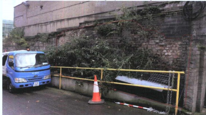
Fig.8.4.10: The western section of the wall is composed of red and yellow place brick, and appears to represent internal lining.
