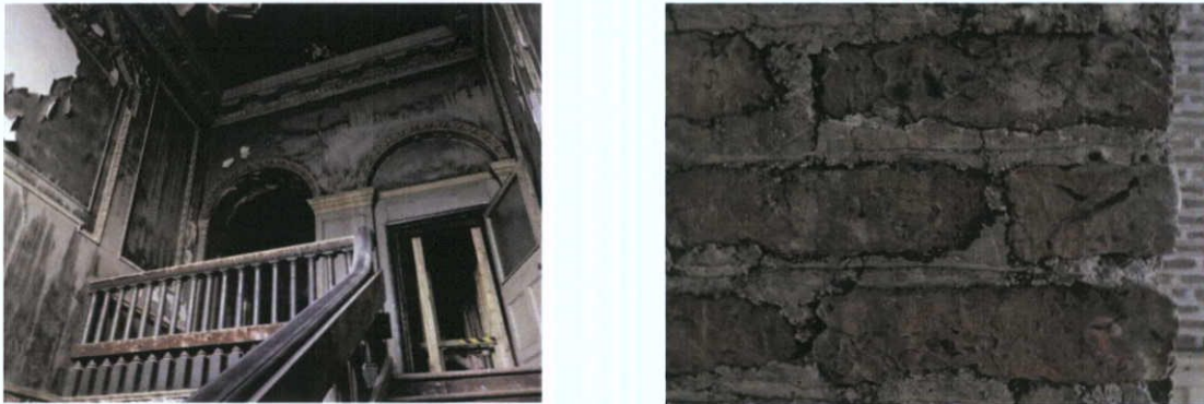
Fig.4.3.8 (left): The internal wall surfaces of the staircase retains decorative plasterwork finishes and enrichment. These were not sampled, but analysis of Georgian plasterwork elsewhere in north Dublin City indicates that the flatwork and the enrichment are composed of different materials – each of which uses very high-grade components and required a great deal of craftsmanship in successful execution.
