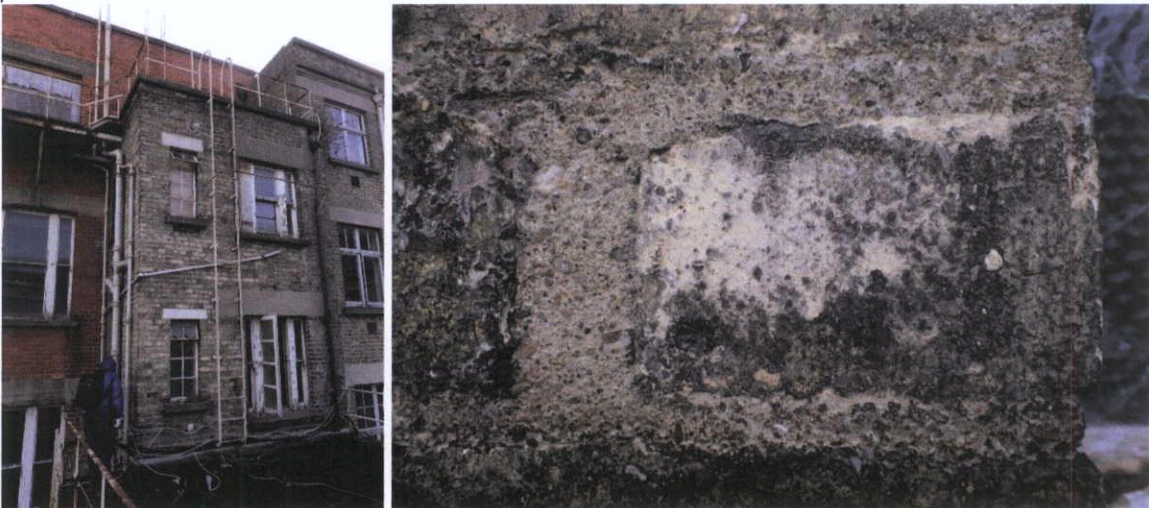
Fig.5.2.6: The return is made from c.1920s yellow stock brick in a lime-cement mortar, with concrete lintels above the openings and forming the parapet coping.
