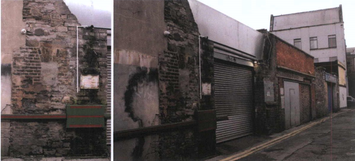
Fig.5.4.2: Calp masonry fabric at the rear of the building with a brick window, and a granite cill.
