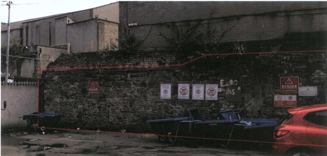
Fig.6.4.5: The eastern section of the wall consists of hewn Calp limestone masonry bonded in a lime-based mortar.
