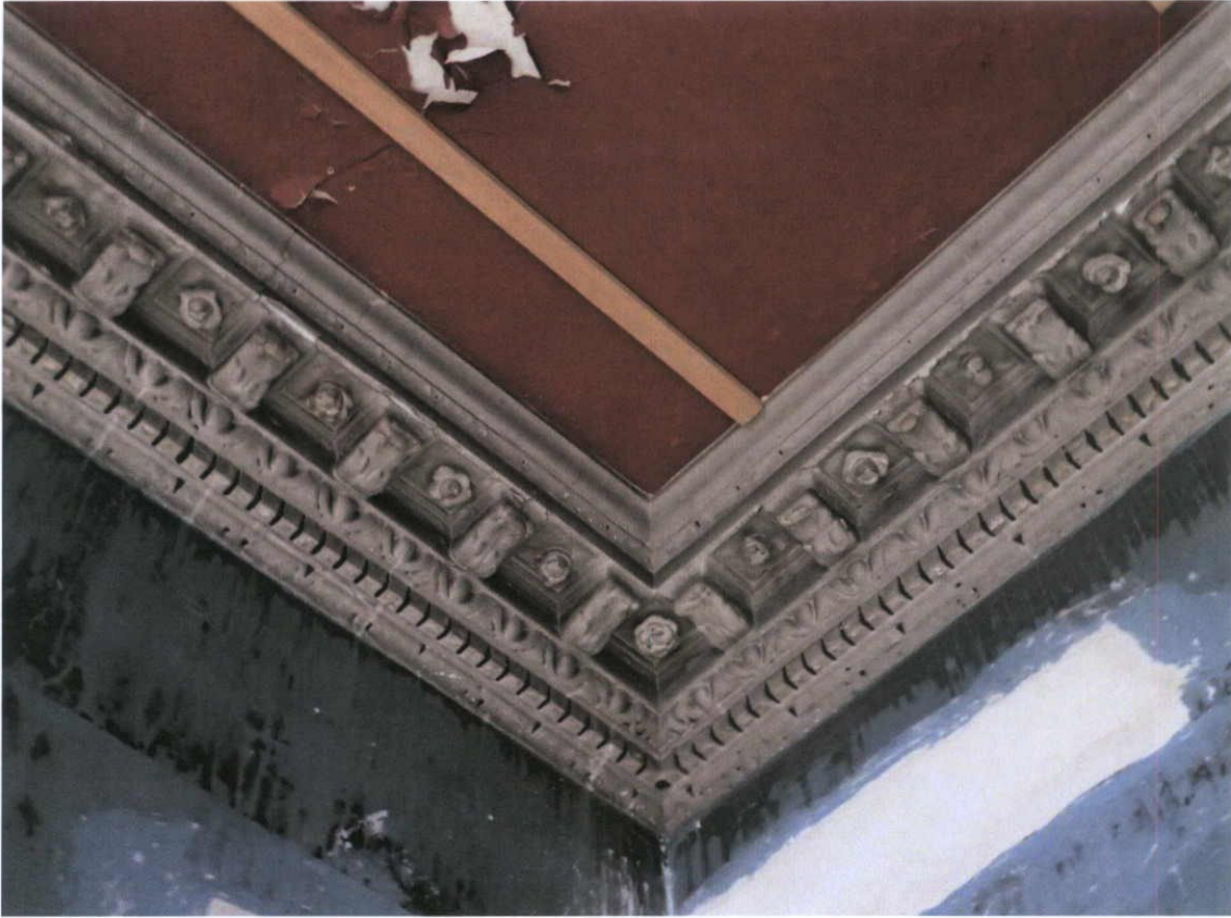
Fig.4.3.12: Detail of the ceiling at the head of the staircase showing three different materials:
