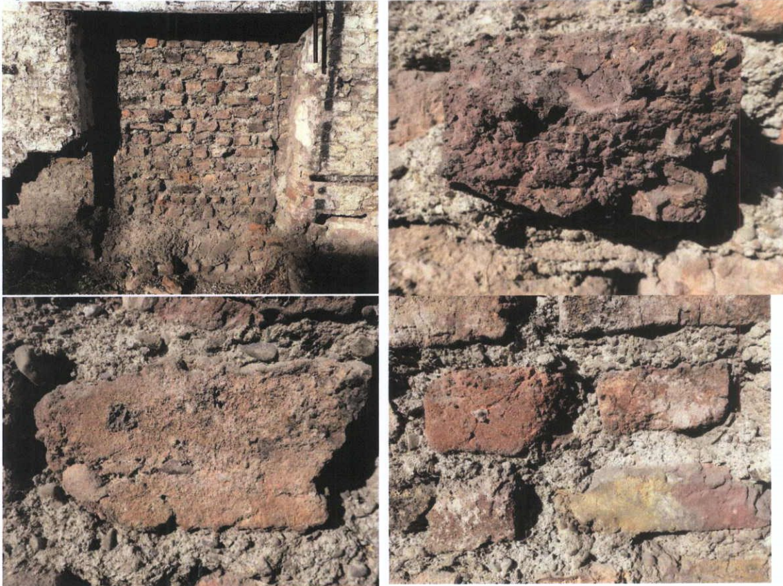
Fig.5.3.20: Irregular clamp fired brick in lime bedding joints infilling a door opening.
