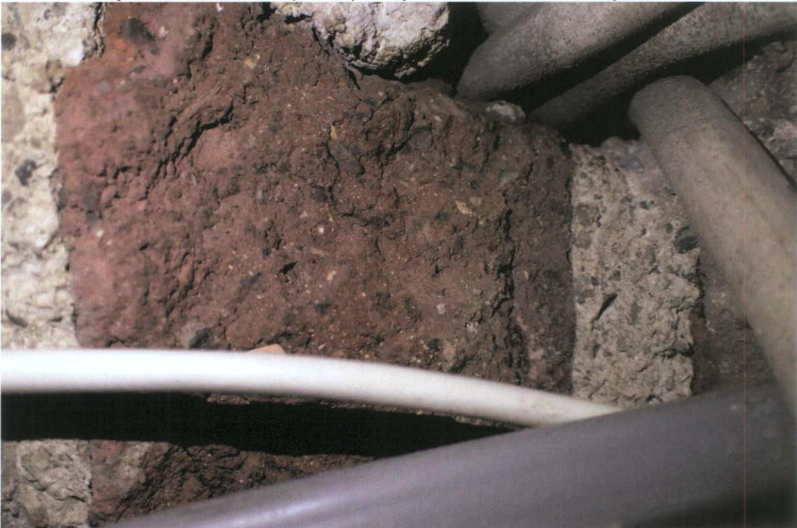
Fig.5.1.9: Detail of a clamp-fired brick seen at basement level showing limestone inclusions.
