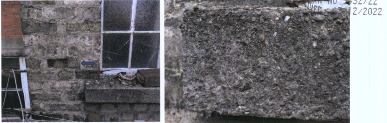
Fig.5.2.7: The window cills are of concrete. The 1920s yellow stock brick also includes occasional earlier clamp-fired yellow stock brick (arrowed), likely to be an example of salvage.
