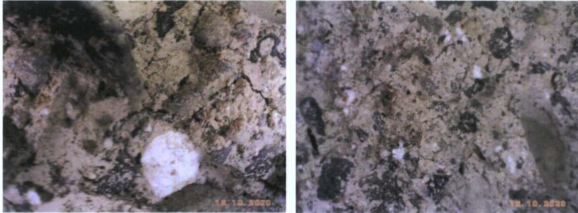
Fig.4.3.14: Microscopic views of a coarse-grained pozzolanic lime mortar used to bed the place brick of the internal walls and wall linings of 41 O'Connell Street. Note common occurrence of large lime lumps.
