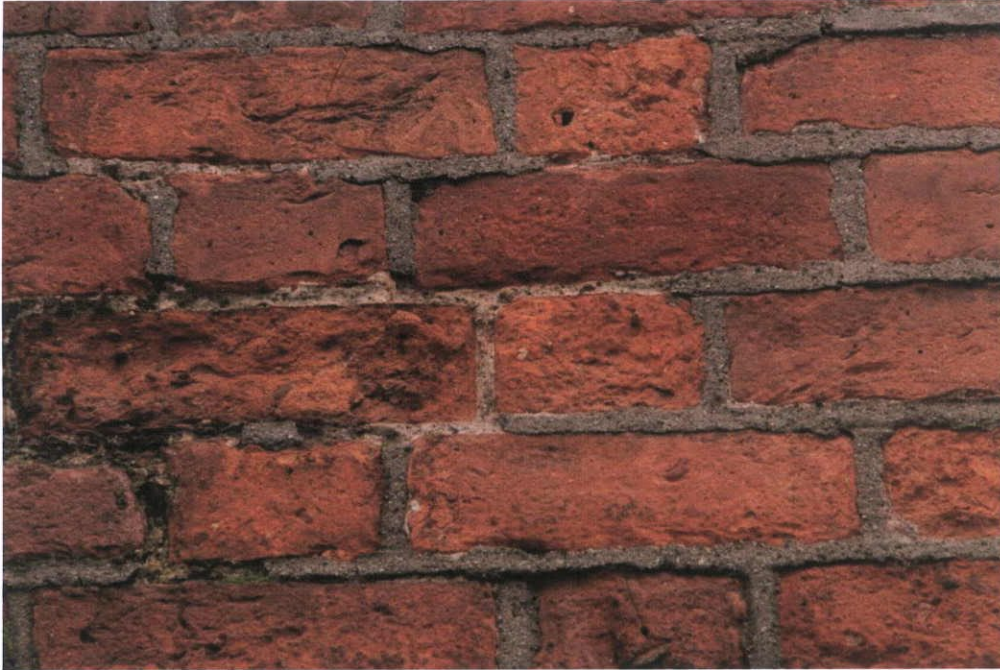
Fig.4.3.4: The façade brick is handmade and contains abundant inclusions of pebbles and fired material. The lime bedding mortar contains relatively coarse aggregate (up to \frac{1}{2} the joint height).
