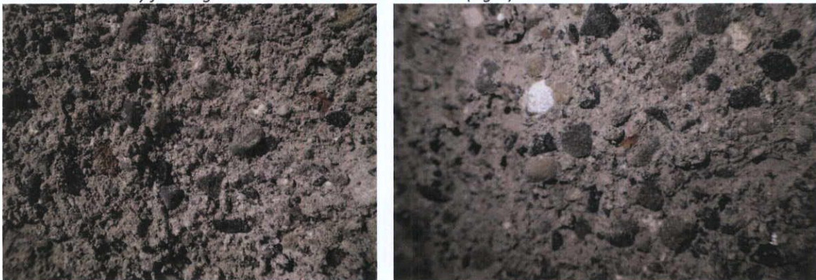
Fig.5.7.9: The render on the north wall of the building is reasonably similar in texture and composition to that found on the south wall. These may be Georgian period building.
