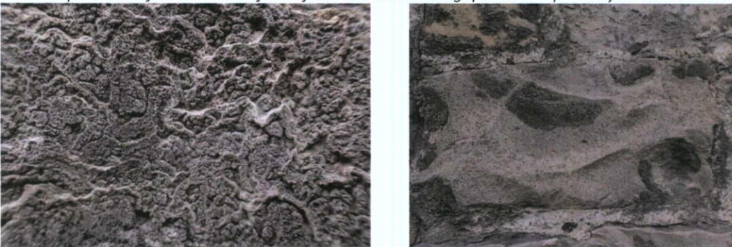
Fig.5.6.7: Black gypsum soiling crusts on the surface of the mortar and stone.
