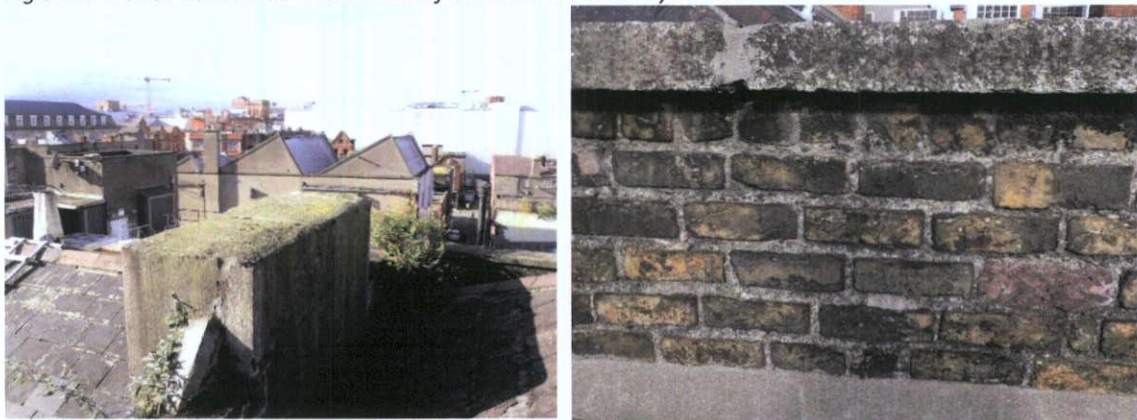
Fig.5.7.15: The cut-down Chimney B on the west side of the roof (left) and the granite-capped stock brick wall linking the two chimneys (right).
