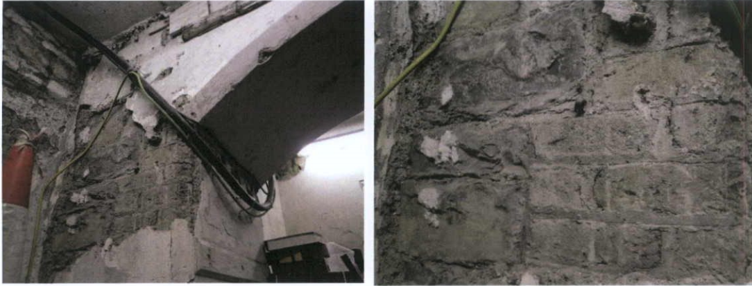
Fig.5.7.5: The nineteenth century brick arch has been repointed in Portland Cement and painted.
