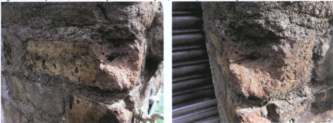
Fig.5.4.7: Groove in the brick jamb; said to be from a bullet during the 1916 Easter Rising.
