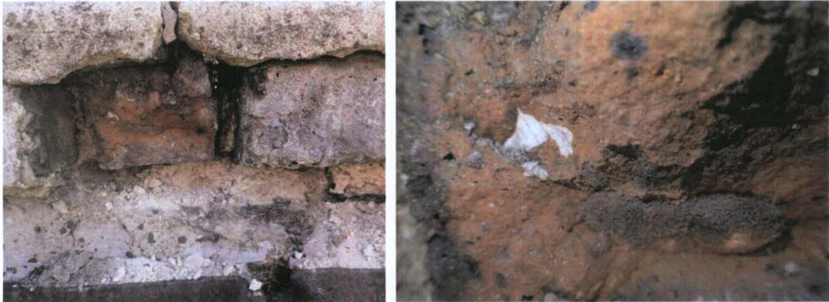
Fig.5.7.14: Shell contained in the brick of the eastern chimney stack.
