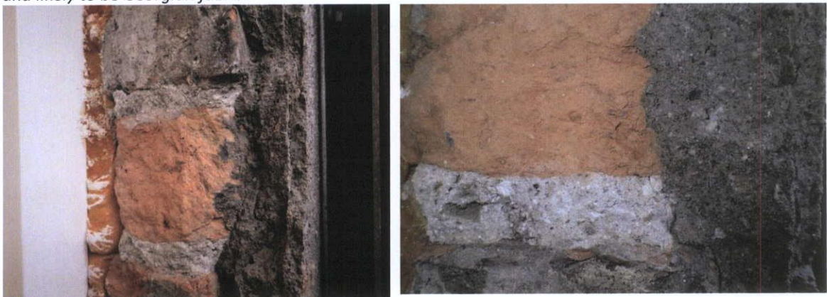
Fig.5.9.5: The rear elevation is coated with multiple layers of Portland Cement render above red stock brick.
