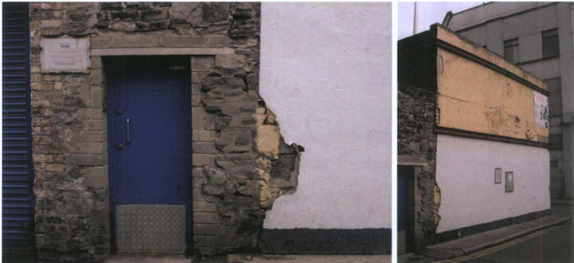
Fig.5.8.1: The rear boundary Calp limestone wall (60a O’Connell Street) is set in a pozzolanic lime mortar similar to others seen along the lane, and is probably eighteenth century Georgian fabric.
