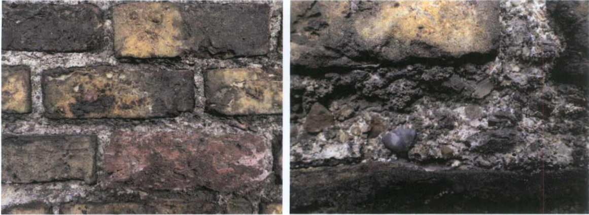
Fig.5.7.16: The soiled party wall is composed of hand-made clamp-fired yellow stock brick bedded in deep coarse-grained lime mortars with scarce crushed brick. This brick is very similar to that transported to Dublin City along the canal networks, and probably mid-nineteenth century.
