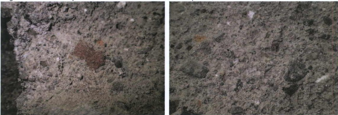
Fig.5.7.7: Limestone aggregate with large coarse lime lumps and crushed brick and brick dust pozzolan on the lime render over the southern basement Calp limestone wall at the front of the building.
