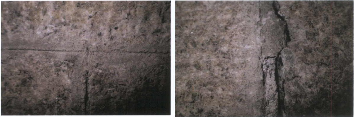
Fig.5.7.11: Detail of the joints of the granite ashlar in the strong room showing the lime bedding mortar beneath the later Portland Cement pointing.
