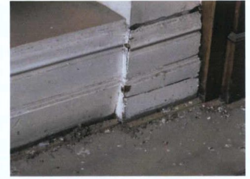
Plate 57: F-5 – Detail to skirting
