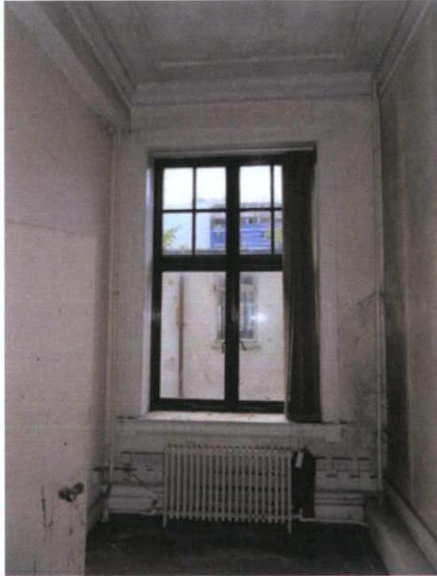
Plate 61: F-4 – View to west
