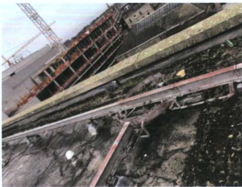
Plate 29: West roof — track for cleaning windows
