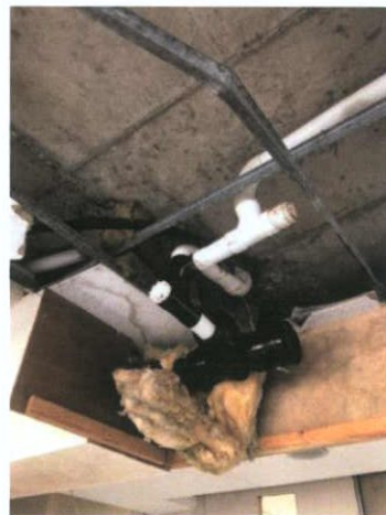
Plate 361: Exposed drainage pipes in ceiling
