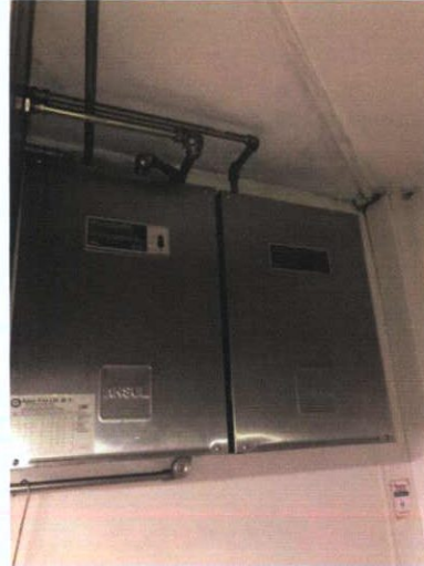
Plate 149: Fire suppression system located in kitchen
