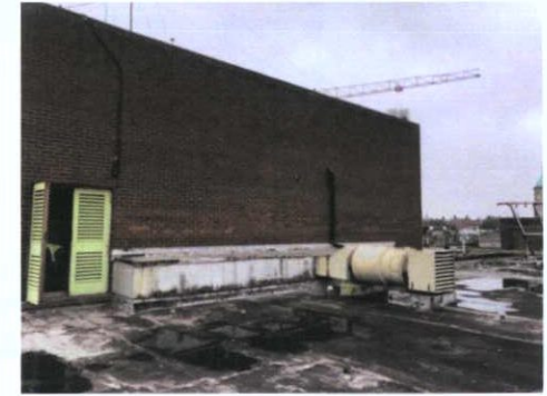
Plate 18: East roof — West 1
