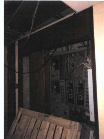
Plate 300: Electrical service cupboard on main corridor
