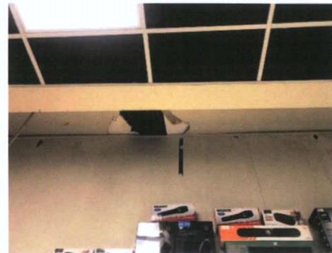
Plate 44: Damage to ceiling in main retail space
