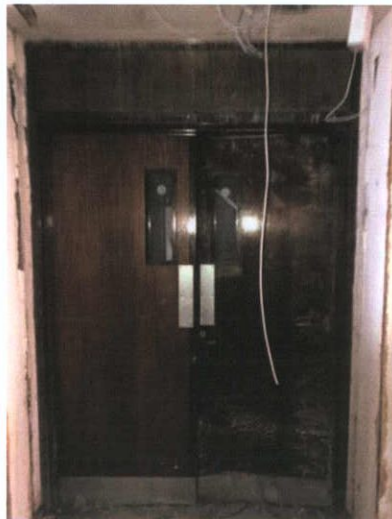
Plate 225: Exit doors to front of building that have been blocked up behind to separate areas
