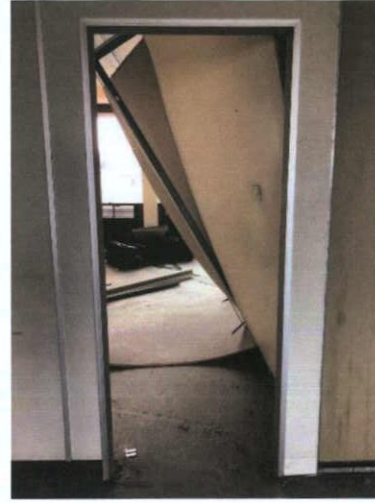
Plate 334: Room 1 — Entrance with damaged stud partition
