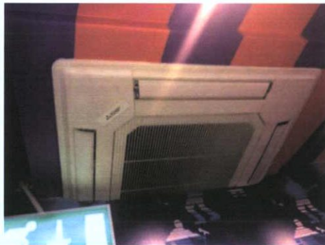
Plate 120: Air Conditioning unit blocked by partition wall
