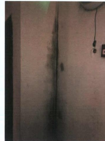
Plate 59: Signs of dampness and mould growth at rear of restaurant
