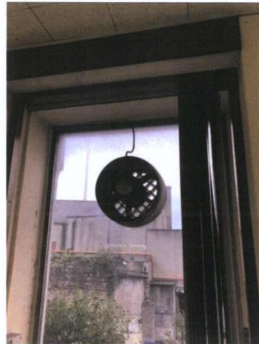
Plate 222: Ventilation fan in reception window
