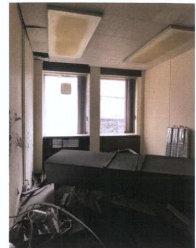
Plate 224: Image showing suspended ceiling and old lighting in office
