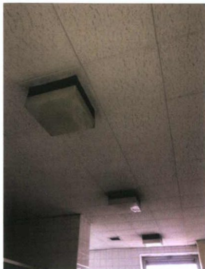
Plate 290: Male WC — lighting and suspending ceiling
