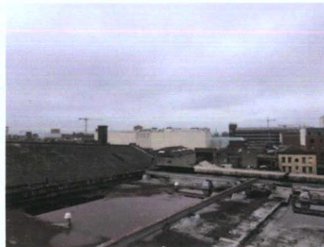
Plate 20: East roof — West 3
