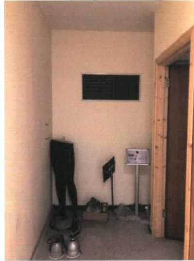
Plate 198: Level entrance lobby showing grille from service riser behind
