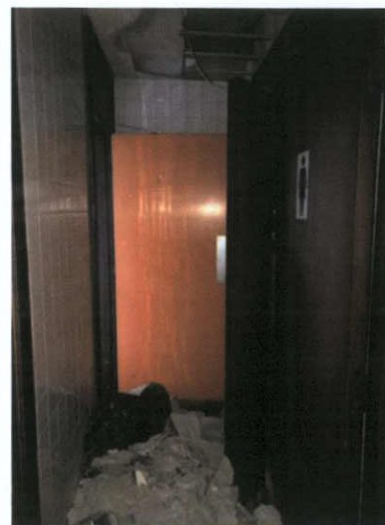
Plate 292: Female WC entry from main hallway- not accessible
