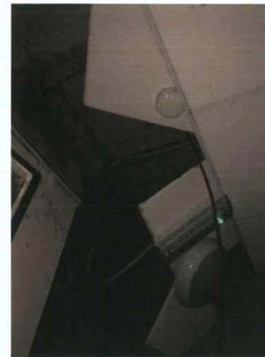
Plate 138: Damage to lighting in fire exit staircase
