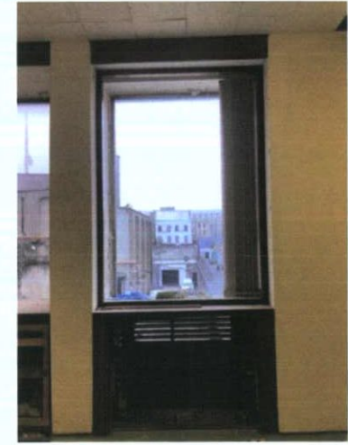
Plate 204: Typical window with ventilation unit below removed and air inlet grilles visible
