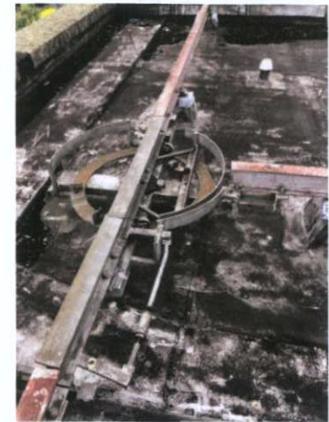
Plate 23: East roof — track for window cleaning crane
