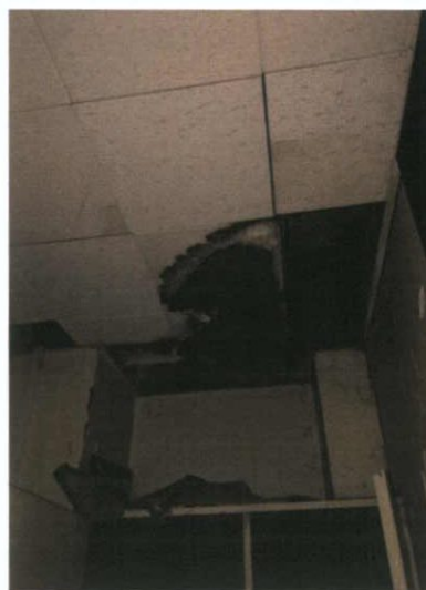
Plate 296: Damage to ceiling of kitchenette
