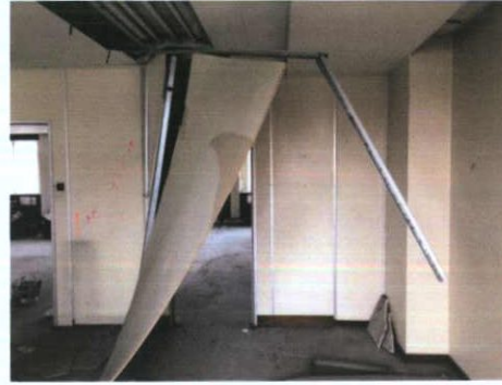
Plate 338: South wall showing damaged partition
