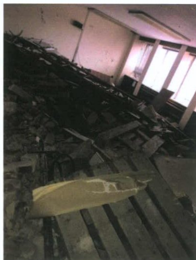
Plate 279: Room 14 — Non accessible due to demolished material
