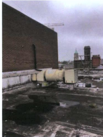
Plate 12: East roof — Ventilation unit
