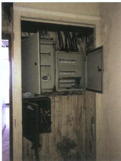
Plate 495: Fuse box at doorway from west stairwell
