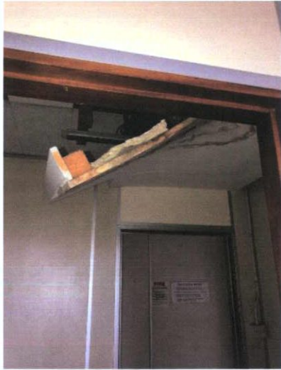
Plate 451: Damage to ceiling in secondary hallway
