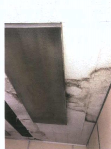
Plate 449: Room 11 — Ceiling water damage
