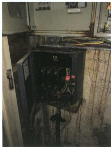
Plate 496: Electrical unit at doorway from west stairwell
