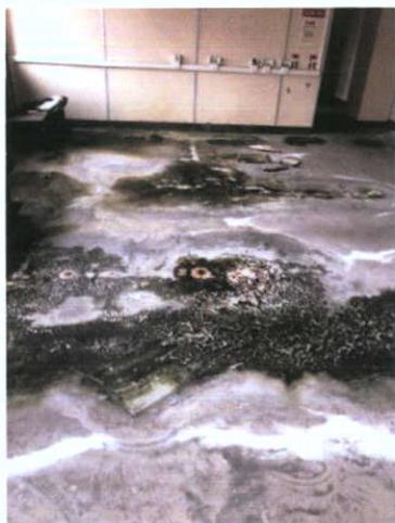
Plate 423: Room 7 — Rot on floor
