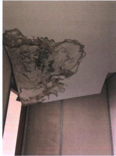
Plate 452: Damage to ceiling in secondary hallway
