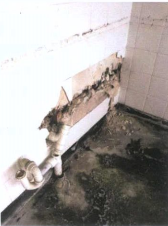
Plate 399: Damage to wall
