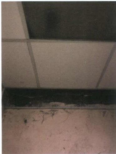
Plate 415: Room 3 — Ceiling damage
