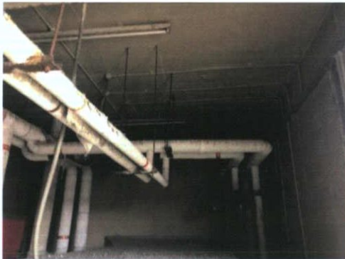
Plate 503: Plant room — Services
