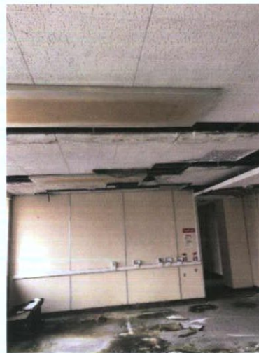
Plate 425: Room 7 — Ceiling damage
