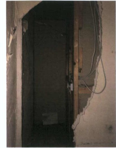
Plate 414: Room 3 — East wall alcove damage
