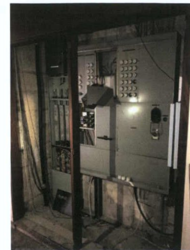
Plate 494: Electrical unit in main hallway
