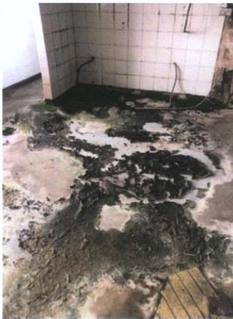
Plate 400: Rot due to leaking roof
