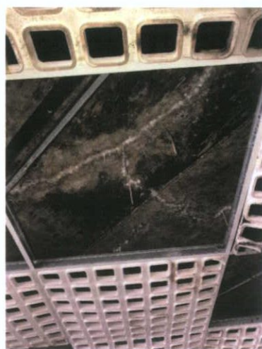
Plate 432: Room 8 — Water leaking through ceiling
