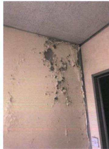
Plate 469: Room 15 — Damage to east wall
