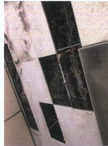
Plate 457: Room 12 — Roof leaking into room
