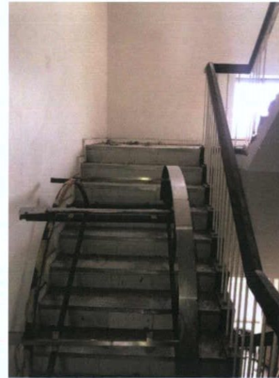
Plate 507: Storage on stair blocking path
