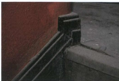
Plate 48: T-5 – Detail to skirting board
