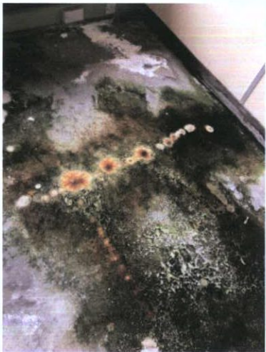
Plate 439: Room 9 — Concrete floor covered in rot
