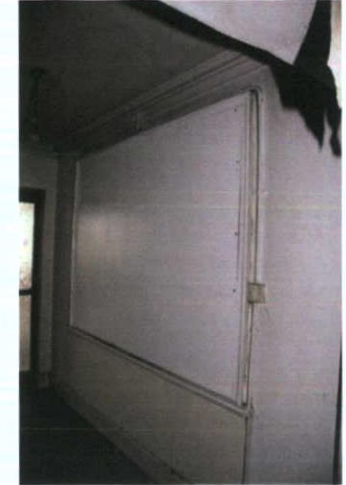
Plate 106: T-2 – Blocked-up window opening to south wall
