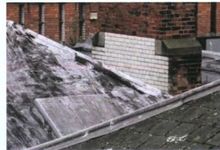
Plate 24: Glazed brick to base of chimney stack to north of Reading Room to reflect light into north-facing rooflight
