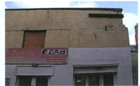
Plate 9: Former slit window, now blocked-up, noted to first floor to south elevation
