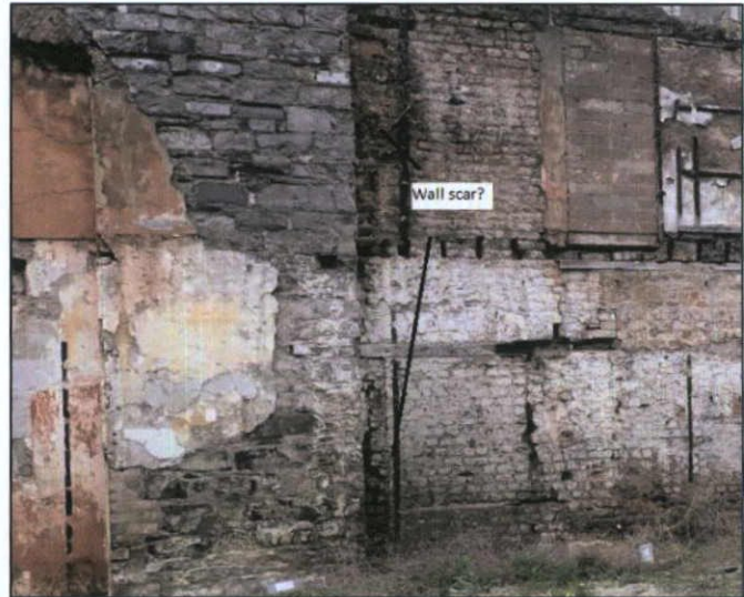
Figure 81 Wall scar of Building 2
