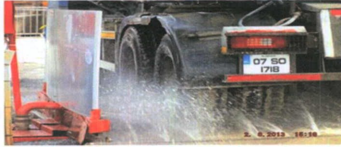
Figure 31. - Typical Wheel Washing Facility
