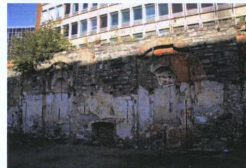
Niches within northern boundary wall, at No.50, suggestive of an 18 th century room of significance
