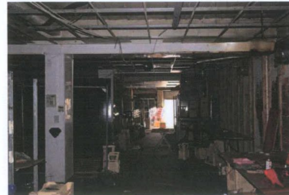
Majority of interior has been stripped of original features
