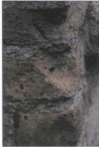
P 13 Possible bullet damage at rear of 57 O'Connell Street Upper
