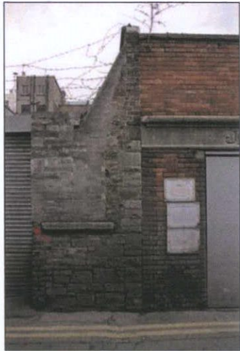
P 12 Evidence of possible bullet damage at rear of 57 O'Connell Street Upper
