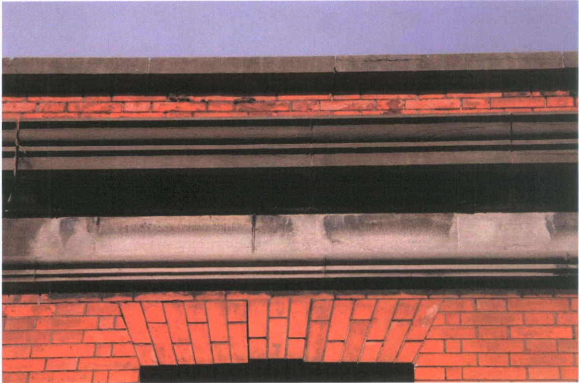
Fig.4.7.3: Detail showing the soiled limestone frieze and coping stones.
