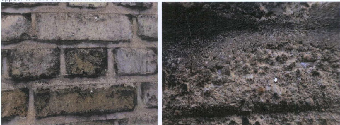
Fig.4.3.5: The rear elevation shows soiled Portland Cement pointing mortar.
