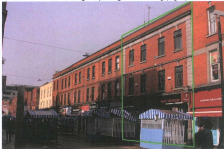
Fig.4.6.2: 1-2 Moore Street. The brickwork is remarkably free from soiling, indicating that it has been cleaned in the relatively recent past.
