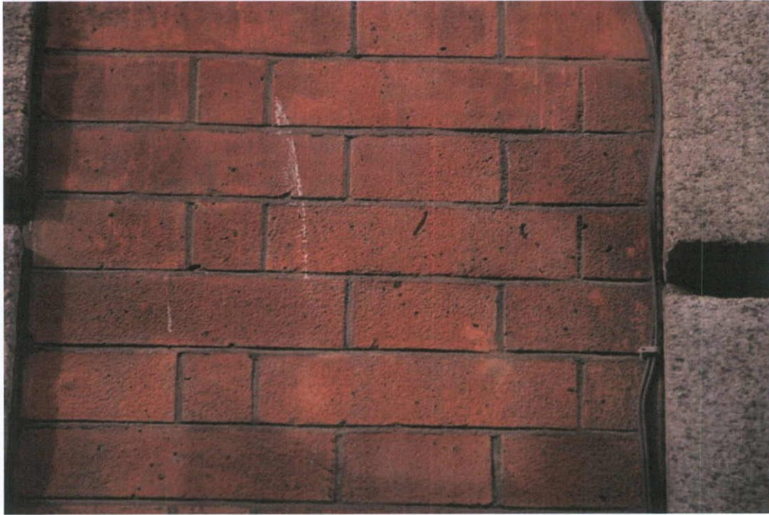
Fig.4.3.3: Detail of the brickwork on the façade of 39 Henry Street showing a damaged surface (probably from past cleaning) and the edge of the Leinster granite detail.
