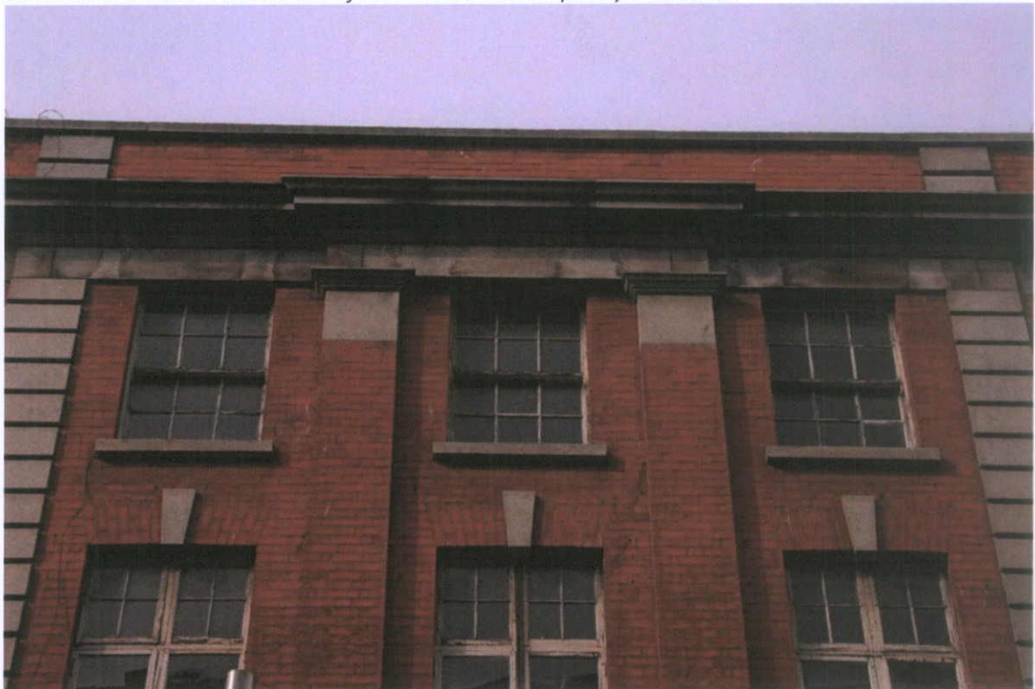
Fig.4.3.2: The superstructure is built with machine-cut red brick with granite used for architectural detailing. The granite shows brown staining, but the building surface is generally free from soiling and has been cleaned in the past.
