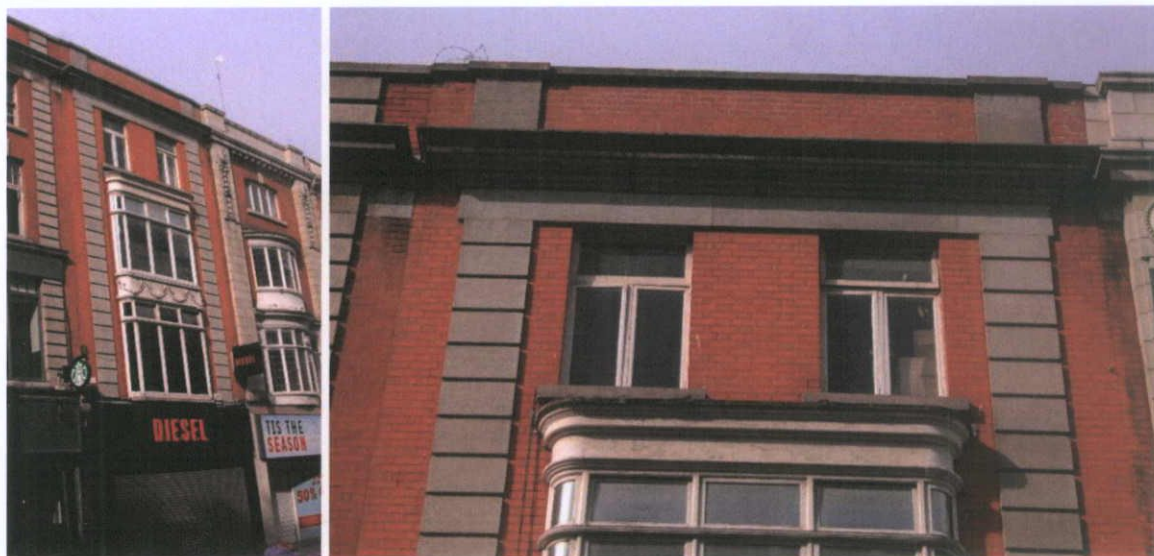
Fig.4.2.1: The façade of 38 Henry Street is of well-fired red brick with limestone detailing, with the parapet rebuilt in a different brick and heavier Portland Cement-based mortar.
