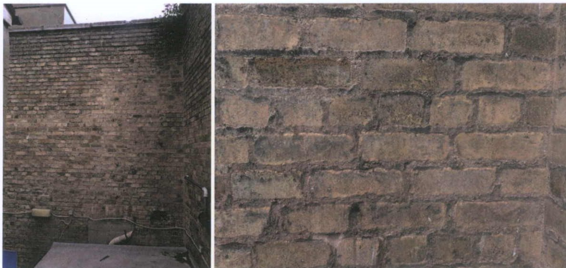
Fig.4.1.1: General view of the brickwork at the rear of 37 Henry Place adjacent to the alley separating Nos.9 and 10 Henry Place.
