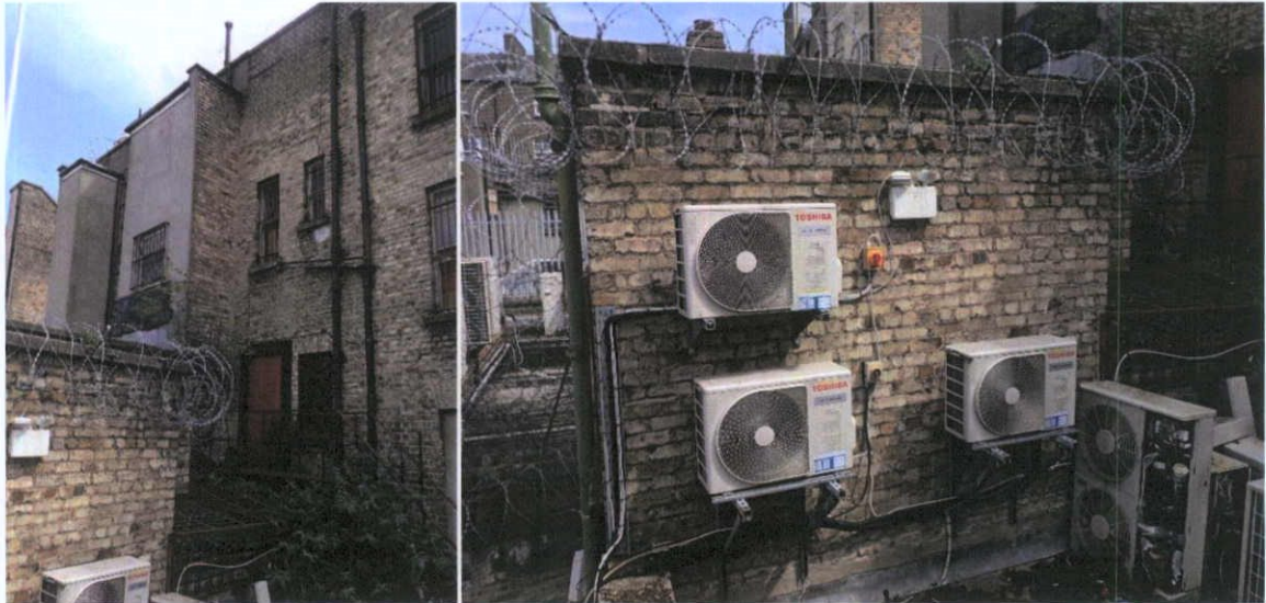
Fig.4.2.4: Yellow stock brick masonry fabric used for the rear and for the return of the building. The same brick is used in the neighbouring rear elevations of Nos.37 and 39 Henry Street, and all three buildings appear to have been erected at the same time.
