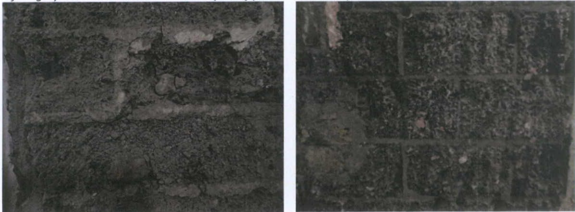
Fig.5.7.5: Concrete blockwork with natural stone, clinker and occasional iron fragments used to form the party wall with No.17 Moore Street, with a similar concrete block of smaller dimension used to form the rear wall of No.18 Moore Street.
