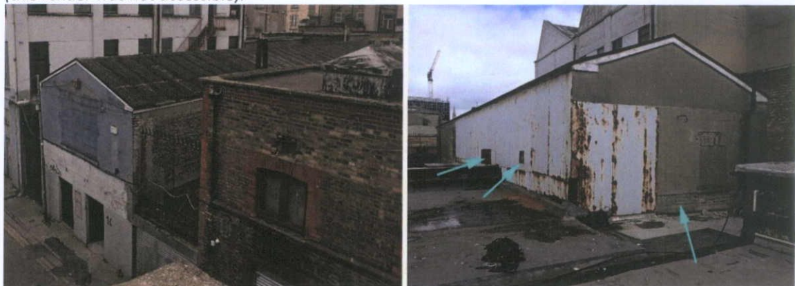
Fig.4.16.2: General view of No.10 Henry Place, with areas of masonry opened up at first floor level on the south and west elevations indicated.
