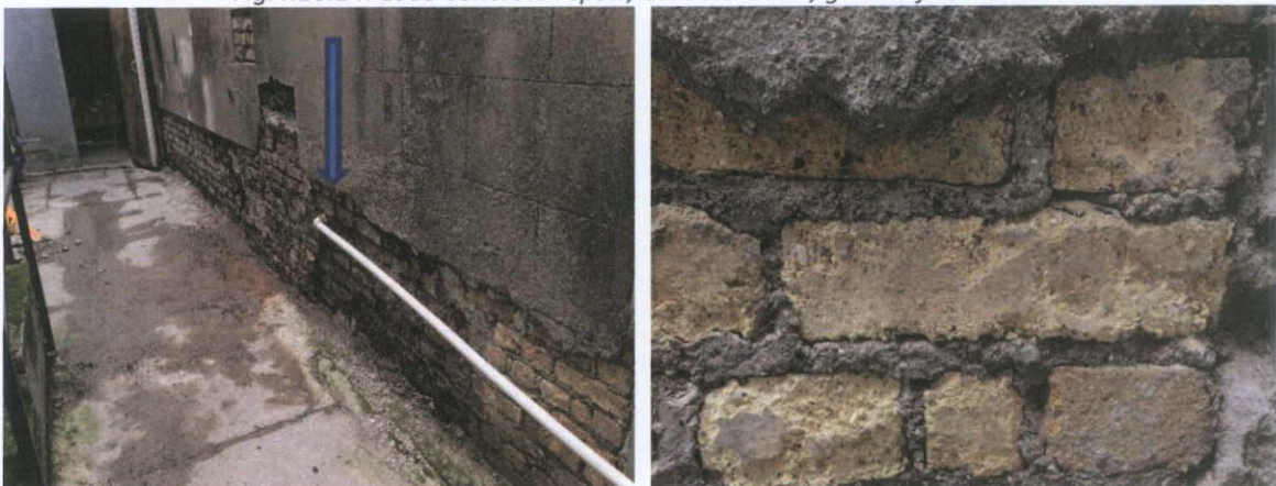
Fig.4.16.15: Junction (arrowed) between the c.1920 yellow stock brick in a cementitious bedding mortar and a section of probably nineteenth century stock brickwork in very poor condition.
