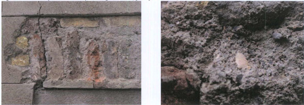
Fig.4.16.5: The first floor window head on the south elevation has a mix of 19 th and c.1920s yellow stock brick (suggesting repair) bedded in a lime-cement mortar with shell included in the aggregate.
