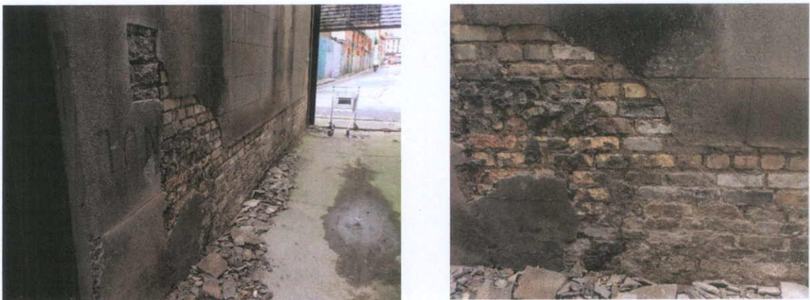
Fig.4.16.9: c.1920 yellow stock brick beneath a Portland Cement render at the north end of the east elevation.
