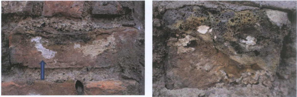
Fig.8.4.12: Poorly-fired place brick in a deep lime-based mortar joint, showing a remnant of a lime-based plaster adhering to part of the surface (left, arrowed). Right: Poorly-fired place brick showing vitrified areas, voids, warping, but with traces of limewash on the surface of the brick.
