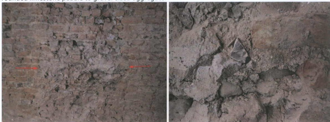
Fig.5.3.7: 'Creephole' at ground floor level, front room, south wall: showing a change in construction with the insertion of broken cobbles and other materials bonded in a cement-based mortar.
