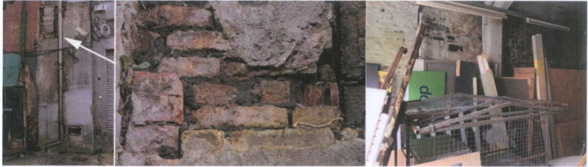
Fig.4.15.3: Exposed wall end at the junction of 5-8 and 9 Henry Place shows a mix of bricks in Portland Cement bedding mortars; internally, the limewash east wall at ground floor level is Calp limestone masonry, and consistent with 19 th century work.
