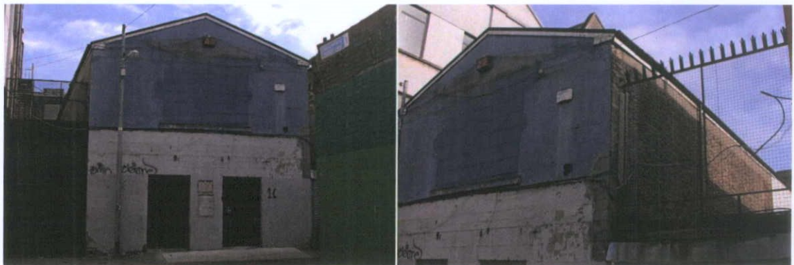
Fig.4.16.1: View of the north façade of 10 Henry Place, and the rendered first floor of the west elevation (this render was not accessible).
