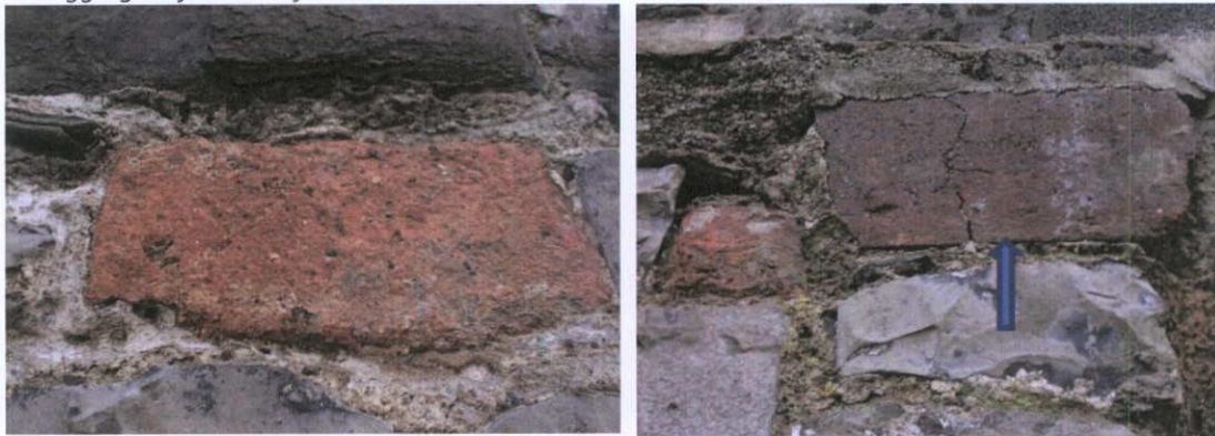
Fig.8.4.9: Warped hand-made clamp fired brick (left) while the upper course contain occasional imported brick (right, arrowed) presumably added as a levelling-up course before the concrete was poured).
