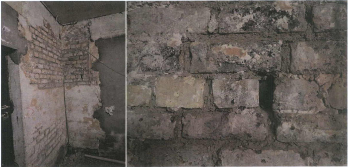
Fig.4.16.7: The north-east corner of the building formed of c.1920s yellow stock brick in a cementitious bedding mortar. There was no trace of any earlier brickwork in this part of the building.
