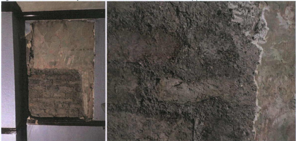
Fig.4.12.3: Yellow and red stock brick bedded in thick lime bedding mortars on the internal face of the north wall of No.9 Henry Street.
