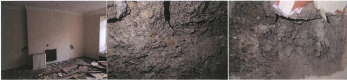
Fig.6.1.3: The south wall of the building (party wall with No.19 Moore Street) is of concrete construction.
