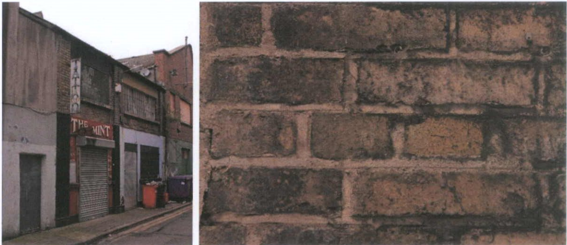
Fig.4.13.1: General view of No.4 Henry Place with a detail of soiled yellow stock brick at first floor level with crudely lined pointing.
