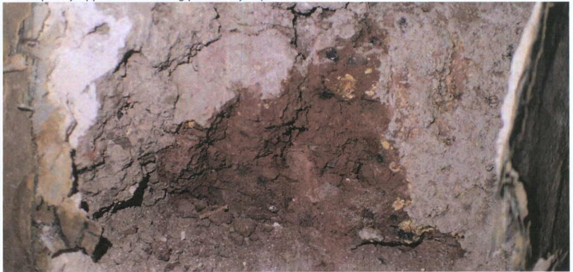
Fig.4.12.7: Hand-made clamp-fired brick with angular limestone aggregate similar to that seen at No.42 O'Connell Street and other Georgian buildings in the area. This type of brick may have been fired at the Moore Street brickfield.
