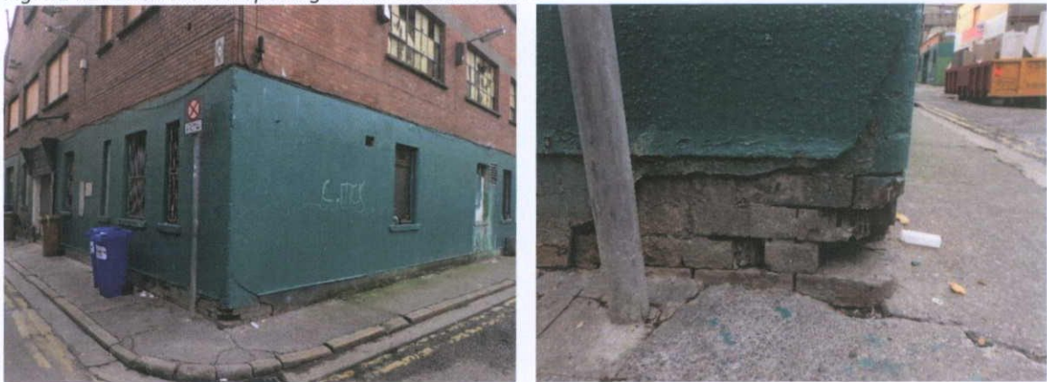
Fig.4.14.3: Render coating the nineteenth century brickwork at ground floor level, with twentieth century brickwork above (left), with extruded perforated brick with rounded edges at the corner (right).
