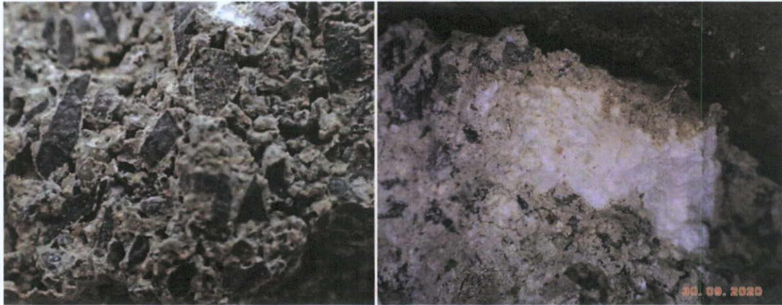
Fig.5.3.10: Detail of 20 th century concrete repair to the south wall at ground floor level.
