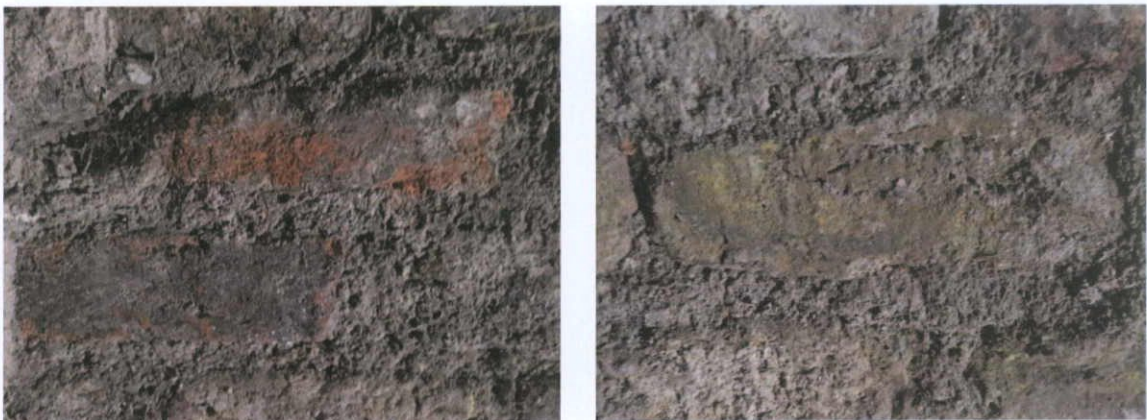
Fig.4.12.5: Red and yellow stock brick, internal wall lining, north wall, 9 Henry Place.
