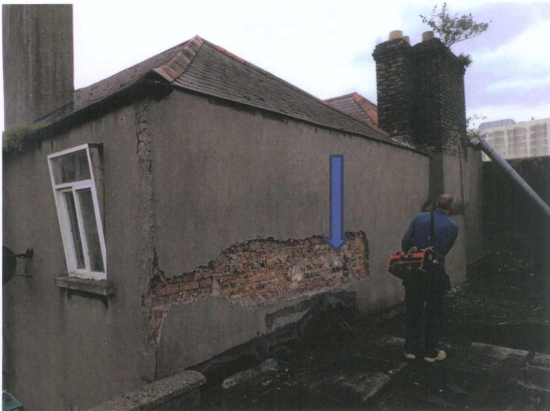
Fig.5.1.6: Exposed brickwork beneath Portland Cement render, north elevation, 10 Moore Street. The masonry has been disturbed and appears to be a 'creep hole' (arrowed). See Fig.5.1.9 also.
