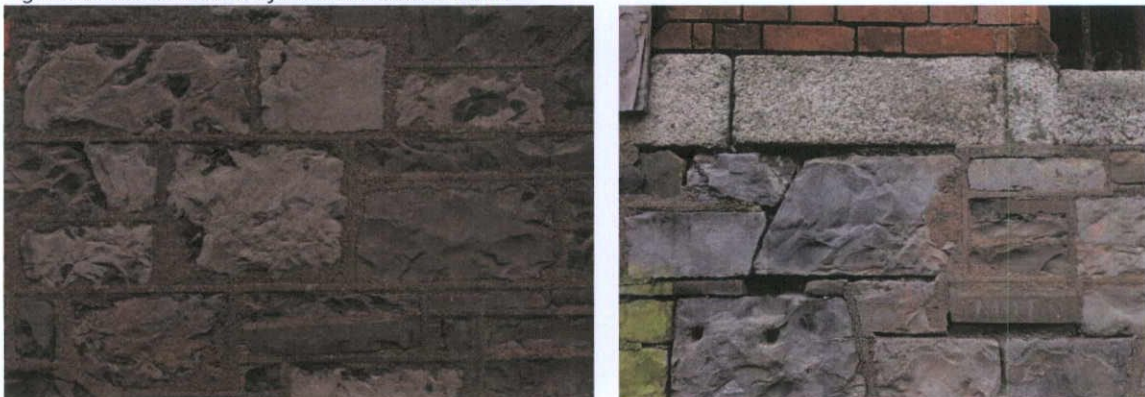
Fig.5.5.2: The coursed hewn Calp limestone masonry has been repointed with coarse-grained Portland Cement strapwork, which was also used as a repair mortar at the time of application.
