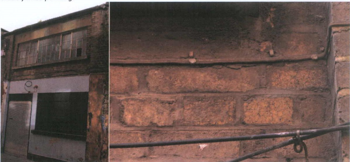
Fig.4.13.2: The brick is pointed in lined Portland Cement-based mortar, and the buff-coloured brick has crazele (network of minor cracks also called crack networks, termed 'crazing' for terracotta).
