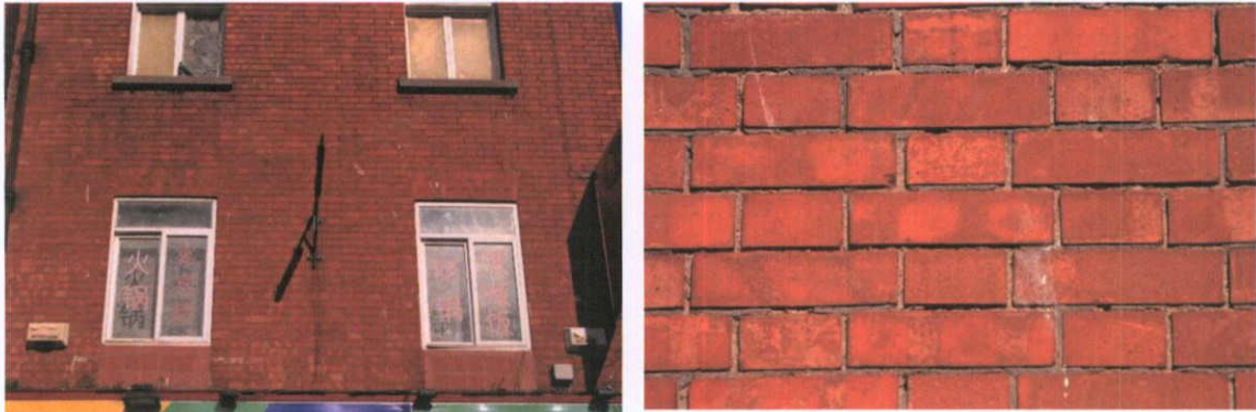
Fig.5.1.2: The façade is of machine-cut fired clay brick, and was not closely examined.
