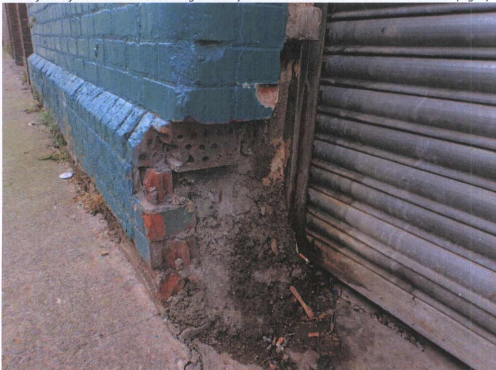
Fig.5.6.9: The south wall is of extruded brick and terracotta with yellow stock brick as internal wall linings, and is probably late nineteenth century construction work.
