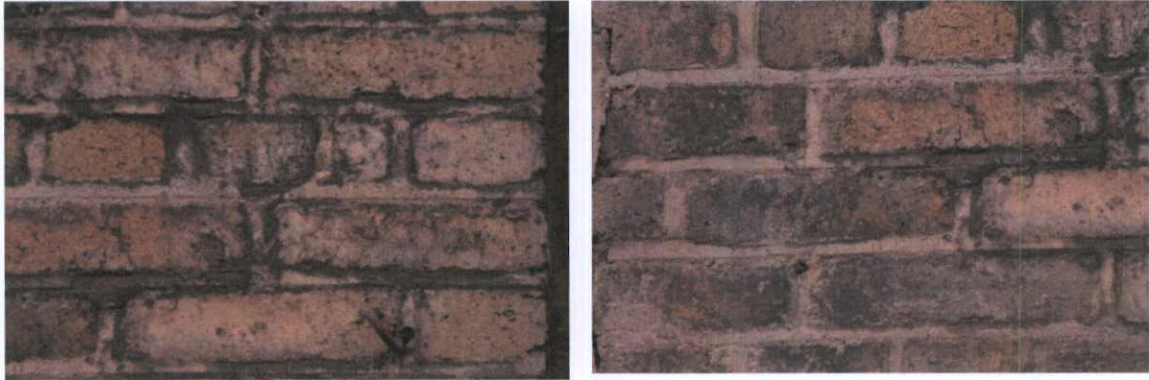
Fig.4.13.3: Soiled buff-coloured brick in lined flush pointing.
