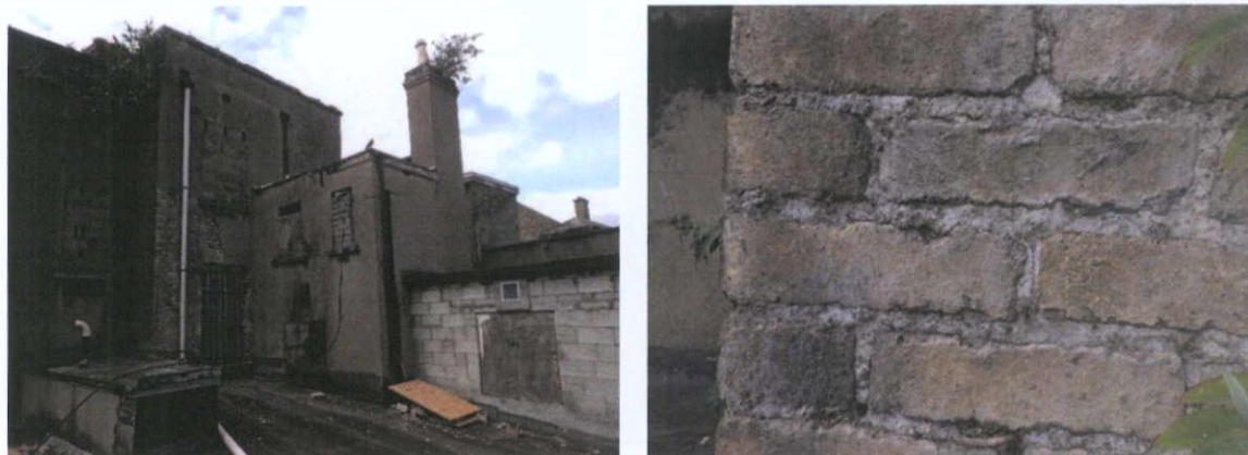
Fig.4.11.3: General view of the rear of No.7 Moore Street, which extends further than the terrace immediately to the south, and was constructed using a yellow stock brick (normally concealed beneath a Portland Cement render).
