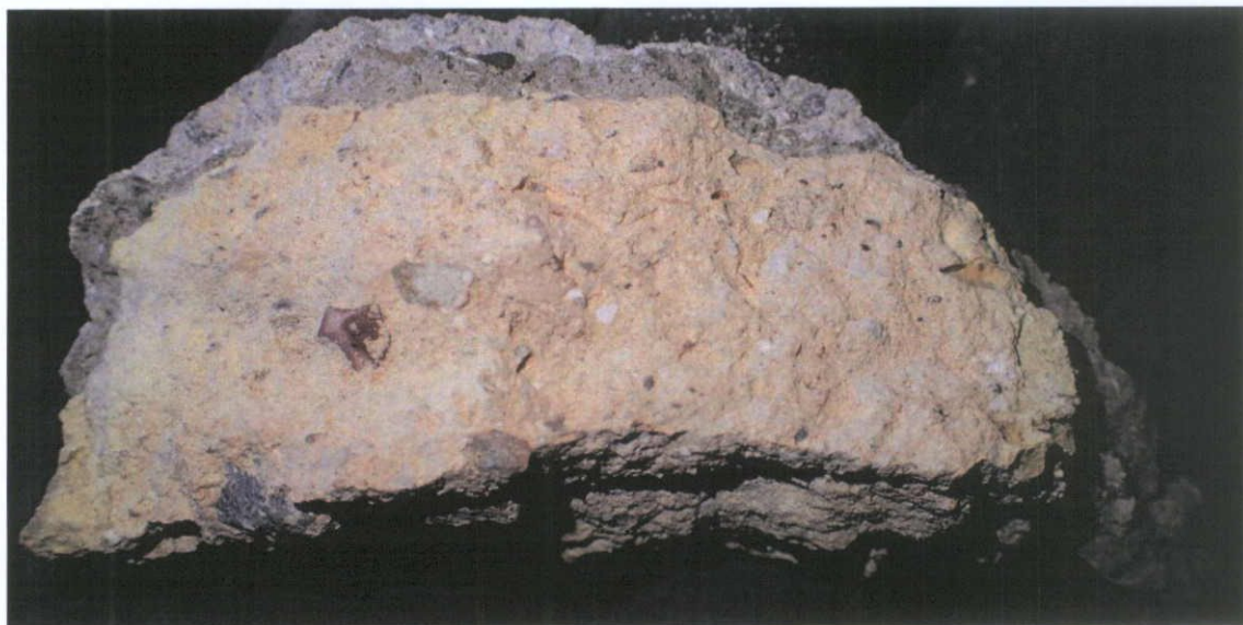
Fig.5.2.12: Yellow 1920s yellow stock brick in grey cementitious bedding mortar.
