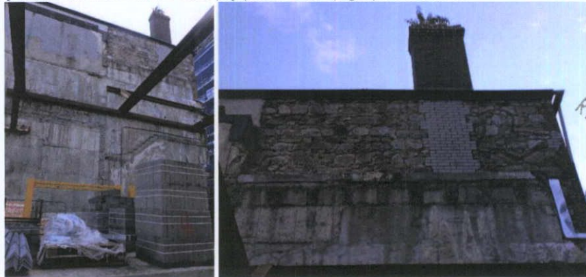
Fig.4.2.3: Reinforced concrete on the south side, with historic masonry of the adjacent property visible at the south-west corner of the site.
