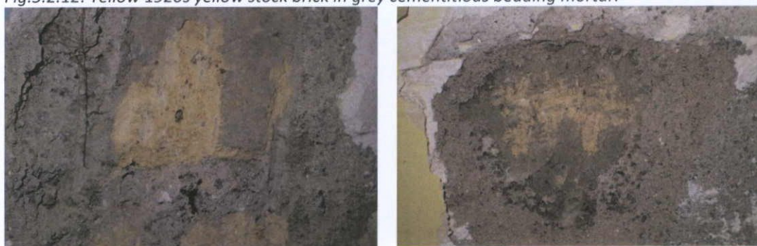
Fig.5.2.13: 1920s yellow stock brick in cementitious mortar exposed in the party walls of the north (left) and east (façade) walls of the first floor level.
