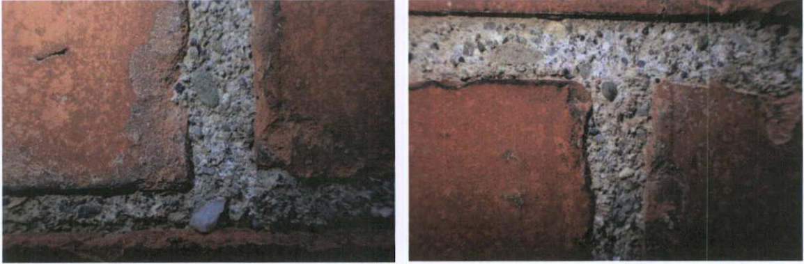
Fig.5.1.4: Detail of aggregate-rich matrix, very different in composition, texture and character to Georgian and Victorian mortars. Brick pozzolan has been added to the bedding mortar.
