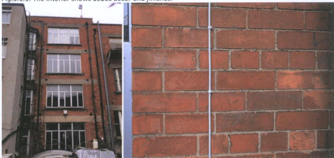
Fig.5.1.2: The rear is composed of machine-cut red brick laid in English garden bond with a lime-cement mortar and having concrete courses above the window openings.
