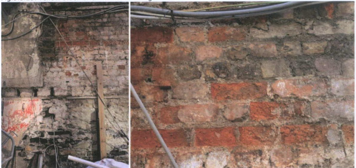
Fig.5.3.26: The red stock brick, in poor condition with the fireskin lost in many places, and the lower section of Calp limestone masonry also visible (left, bottom).
