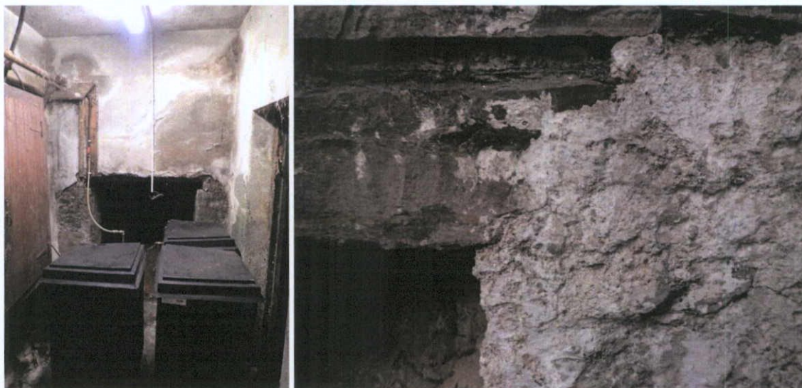
Fig.5.4.8: Calp limestone masonry at basement level at the front of No.57 O'Connell Street.
