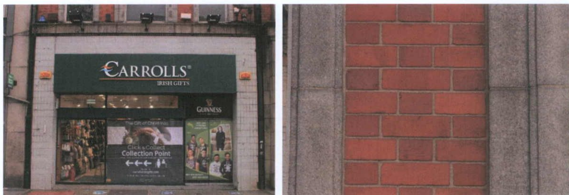
Fig.5.5.2: Modern shopfront with earlier granite course above (left); and a detail showing kiln-fired c.1920s brick in flush mortar joints (right).
