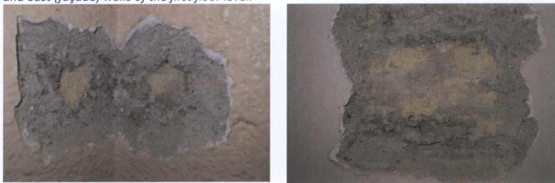
Fig.5.2.14: 1920s yellow stock brick in cementitious mortar exposed in the party walls of the south (left) and west (rear) walls of the first floor level.
