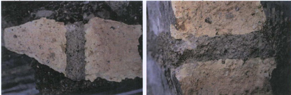
Fig.5.2.8: Cross section showing the 1920s brick with natural stone inclusions in an evenly-fire matrix and bonded with a cementitious bedding mortar. Sample #90.
