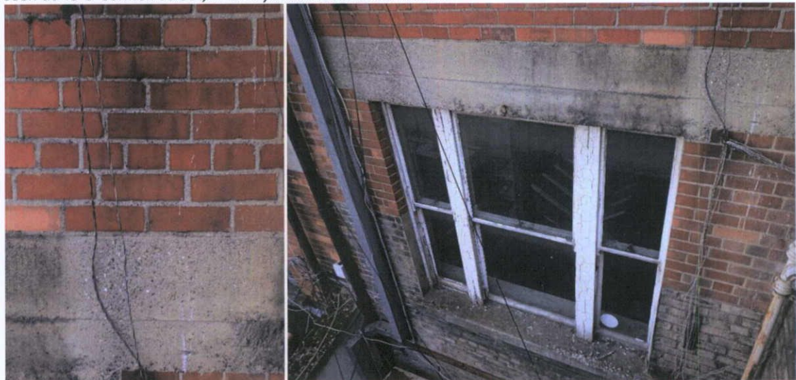
Fig.5.2.2: Detail of the 1920s machine-cut brick and concrete lintel of the superstructure, above yellow stock brick at the rear basement level.
