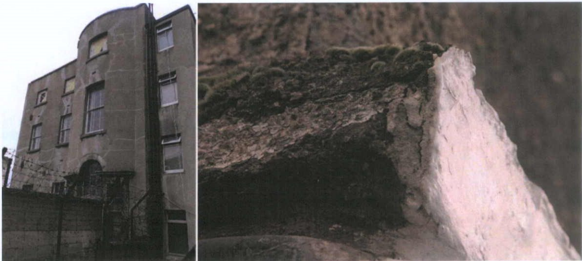
Fig.4.3.13: The rear retains a tripartite arched window in the curving bay, mirroring the treatment of the main door. The rear has been re-rendered throughout in a Portland Cement-based mortar.
