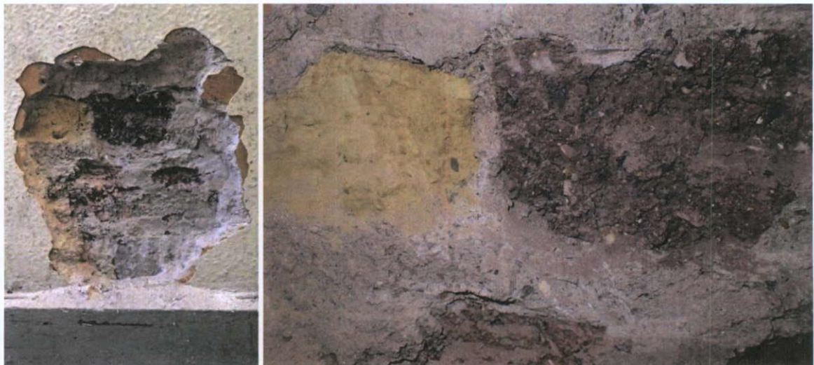
Fig.5.2.17: Ground floor, south wall, interior showing 1920s yellow stock brick and dark-red hand-made clamp-fired brick above skirting level, both bedded in a cementitious bedding mortar. The red brick appears to be a Georgian period brick, similar to others seen along the west side of O'Connell Street and possibly an example of a brick from the Moore Street brickfield. This appears to be a salvaged brick, reused in the masonry of the 1920s construction work.
