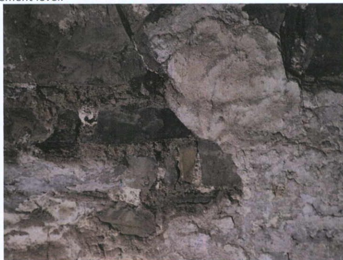
Fig.5.2.3: Dublin Calp limestone at basement level with single-coat lime plaster and multiple coats of limewash.
