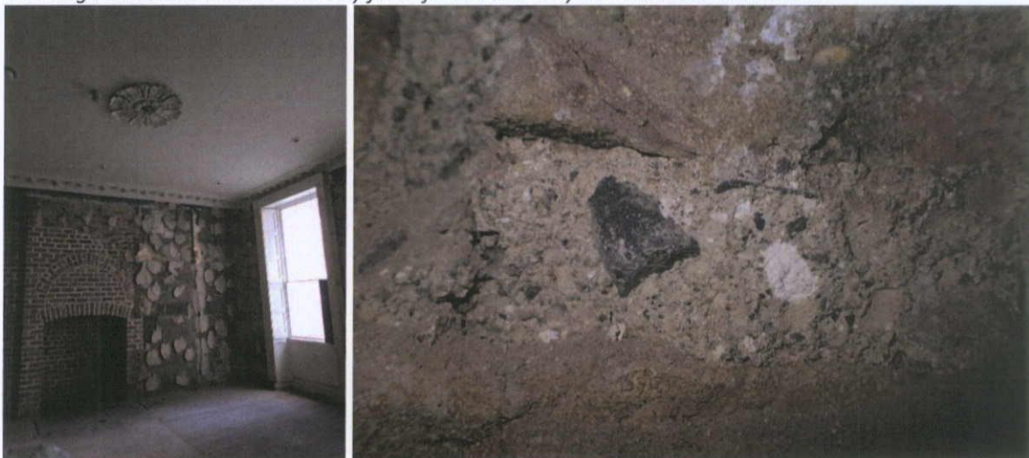
Fig.4.3.6: The ground floor shows later alterations, but the party wall shows place brick laid in a coarse-grained lime bedding mortar with poorly sorted limestone, quartz and chert aggregate and large lime lumps.
