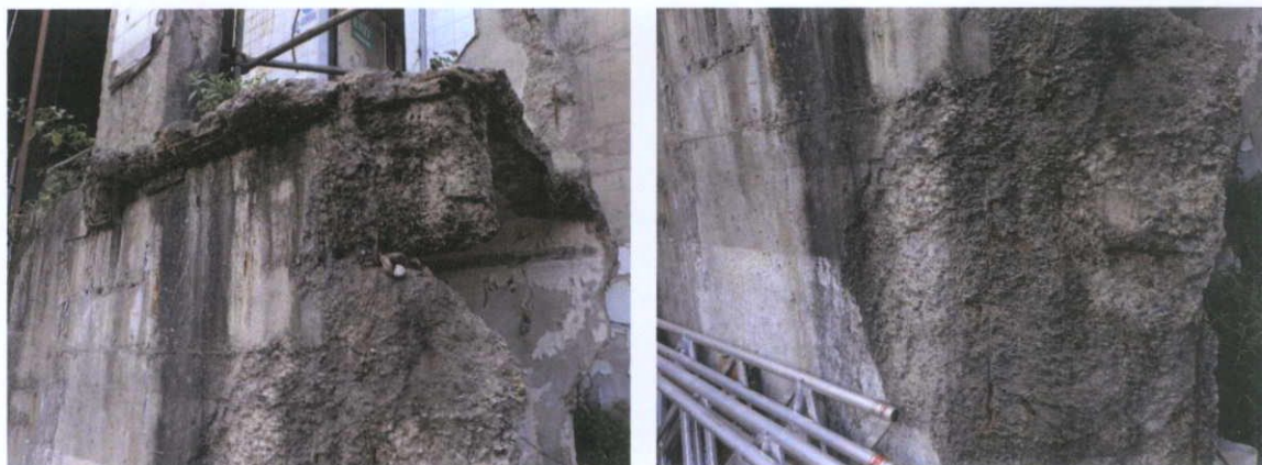
Fig.4.2.5: Detail of reinforced concrete structure on the north side of the site.
