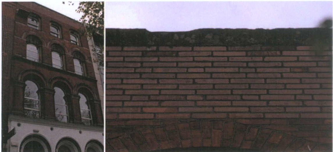
Fig.5.7.1: Façade of 60 O'Connell Street with a detail showing the more recent mid-to late twentieth century brick at parapet level; with repointed nineteenth century brickwork seen below.
