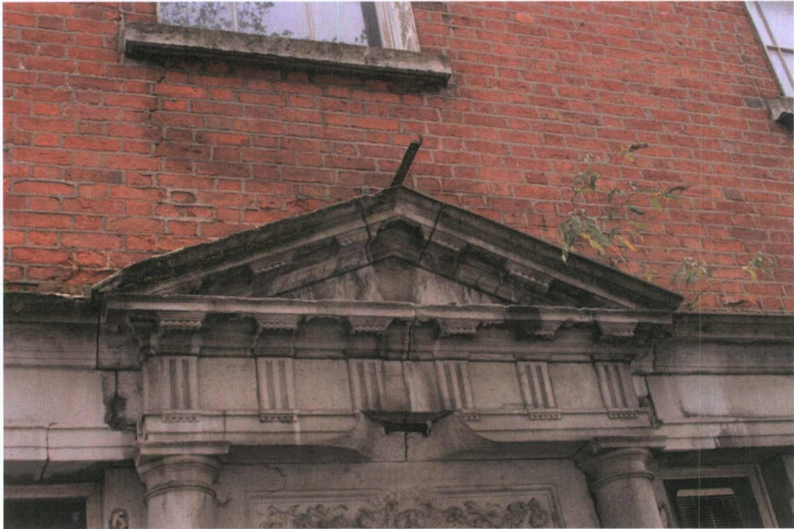
Fig.4.3.2: The red facing brick is laid in Flemish bond and has been repointed throughout in a Portland Cement-based mortar. The repointing is failing (losing bond) in areas of saturation, and loss of the surface of the brick is evidence in many areas.
