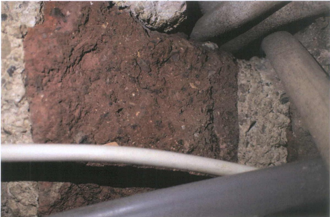
Fig.5.1.9: Detail of a clamp-fired brick seen at basement level showing limestone inclusions.
