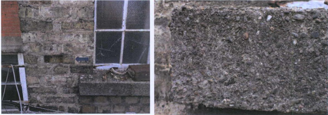
Fig.5.2.7: The window cills are of concrete. The 1920s yellow stock brick also includes occasional earlier clamp-fired yellow stock brick (arrowed), likely to be an example of salvage.
