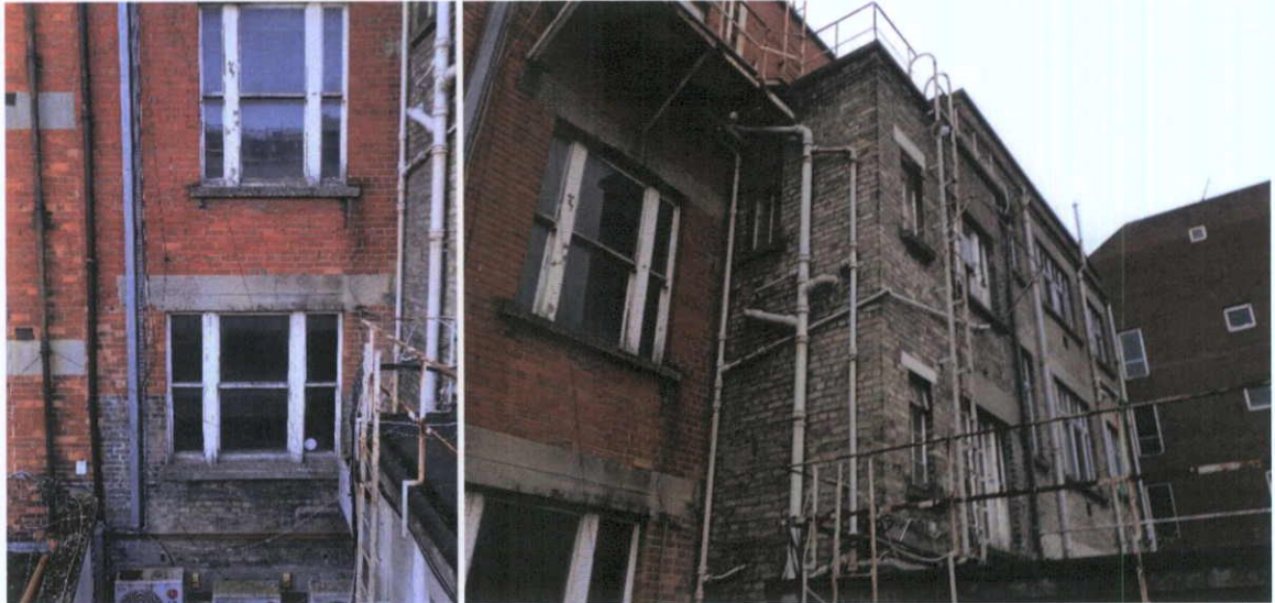
Fig.5.2.1: The rear of 44 O'Connell Street consists of 1920s red brick with concrete lintels similar to that seen at 43 O'Connell Street, with a yellow stock brick return.
