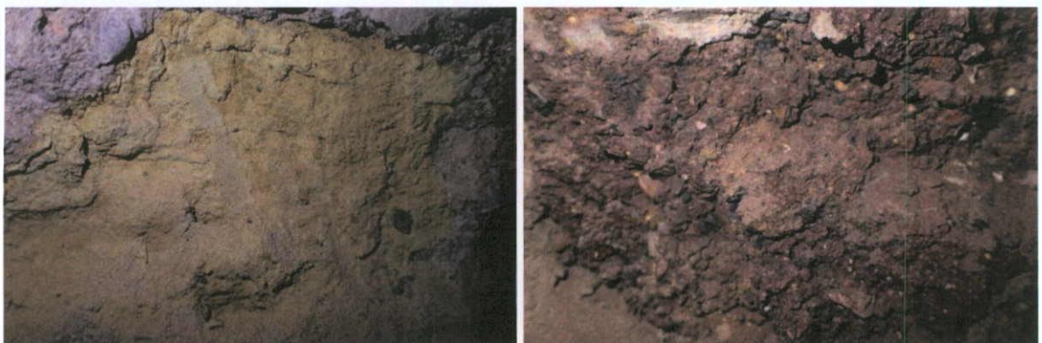
Fig.5.2.18: Detail of the fine-grained yellow stock brick from the 1920s (left) and the dark-red clamp-fired Georgian brick which contains abundant natural stone inclusions, partially calcined limestone and burnt 'hot spots' suspended in the matrix.
