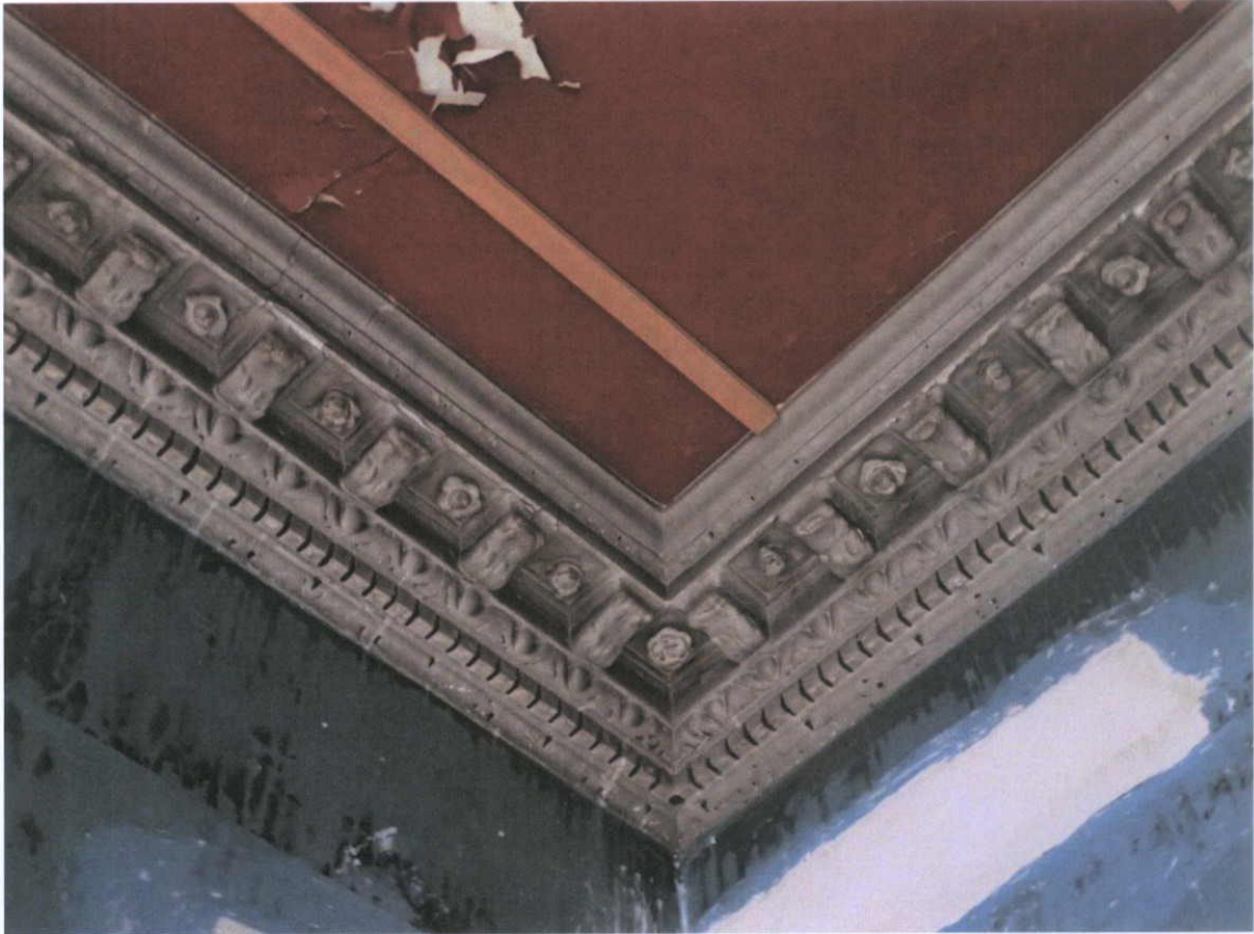
Fig.4.3.12: Detail of the ceiling at the head of the staircase showing three different materials: a) Flatwork ceiling plaster (probably haired lime with additions) b) Ornate cornice probably built out from timber or brick base c) Flatwork wall plaster (probably not haired, but likely to contain brick pozzolan).
