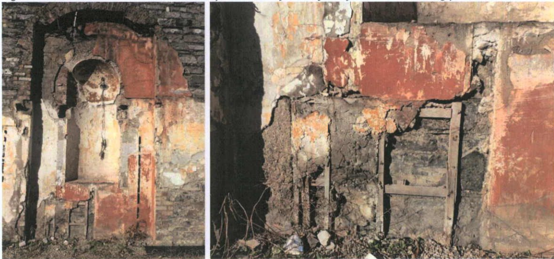
Fig.5.3.11: The eastern arch has gypsum plaster on a modern keyed and netted plaster.
