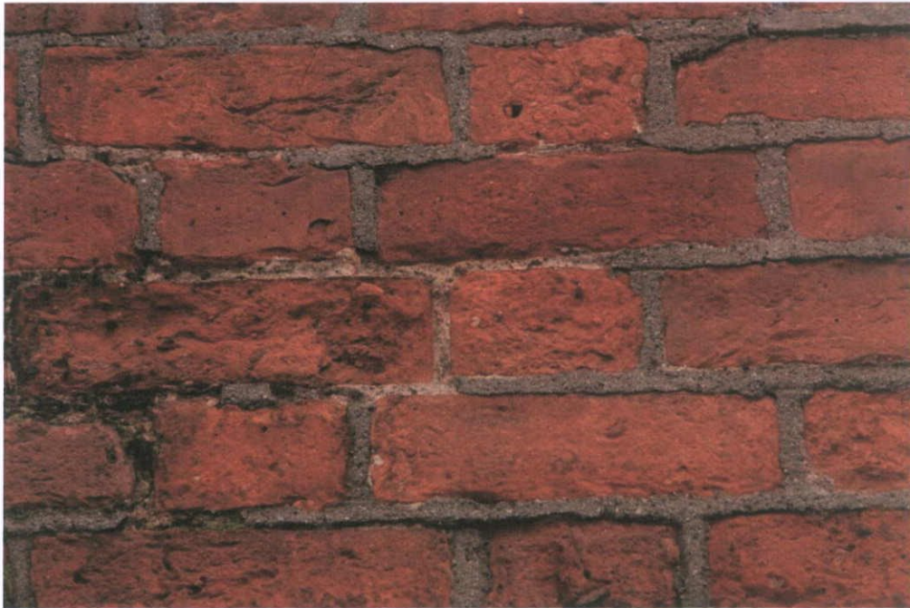
Fig.4.3.4: The façade brick is handmade and contains abundant inclusions of pebbles and fired material. The lime bedding mortar contains relatively coarse aggregate (up to ½ the joint height).
