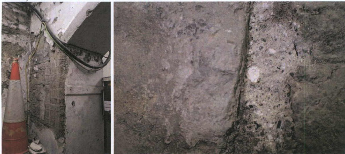
Fig.5.7.4: Detail of a mid-nineteenth century brick arch at basement level of No.60, with sharp limestone sand and coarse lime lumps in the bedding mortar (beneath the Portland Cement pointing).
