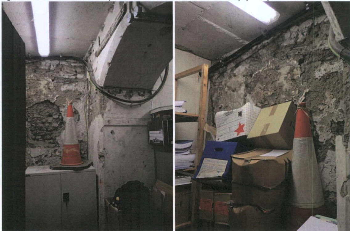
Fig.5.7.3: View of a brick pier at the front of the property at basement level, with a rendered Calp limestone masonry wall.
