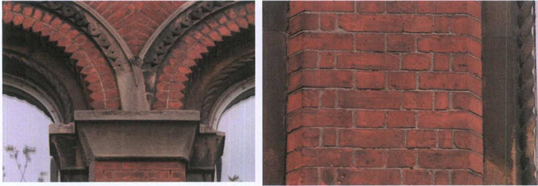
Fig.5.7.2: Mid-nineteenth century Victorian brick and stonework on the façade of 60 O’Connell Street.
