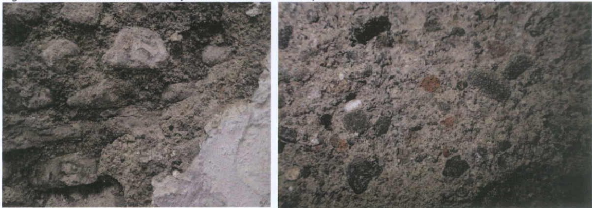
Fig.5.7.6: The south wall of the basement well is formed from Calp limestone masonry, many of which consist of rounded and sub-rounded cobbles which are indicative of Georgian building. The lime render laid on top of the wall is in poor condition; but contains poorly-sorted predominantly limestone aggregate with large coarse lime lumps and crushed brick and brick dust pozzolan.
