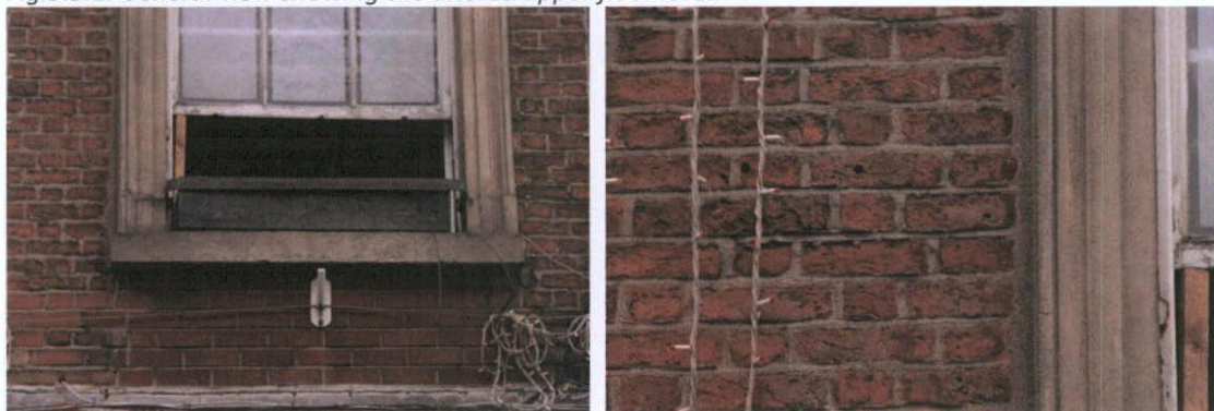
Fig.5.9.2: Modern brickwork below the window cill, and original brick repointed in Portland Cement.
