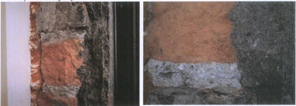
Fig.5.9.5: The rear elevation is coated with multiple layers of Portland Cement render above red stock brick.
