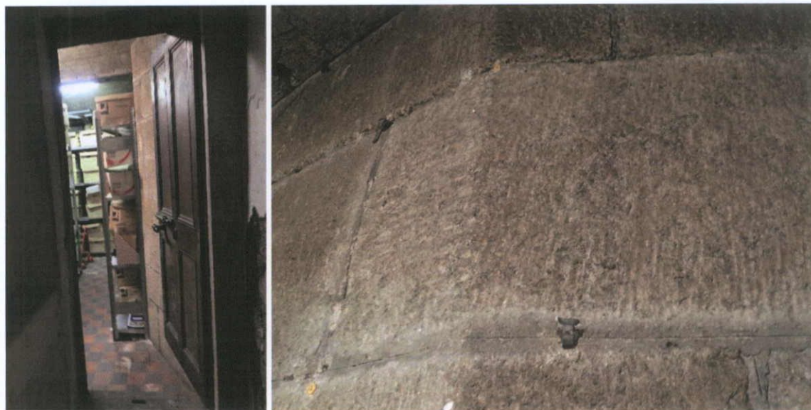
Fig.5.7.10: The strong room is lined with granite laid in a lime putty mortar, and pointed with a Portland Cement-based mortar with an incised line.
